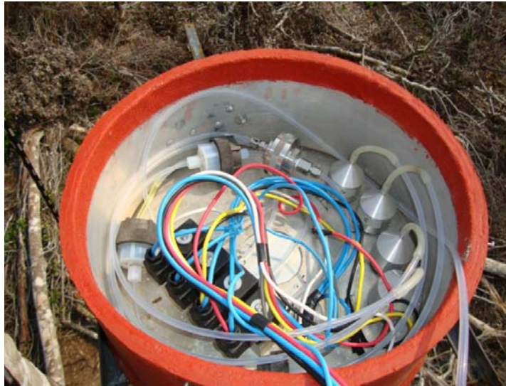
Figure 5 – Shelter Box installed in the top of the tower: manifold, electrovalves, filters, pre-filters for retention of particulate materials.
