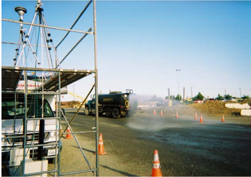
Figure 4. Water Truck at the Bradshaw Plant (Downwind monitoring site shown on left)
