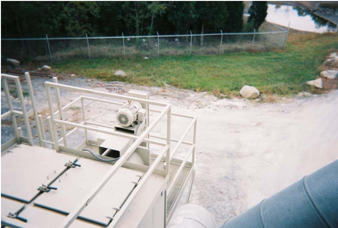
Figure 3-3c. Plant 4 Fabric Filter Outlet Duct Test Location (Stack extension to be built.)
