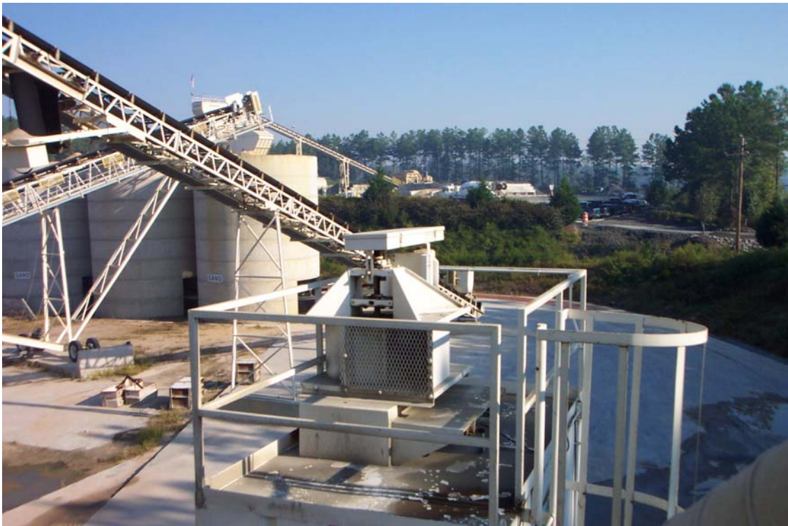
Figure 3-1c. Plant 1 Fabric Filter Outlet Duct Test Location (stack location to be built.)
