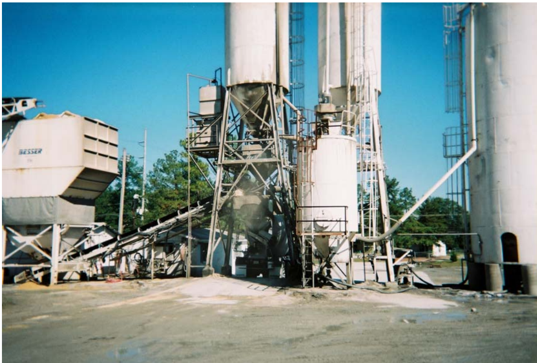
Figure 3-4c. Plant 5 Fabric Filter Outlet Duct Test Location (Stack extension to be built.)
