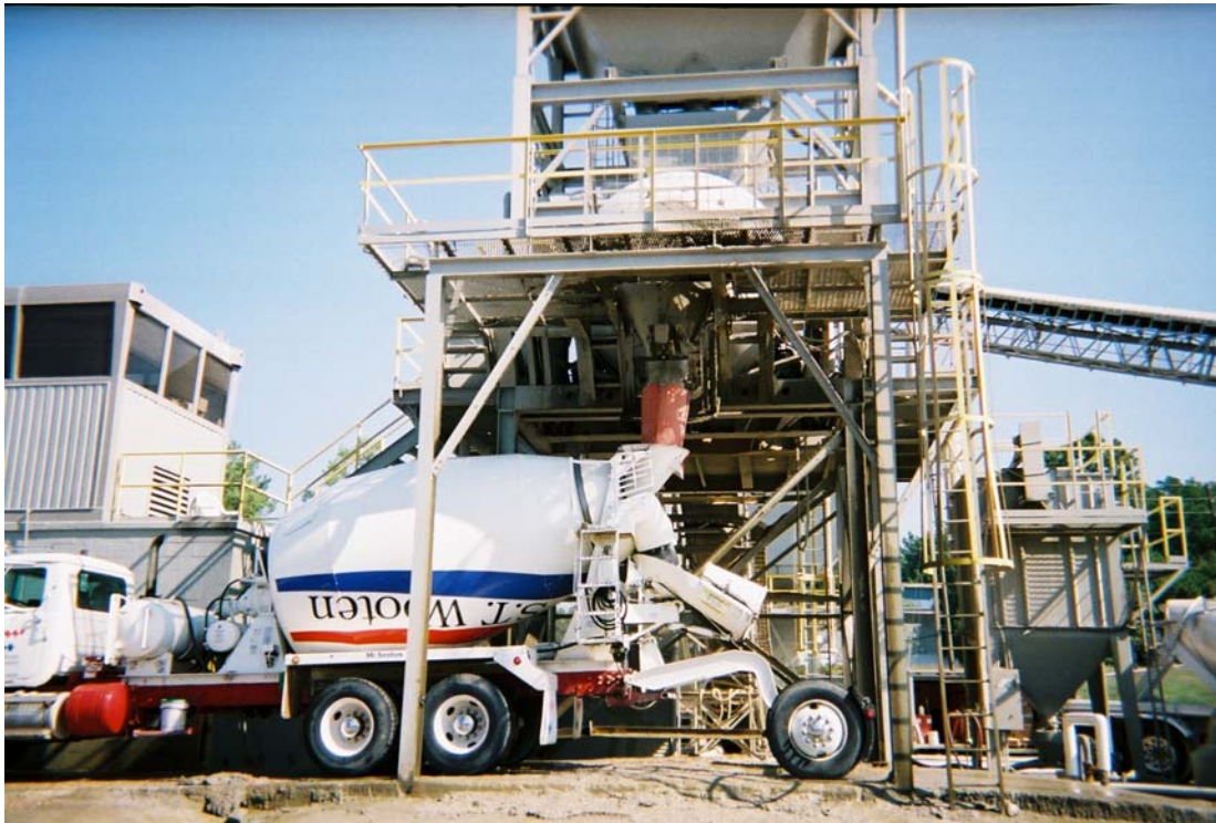
Figure 3-2a. Plant 2 Truck Loading Area
