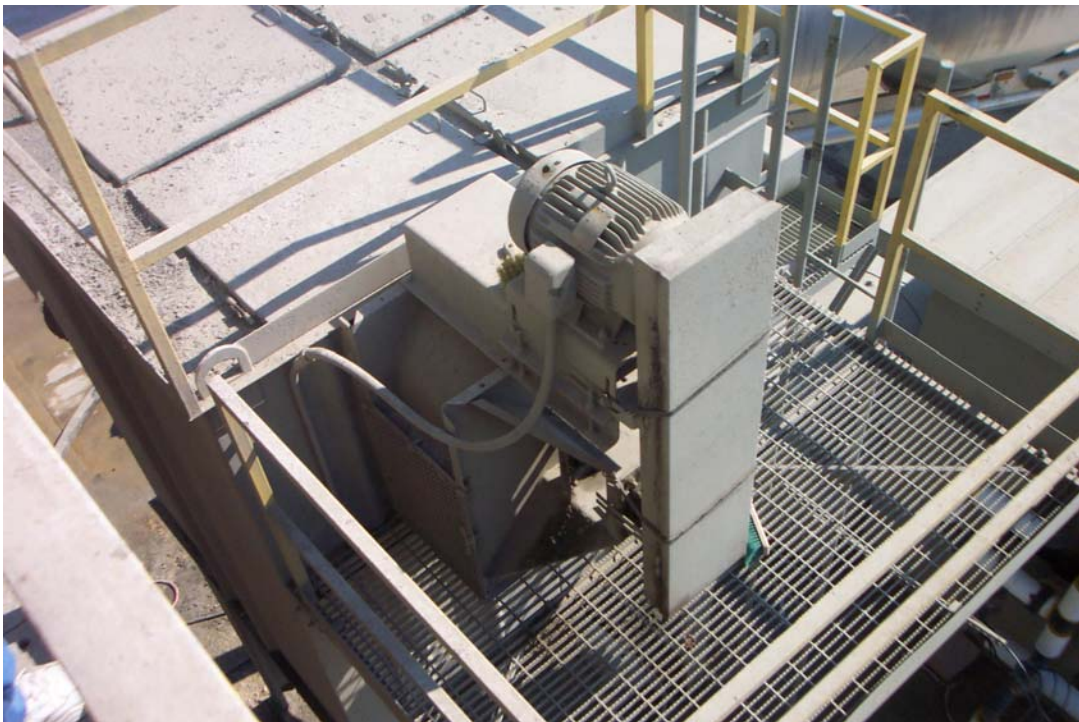
Figure 3-2c. Plant 2 Fabric Filter Outlet Duct Test Location (stack extension to be built.)
