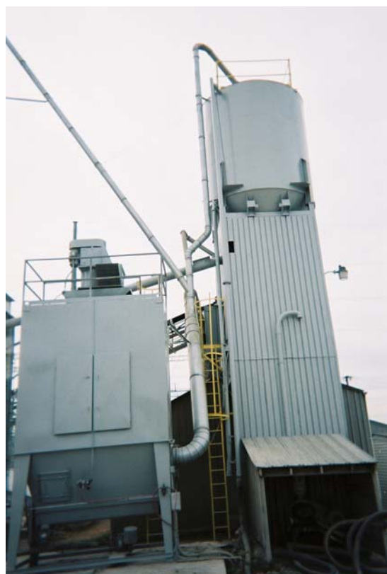
Figure 3-5c. Plant 6 Fabric Filter Outlet Duct Test Location (Stack extension to be built.)
