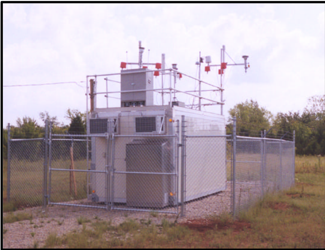
Figure 1. Movable platform deployed at the Park Hills (MO) satellite site.
