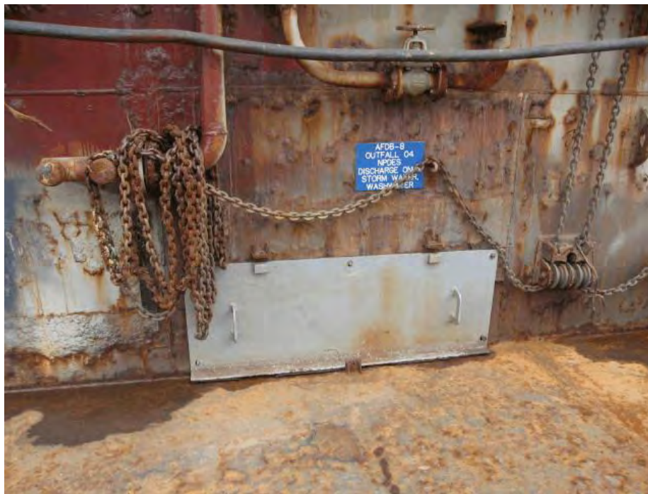
Photo 2 - View of Outfall No. 4 inlet on from inside drydock. Note metal plate used to prevent discharges during normal operations.
