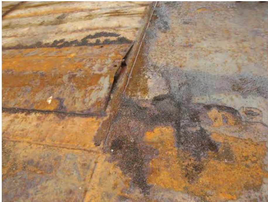
Photo 4 – Accumulated solids on drydock deck
