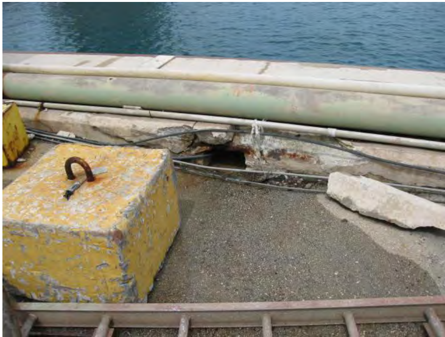
Photo 8 – Evidence of discharge of non-stormwater to harbor from a scupper immediately adjacent to the where a barge was undergoing work onshore.
