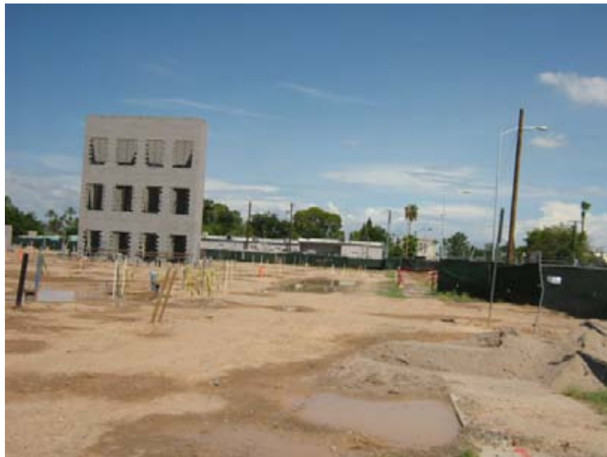
Photograph 14: Mesa Municipal Court General view of southern portion of construction site area looking east
