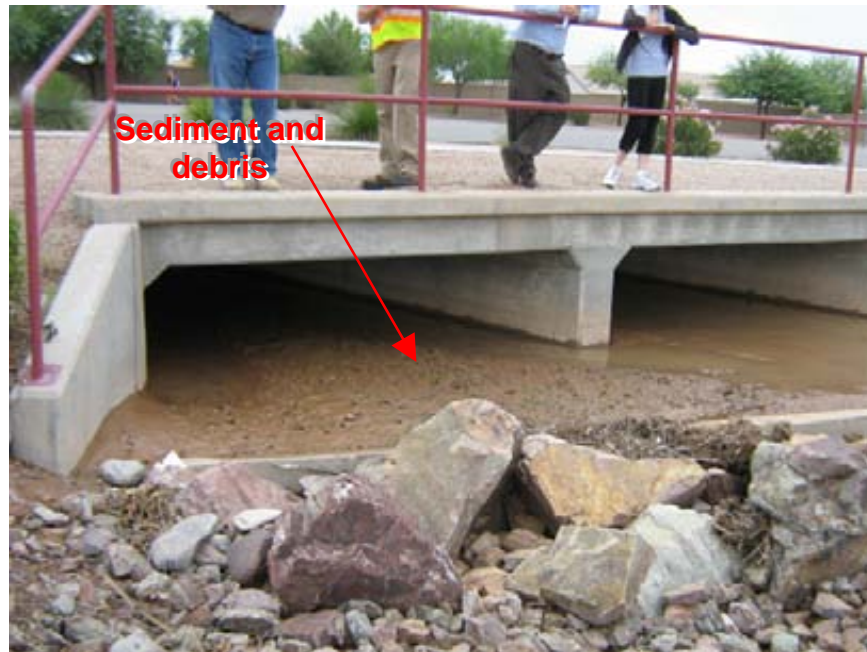
Photograph 7: Mountain View Village Center Sediment and debris were observed in the drainage channel above the flow control structure
