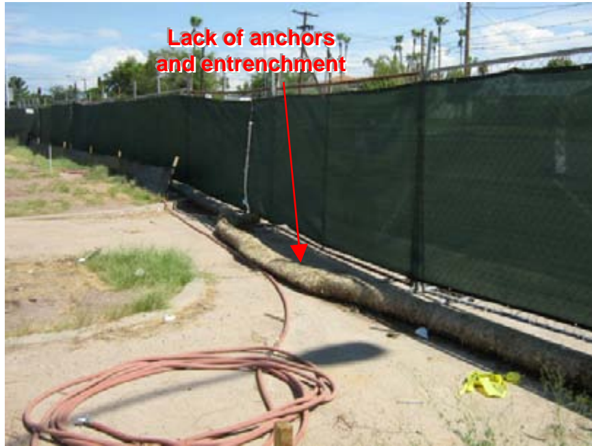
Photograph 15: Mesa Municipal Court Straw wattles were installed on an impervious surface, and therefore were not properly entrenched or anchored to create an adequate seal
