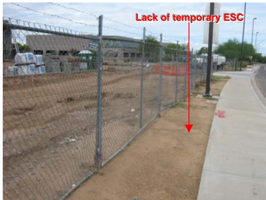
Photograph 12: Superstition Springs Commerce Center BMPs were not implemented as perimeter control along Hampton Avenue, between the disturbed area and the offsite curb and gutter flowline
