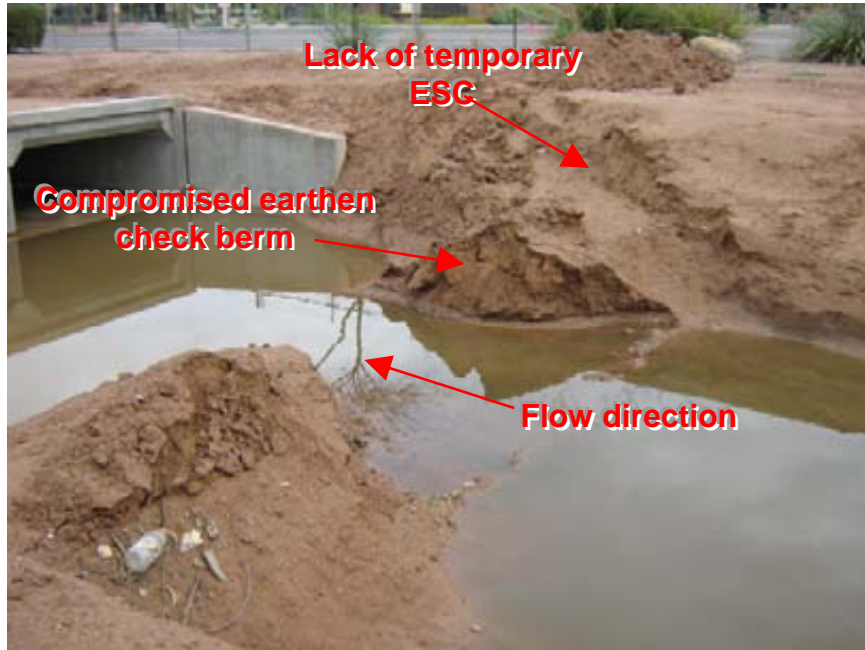
Photograph 3: Mountain View Village Center Earthen check berm consisting of unconsolidated fill had been placed within the drainage channel and was compromised by a recent flow event
