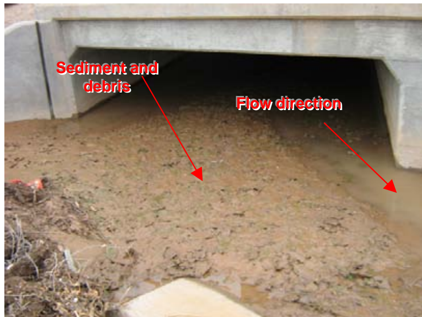
Photograph 8: Mountain View Village Center Close-up view of area shown in Photograph 7 depicting sediment deposition directly downstream of the failed silt fence shown in Photograph 6
