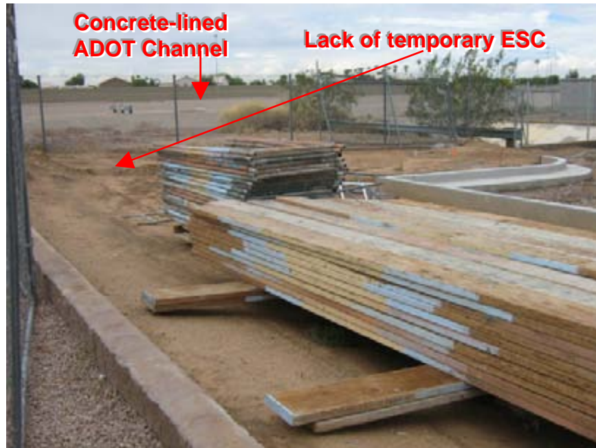
Photograph 11: Superstition Springs Commerce Center View showing proximity of site to the ADOT Channel and lack of BMPs
