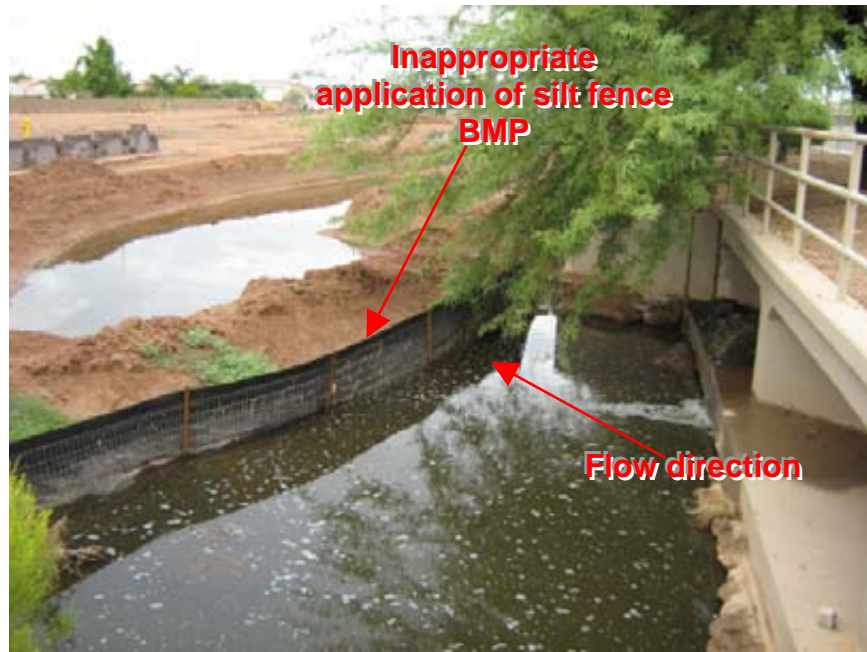
Photograph 1: Mountain View Village Center Drainage channel conveys flow into the northeast side of the site, where a silt fence BMP had been improperly implemented in an area of concentrated flow
