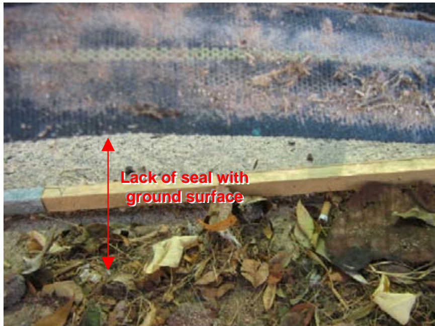
Photograph 16: Mesa Municipal Court Sections of the silt fence along the southern perimeter were not maintained with adequate entrenchment
