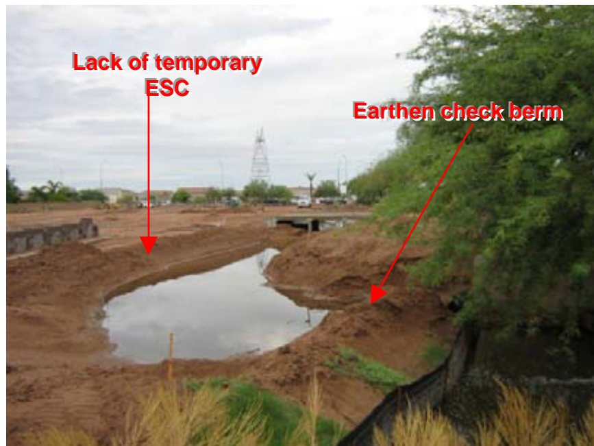
Photograph 2: Mountain View Village Center View of drainage channel leading west across the site and earthen check berms installed along this course
