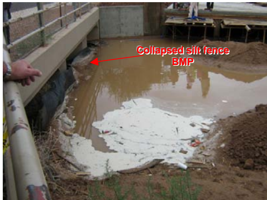
Photograph 6: Mountain View Village Center Collapsed silt fence BMP installed within the concentrated flow of the drainage channel prior to exiting the site
