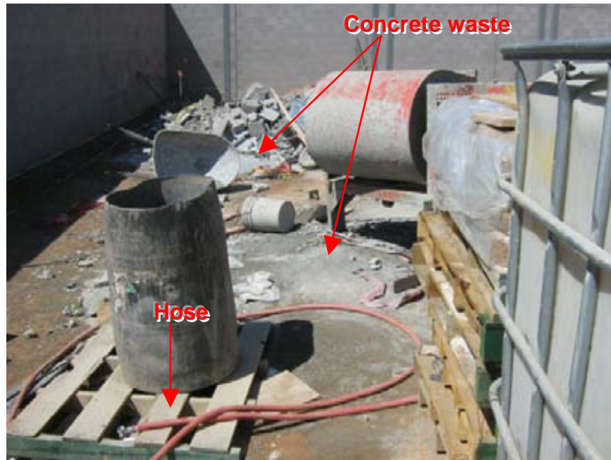
Photograph 17: Mesa Municipal Court Concrete waste and washout hose located near mixer
