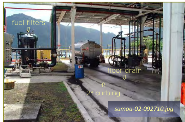
Photo #1-6: Area B - Bottom Fill Loading Rack Taken By: Greg V. Arthur Date: 09/27/10
