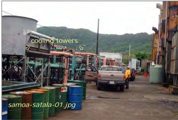
Photo #1: Cooling Towers and Paved Access Areas Taken By: Greg V. Arthur Date: 04/01/08
