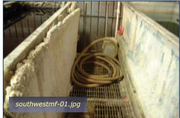
Photo #2: Portable Pump Transfer Hose Taken By: Greg V. Arthur Date: 09/22/09
