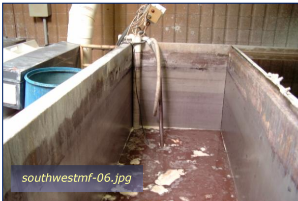
Photo #3: Transfer Holding Tank T5 Taken By: Greg V. Arthur Date: 09/22/09
