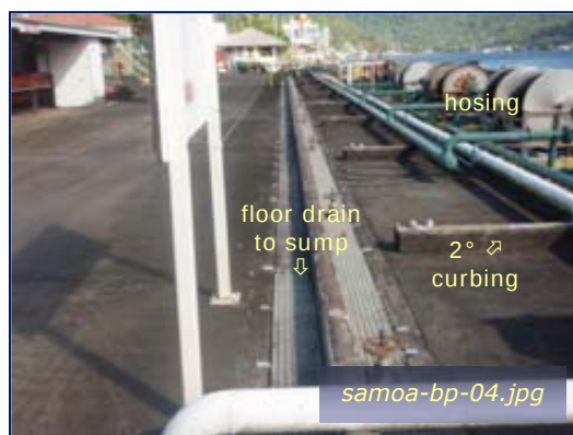
Photo #5: Fueling Dock – looking west Taken By: Nick King, Assistant Terminal Manager Date: 06/22/09
