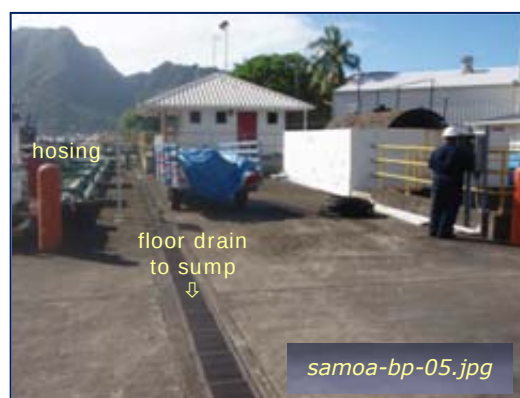
Photo #6: Fueling Dock – looking east Taken By: Nick King, Assistant Terminal Manager Date: 06/22/09
