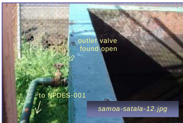
Photo #5: Waste Oil Tanks 2°Containment Taken By: Greg V. Arthur Date: 04/30/09
