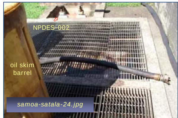
Photo #8: NPDES Sump #2 – Western Oil Water Sep Taken By: Greg V. Arthur Date: 04/30/09
