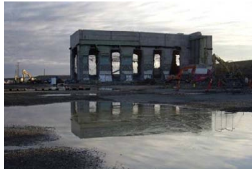
TAN-607 Hot Shop ready for explosives
