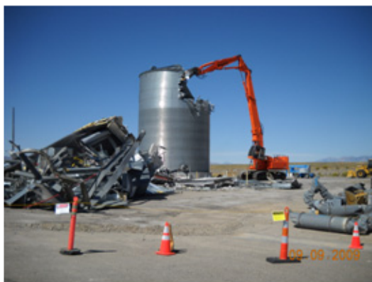
PBF-761, Spray Dryer Absorber
