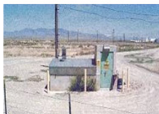
TAN-655, Liquid Waste Lift Station
