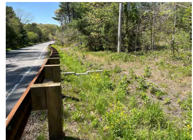
Roadside Swale with Check Dam (Credit: HW)
