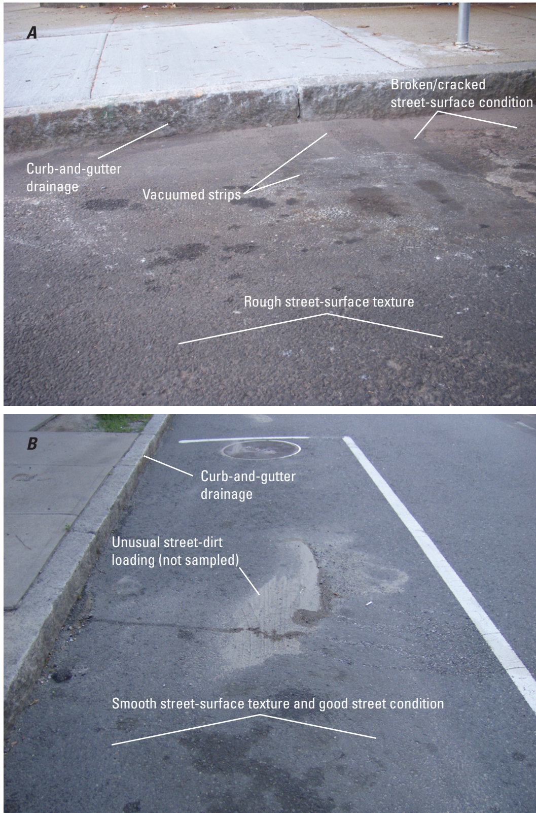
Figure 4. Photograph of A , two cleaned vacuumed paths typical of street-solid composite sampling, and examples of a rough street-surface and a poor street-surface condition (photo courtesy of Tom Maguire, MassDEP), and B , a smooth street surface with good street-surface condition, curb-and-gutter drainage system, and an example of unusual loading avoided during sampling, Cambridge, Massachusetts.
