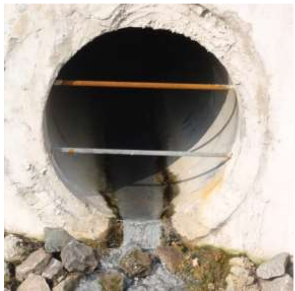
Figure 2. White/gray material seen in the pipes is a bacterial plaque often indicative of sanitary sewage.
