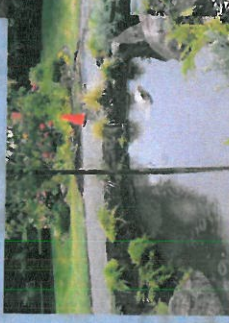
Images of the first rain after the curb cut and installation of the rain garden. Stormwater flowing down Chestnut Street is diverted to the rain garden. Before, stormwater flowed to a nearby catch basin and discharged untreated directly into the Exeter River.
