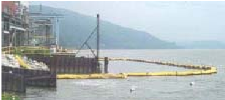
Figure 4.16 Gunderboom® MLEST™ Deployed at Lovett Generating Station
