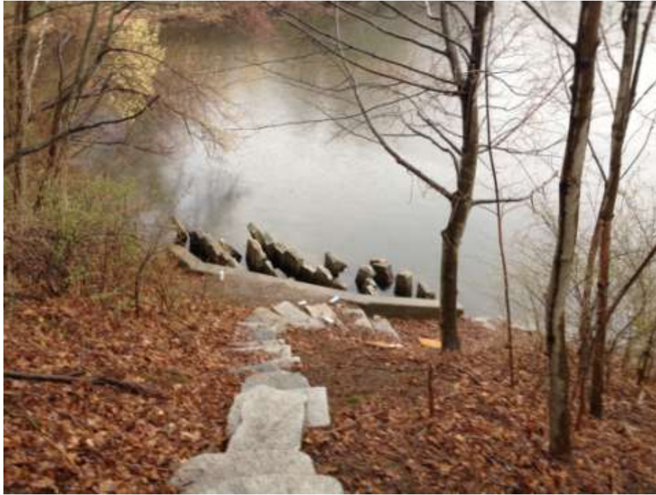
Outfall 6585 Located at Spy Pond, Arlington MA
