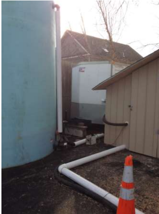
DPE System with temporary holding tank
