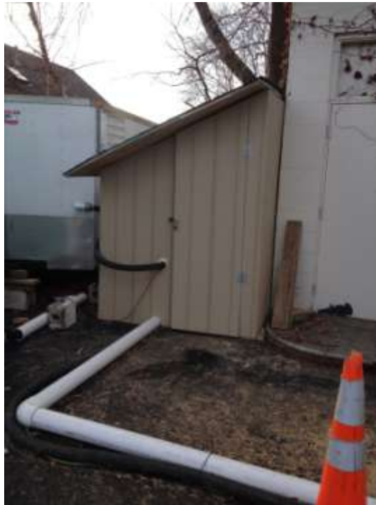
System Enclosure located at 350 Pleasant Street
