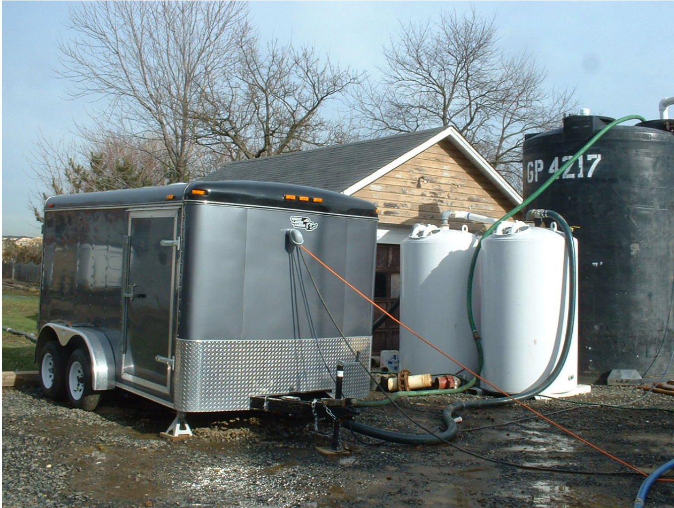
ABOVE – View of Mobile Treatment Trailer and GAC filters
