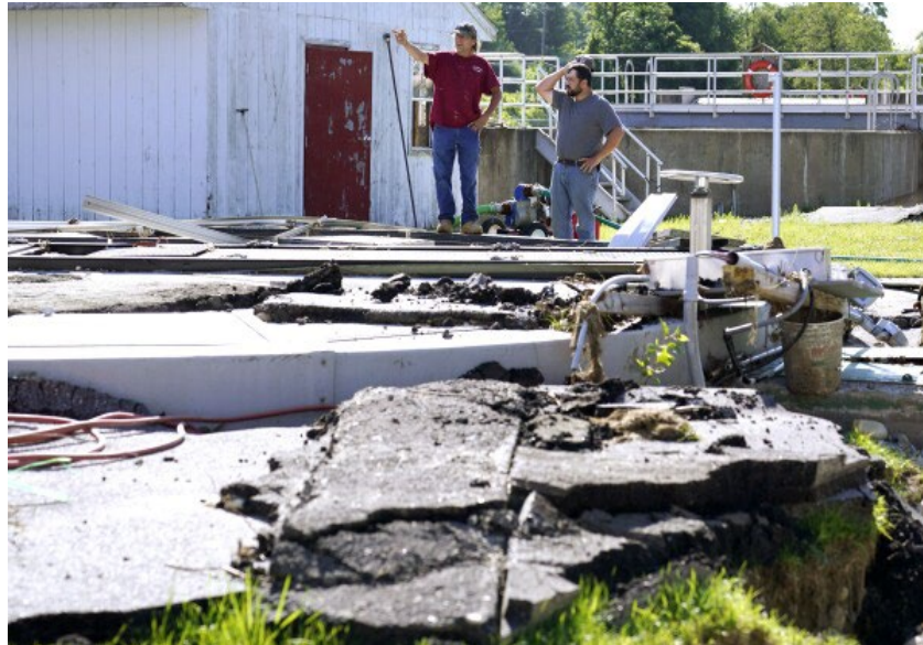
Figure 2: Ludlow Wastewater Treatment Plant (photo August 2, 2023, taken after July storm event) 17
