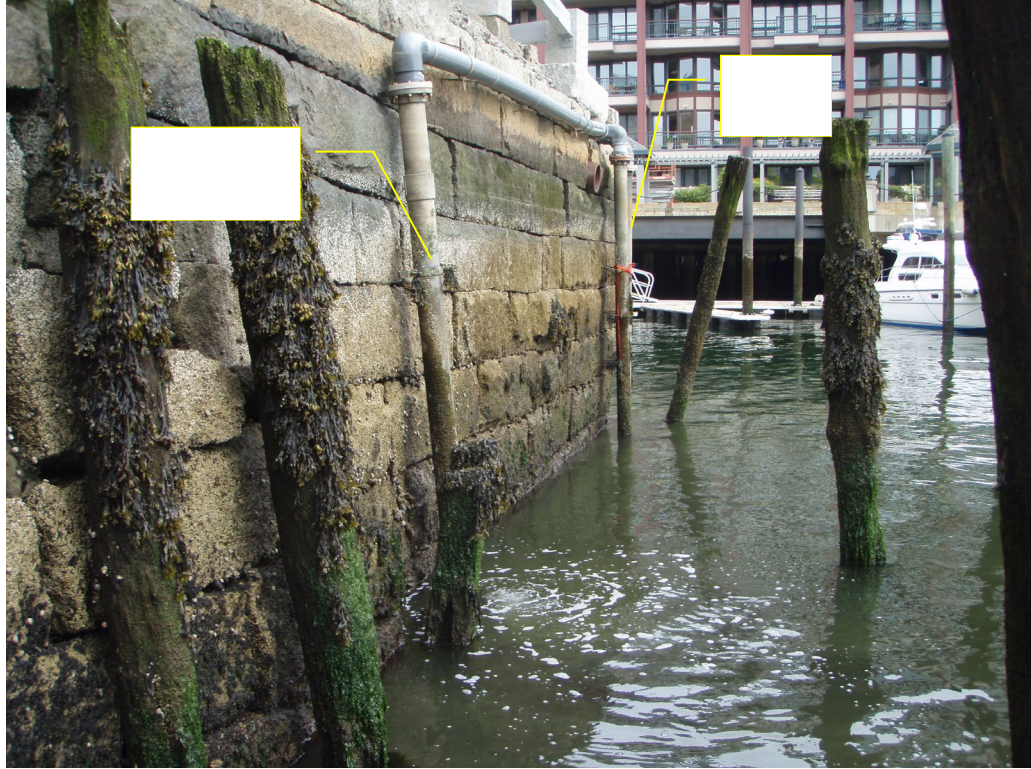
Figure 3: Intake and Discharge Pipes on Union Wharf Seawall
