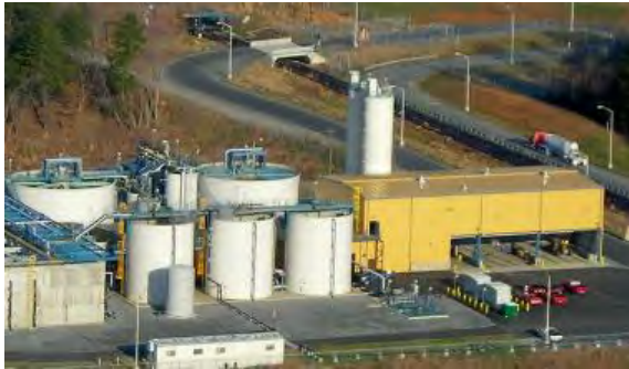
Figure 1 – FGD Physical/Chemical Treatment System (Courtesy of GE/Siemens/Duke Energy)
