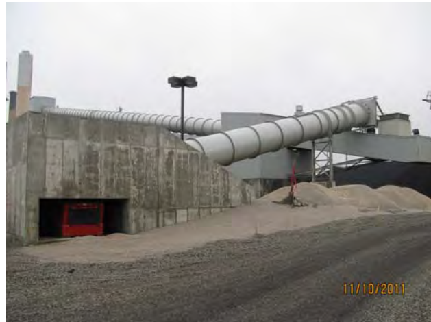
Limestone Conveying System
