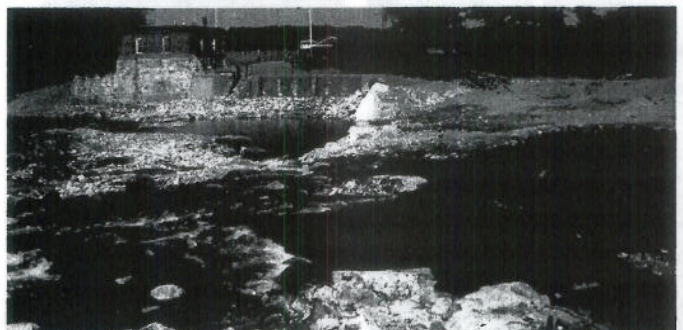
Removal of the Madison Electric Works Dam on the Sandy River in Norridgewock, Maine. The dam was removed in the summer of 2006, allowing diadromous fish access to the watershed of Maine's 12th largest river. Eric Hutchins
