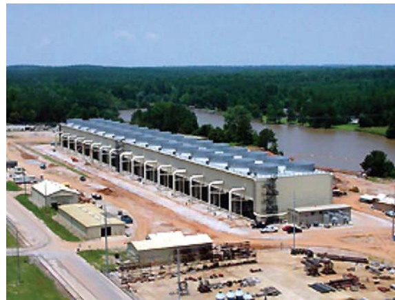
Figure 28-3 32 Cell, Mechanical-Draft, Counterflow Wet Cooling Tower
