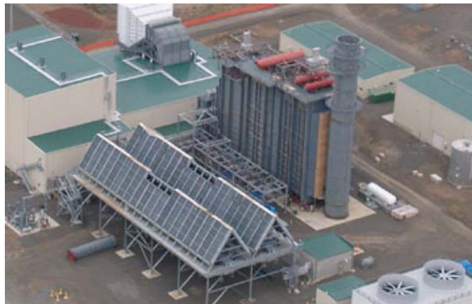
Figure 28-8 Hybrid Water-Conservation Cooling System (shown with a 10 Cell Air-Cooled Condenser and a 2 Cell Wet Cooling Tower)
