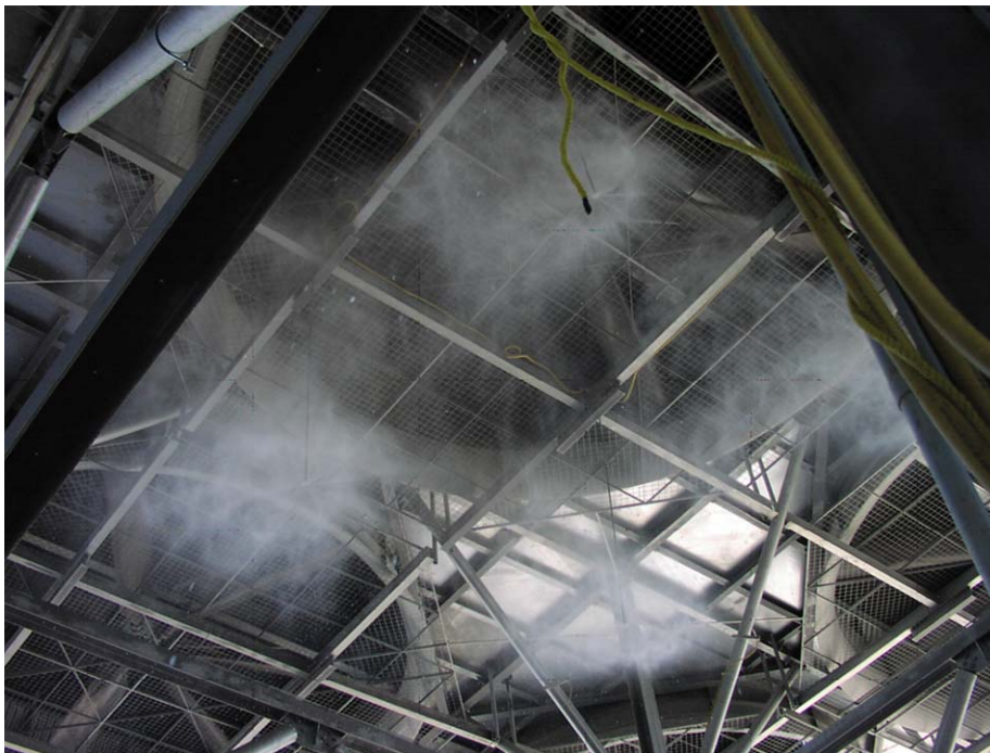
Figure 28-15 Spray Nozzle Arrangement at Bighorn Power Plant
