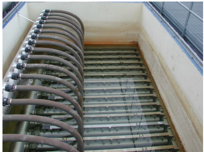
Figure 1 GWRS microfiltration system (Photo Credit: Gina DePinto)
