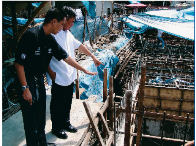
Figure 3 LINAW Team Leader for Muntinlupa City John Emmanuel Pabilonia and former Muntinlupa City Mayor Jaime Fresnedi inspect the construction of the public market treatment facility.
