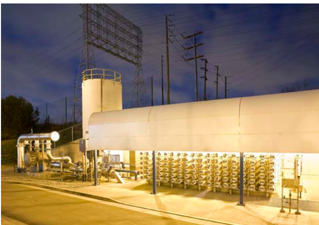
Figure 2 Reverse osmosis treatment at the ECLWRF
