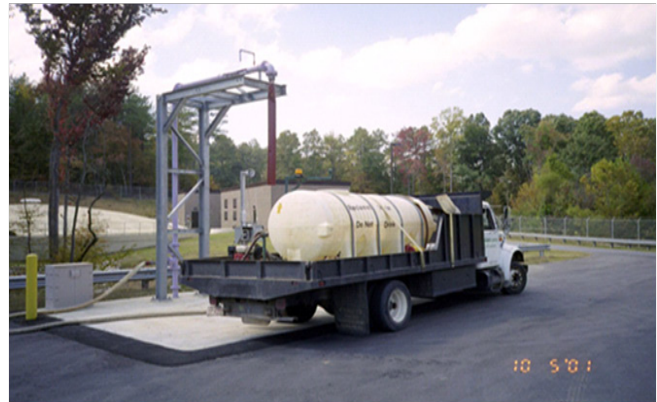
Figure 5-14 Cary, N.C., bulk fill station allows approved contractors, landscapers, and town staff to use reclaimed water
