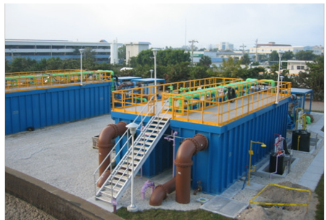
Figure 1 Marco Island WWTP membrane trains (Photo credit: Jeff Poteet)
