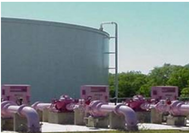
Figure 2-8 Reclaimed water pumping station, San Antonio, Texas (Photo credit: Don Vandertulip)
