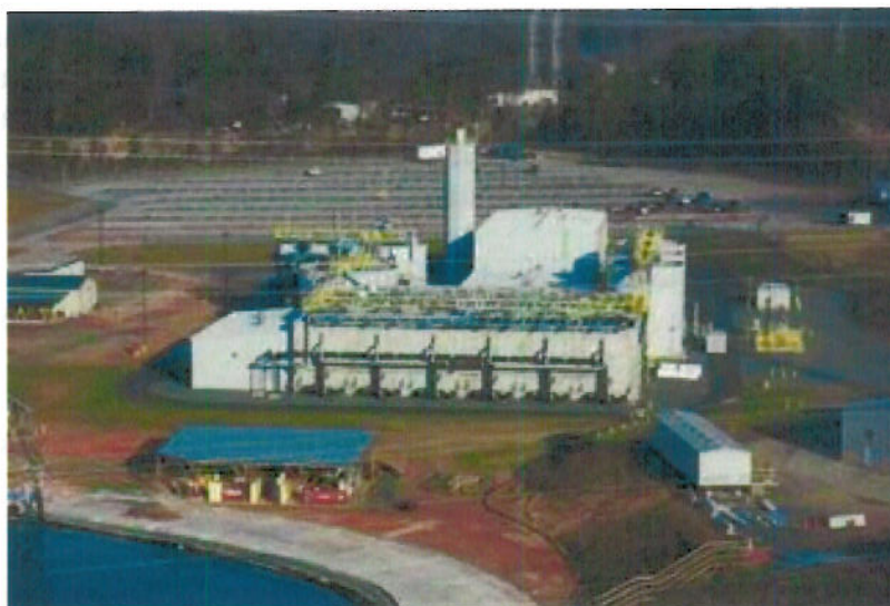
Allen Station wastewater treatment system. Photo courtesy Duke Energy.
