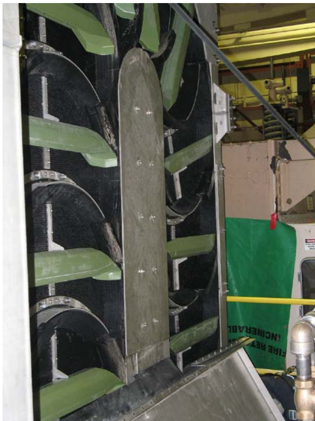
Figure 2-23 Image of Geiger screen installed at Fort Calhoun Station
