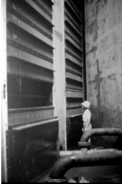
Figure 10-2 Oswego angled screen intake system dewatered (courtesy of Alden Research Laboratory, Inc.)
