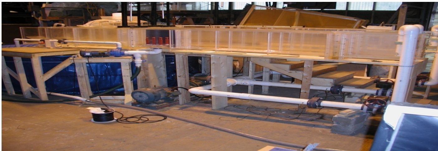
Figure 17-4 Schematic with approximate distances between system components and egg and larvae release and collection locations and photograph of Filtrex Test Facility (Alden 2007)
