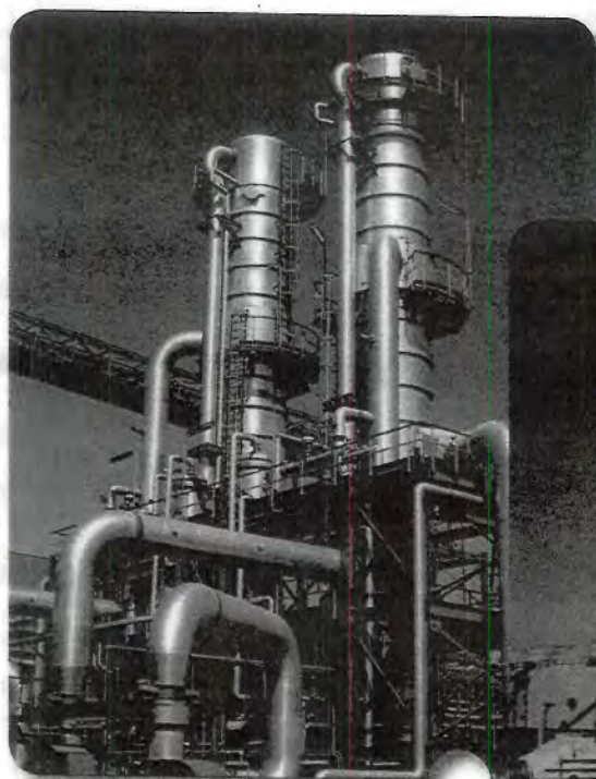
FGD Waste ZLD System
