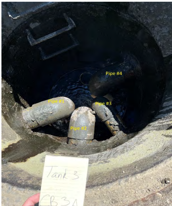
PHOTO 6: Catch Basin (CB-3A) following clean out within Tank 3 with several pipes; typical.
