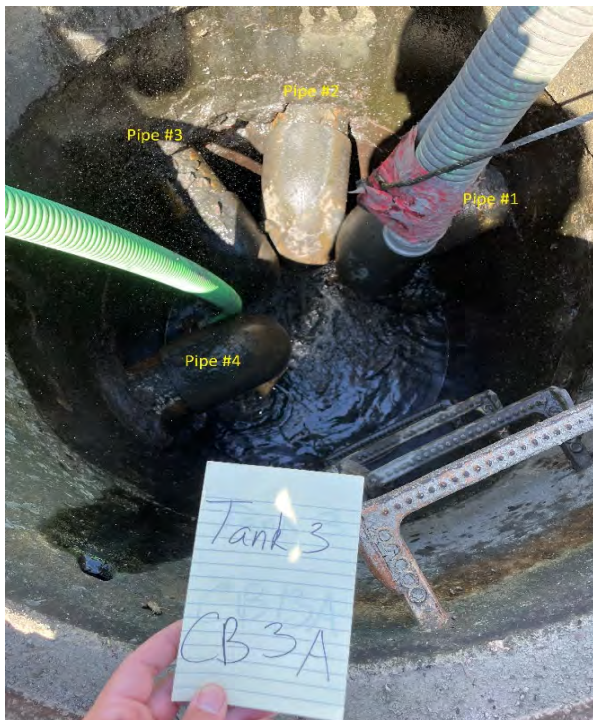
PHOTO 5: Catch Basin (CB-3A) prior to clean out within Tank 3 with several pipes; typical.
