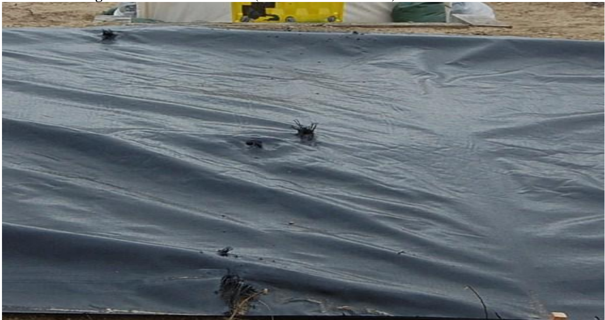
Figure 12. 100 Meter GTL (Plastic Frontal Cover) on 26 October 2010
