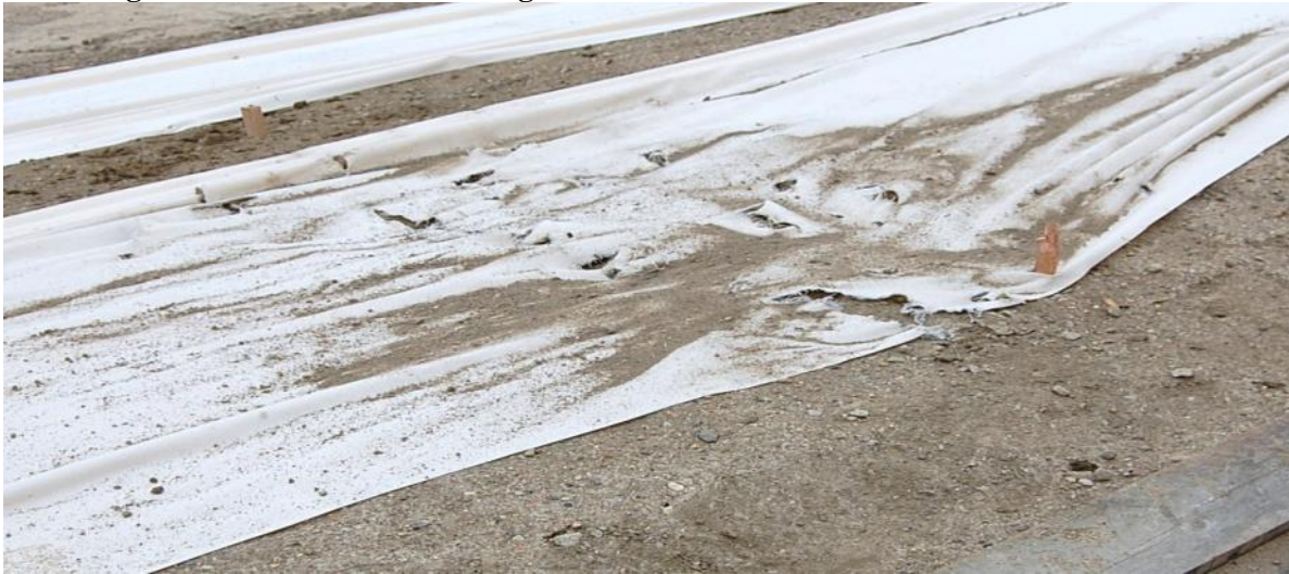
Figure 24. 300 Meter Gun Target Line Earthen Berm and Cover on 25 October 2010
