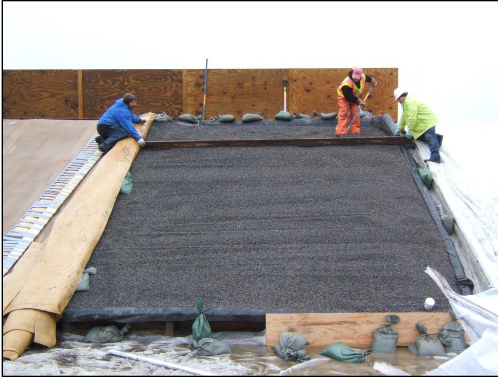
Figure 9. Tango Range Lanes 14 and 15, Re-Installing Rubber Granules after Mass Balance Work, Camp Edwards, Massachusetts
