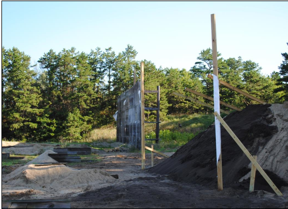
Figure 7. Eastern Backstop Berm Supplemental Test Fire 2:1 Slope Echo Range Camp Edwards, Massachusetts
