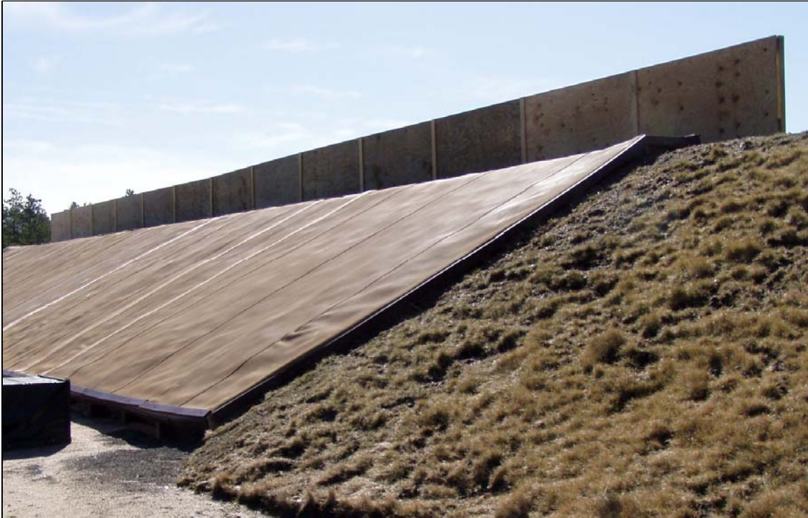
Figure 10. Plywood Overshot Telltale Wall, Tango Range, Camp Edwards, Massachusetts.
