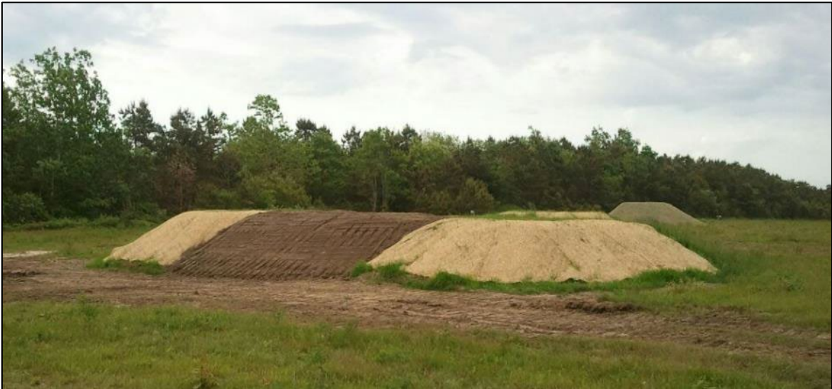
Figure 5. Sierra Range Targets Berms with Core Material (Background), Sand, Top Soil and Erosion Control Matting, Camp Edwards, Massachusetts
