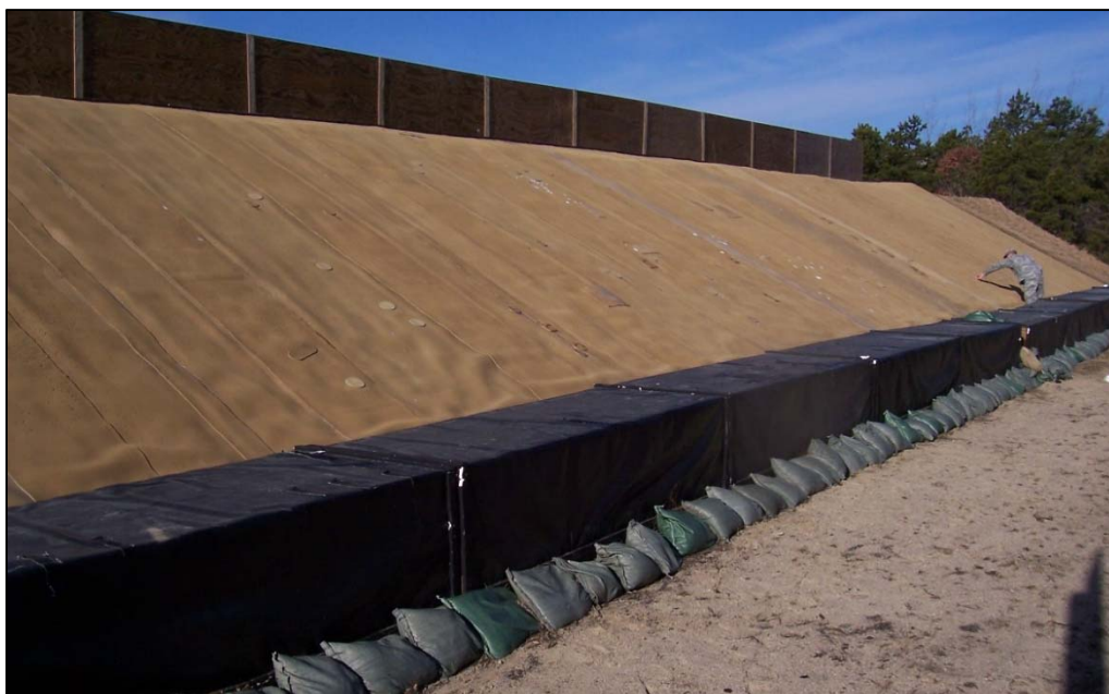
Figure 3. Toe-Berm Boxes, Tango Range, Protecting STAPP™ system Base and Internal Reservoir, Camp Edwards, Massachusetts.
