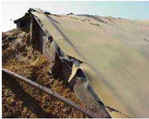
Figure 6-4. Example of Damage to STAPP™ Support Frame
