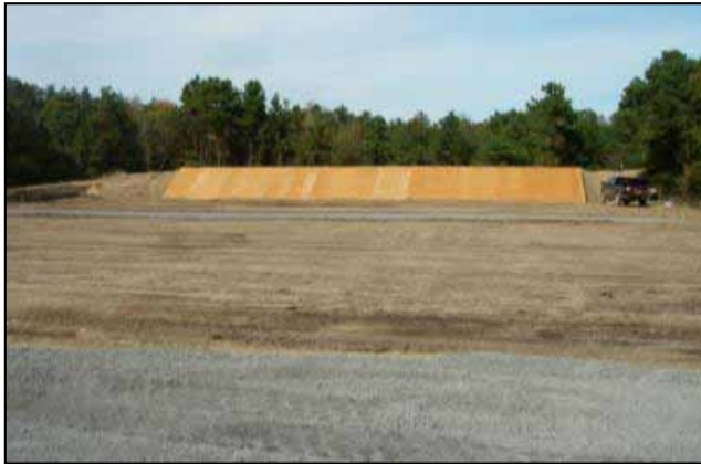
Figure 3-2. Juliet Range Installed with STAPP™
