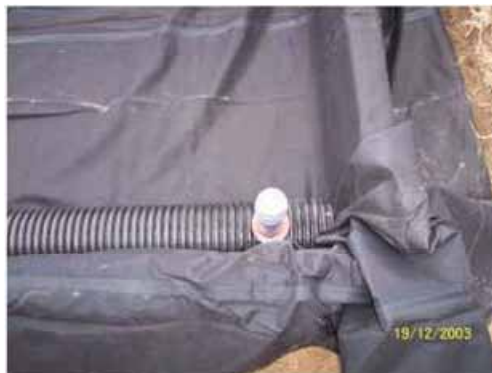
Figure 6-3. Internal Water Reservoir System
