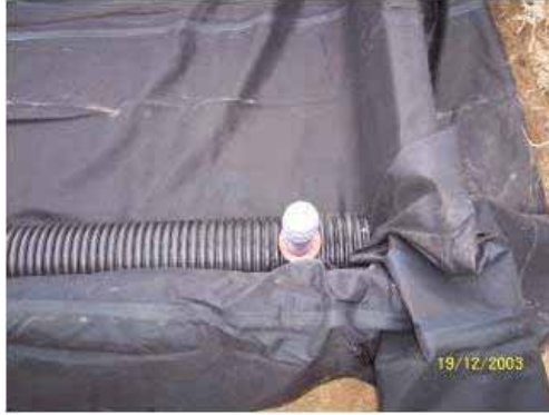
Figure 4-4. Internal Water Reservoir System
