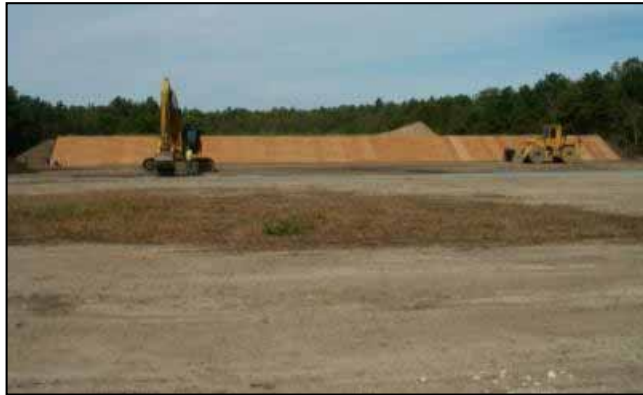
Figure 3-3 Kilo Range Installed with STAPP™
