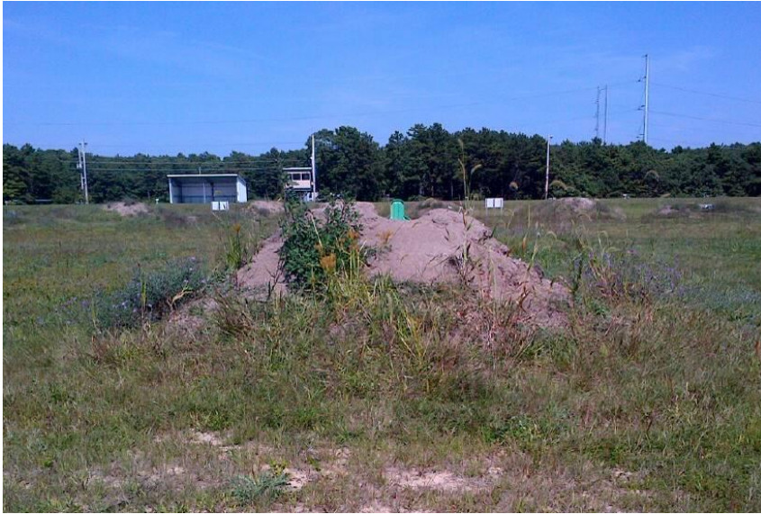
Figure 8-2. Auxiliary berm (facing up range-North) that has ceased to function as intended Sierra Range, Camp Edwards, Massachusetts.
