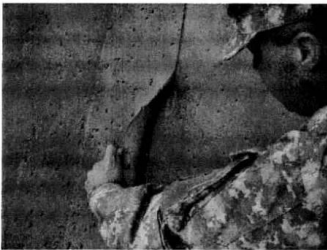
Photograph B-3: Overlapping Sheet of Top Layer of Rubber That Needs to be Re-Sealed.
