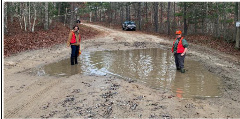
Natural Resources staff preparing for in-situ modifications to FRED puddle. Work will improve conditions for both vehicles and clam shrimp. After draining, fine sediment will be scraped away and the bottom raised and hardened by compacting layers of sand over gravel. Finally, some scraped sediment containing clam shrimp eggs will be returned. Erin Hilley
