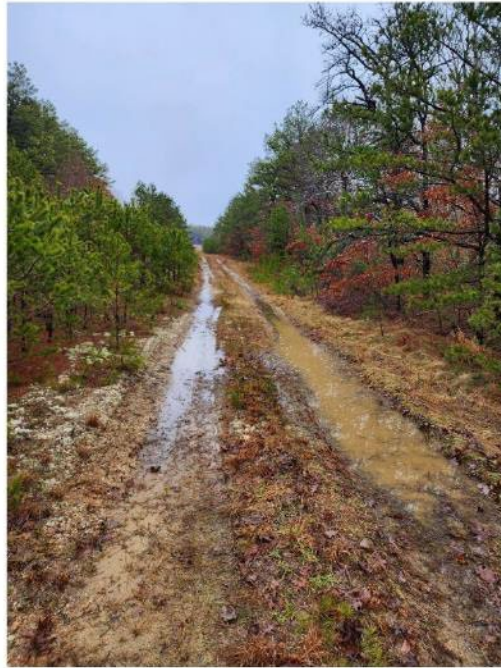
Figure 1; SVL1 rutting and puddles on road leading to SVL3.
