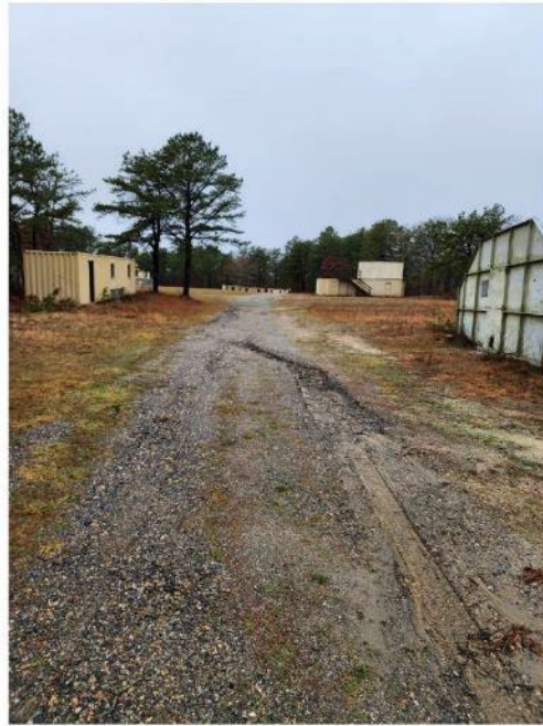
Figure 3: Rutting and erosion at SVL6.
