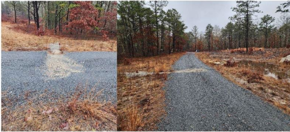
Figure 6 and 7: Rutting and erosion at BP20 (picture location 2).
