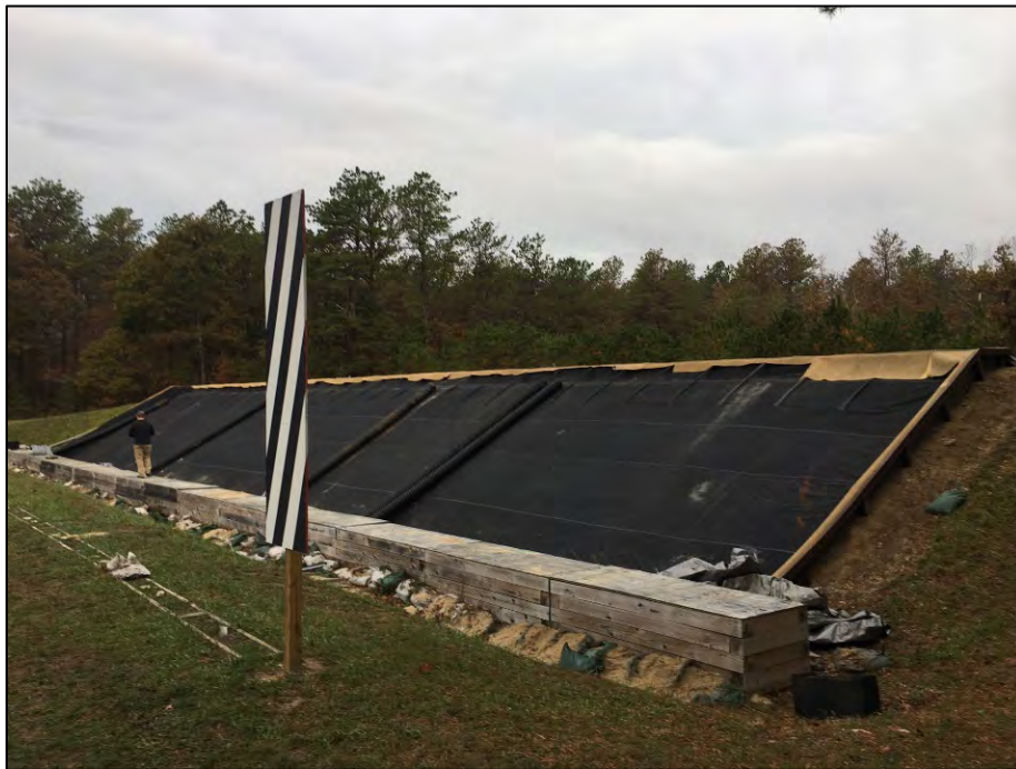
Photograph 2-4 The Juliet Range STAPP™ system cleaned out. The bottom liner is visible.
