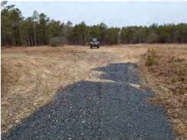
Figure 5: Minor erosion occurring where the gravel road ends at BP-20.
