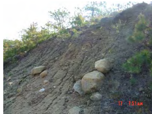
Figure 5-12. A Range Berm Surface Rocks and Erosion
