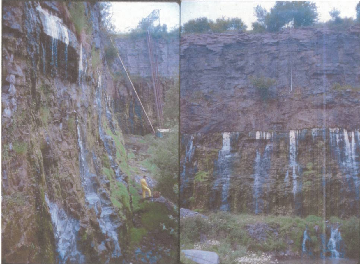
Figure 7 – Seeps on East Wall of Gates Dolomite Quarry (contaminated seeps are in the SE corner)
