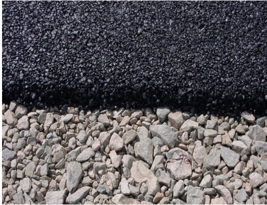
Porous pavement close-up, Aurora, CO. Courtesy of: The Colorado Association of Stormwater and Floodplain Managers (CASFM) .
