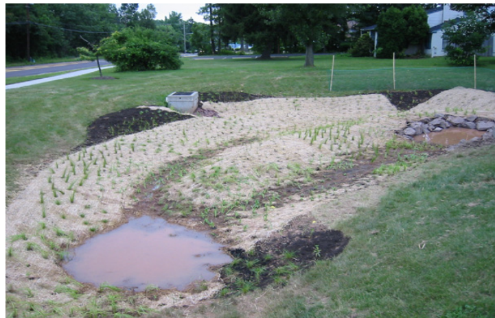
Constructed Wetland Designed by F.X. Browne, Inc.
