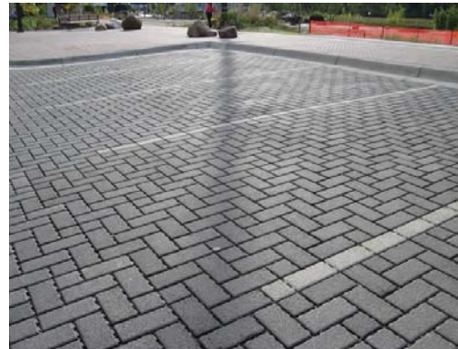
Permeable Pavers at the transit center parking lot in Mound, Minnesota. Courtesy of: Julie Westerland, MN DNR.
