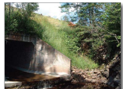
Figure 4. Same slope after revegetation
