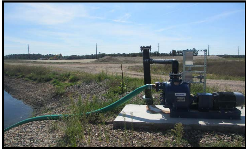
Photo 5.5.4a: Pump at Southwest corner of Southwestern Secondary Pond. Transfers water to the truck washing station on the temporary CCR storage pad adjacent to the management units.
