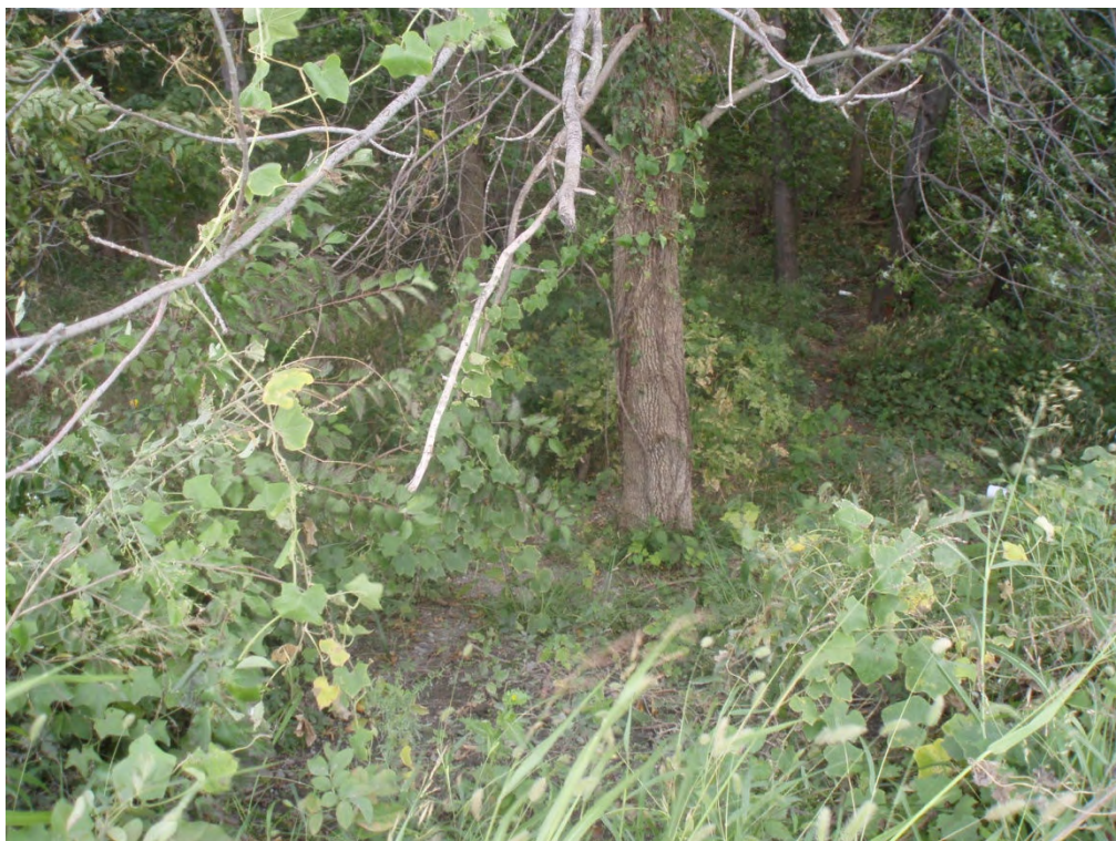
15. Exterior of northwestern dike (Area 4) – 10” tree observed at toe of embankment.
