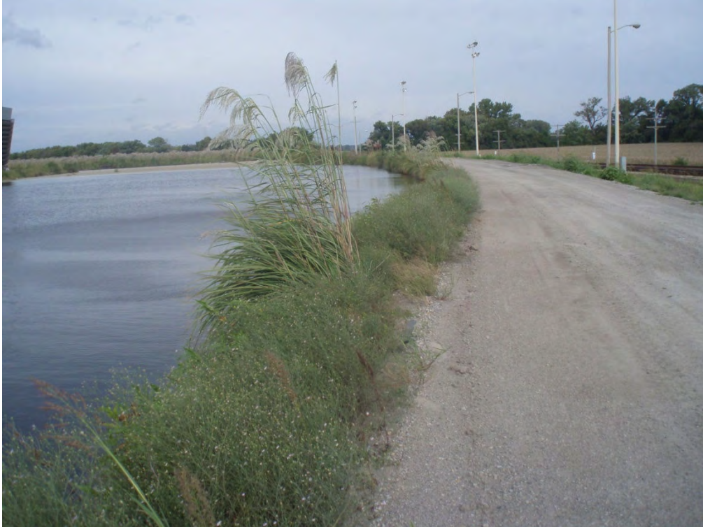
3. Interior of north dike – Taken from east end of Area 1, looking west
