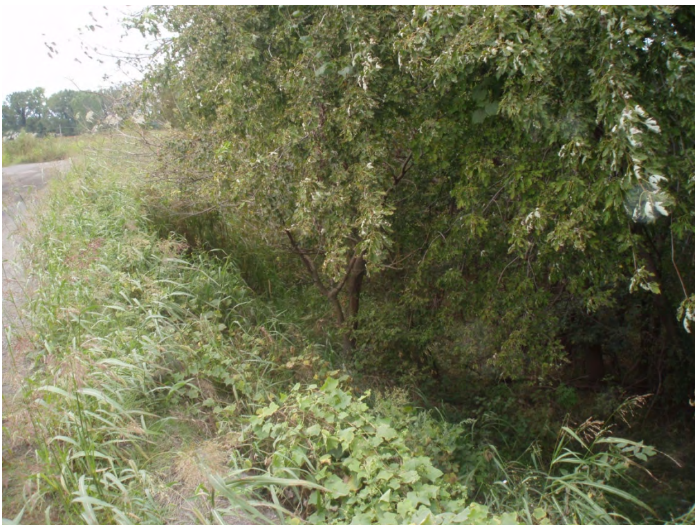
13. Exterior of northwestern dike (Area 4) – heavy vegetation and trees observed.
