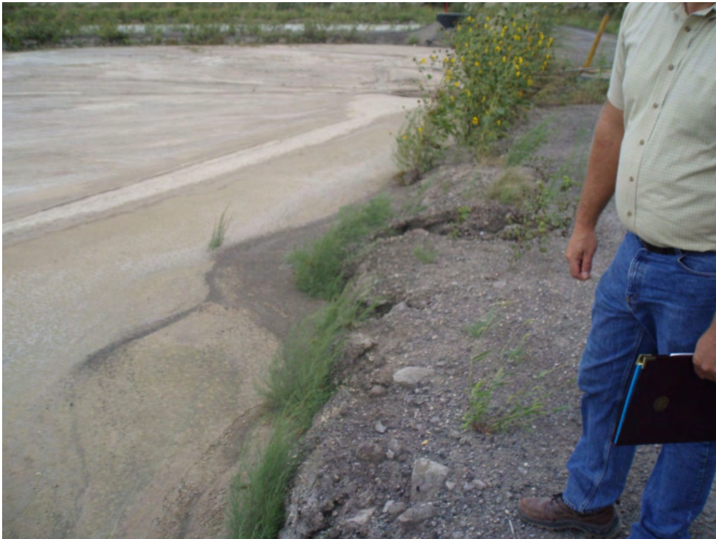
10. Interior of northern dike in Area 2 – Some minor washout/erosion observed.
