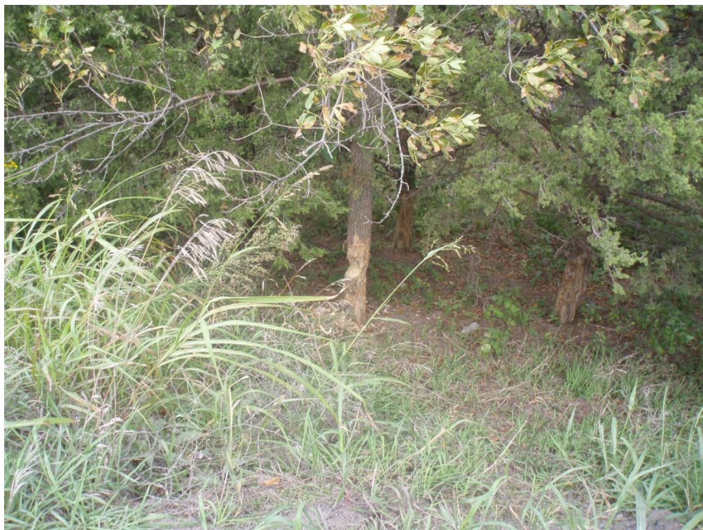
18. Exterior of northwestern dike (Area 4) – 10" tree observed at toe of embankment.
