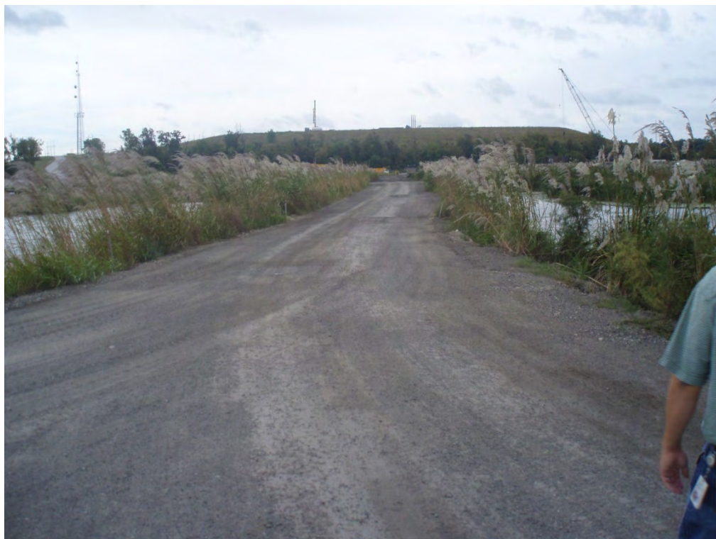
8. Interior separation dike, separating Area 1 from Area 2 - Taken from north end, looking south.
