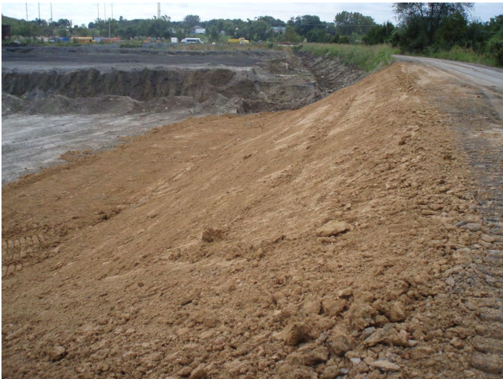
20. Interior of western dike (Area 3) – Taken from western dike looking south along interior of dike. Clay liner being installed
