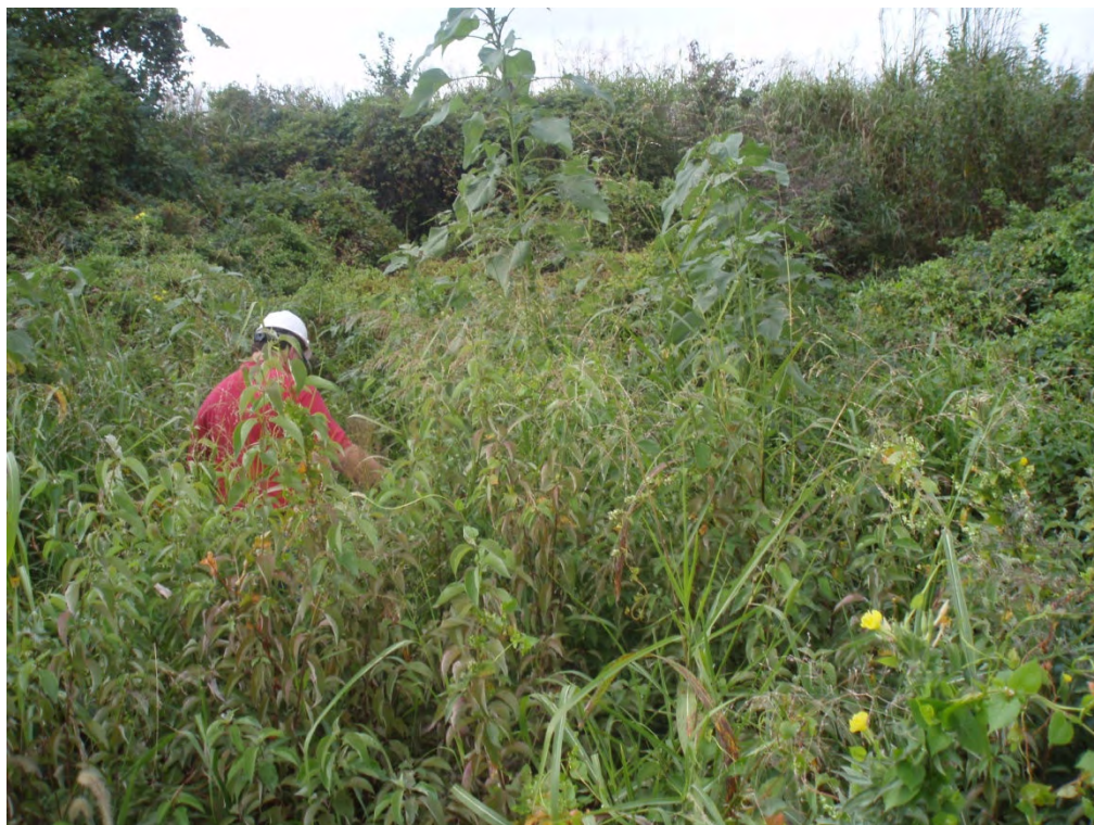
6. Outfall of emergency overflow structure – exterior of north side of Area 1 dike. Heavy vegetation made access to the outfall impractical.
