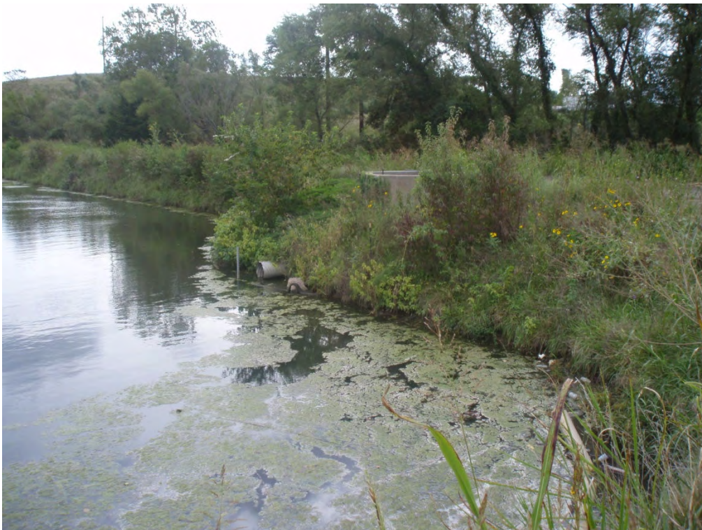
24. Storm water pond discharge pipe on interior of south side of dike.
