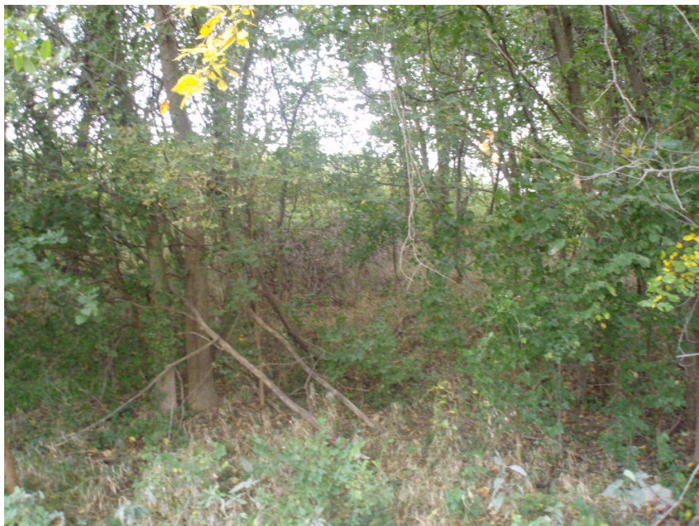
7. Exterior of dike – Taken from north side of Area 2 looking south, up side of dike.
