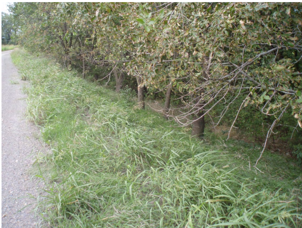
16. Exterior of northwestern dike (Area 4) – multiple trees observed on embankment.
