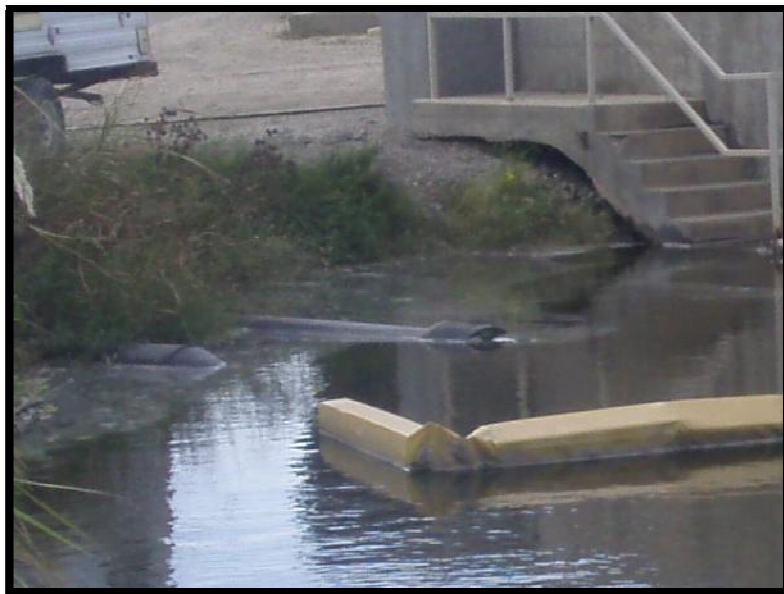
Figure 5.5.2-1: Inlet end of the Clear Water Pond Outlet Structure that leads to the Kansas River.
