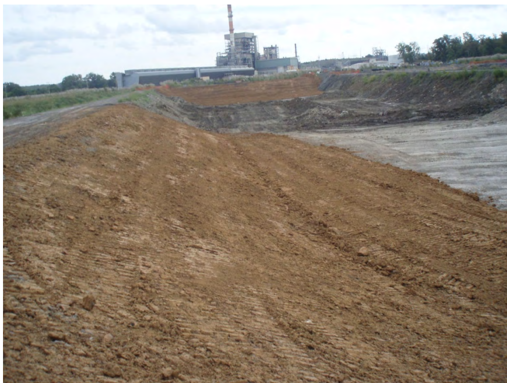
21. Interior separation dike (Area 3) – Taken from western dike looking east along interior separation dike. Clay liner being installed
