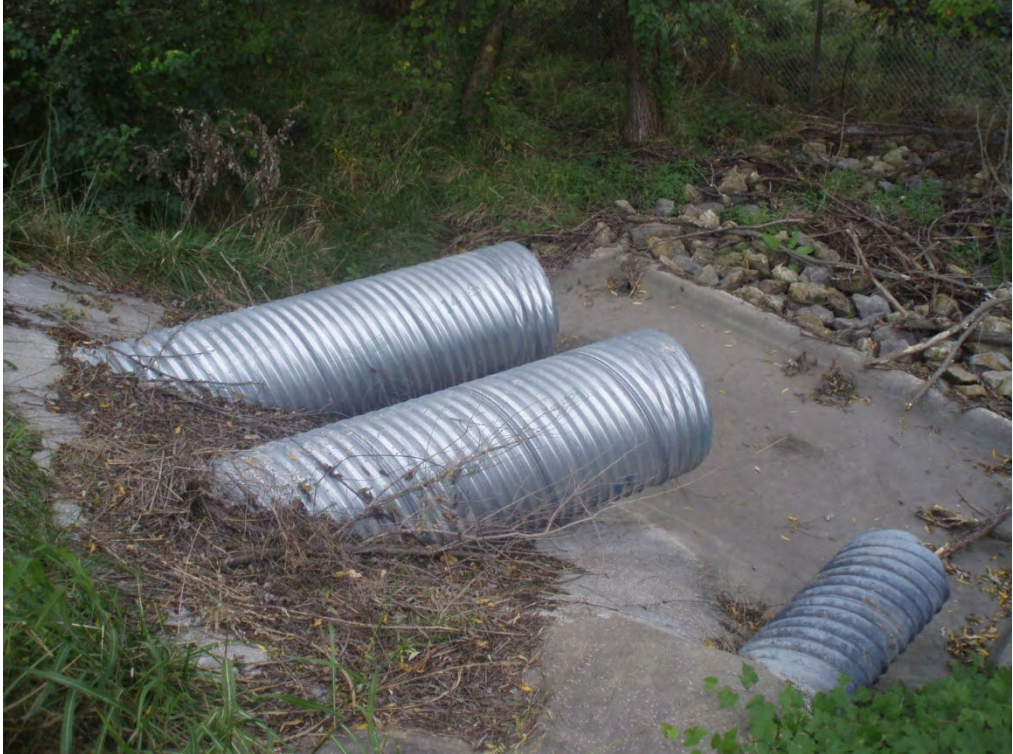
25. Storm water pond outfall pipes on exterior of south side of dike.
