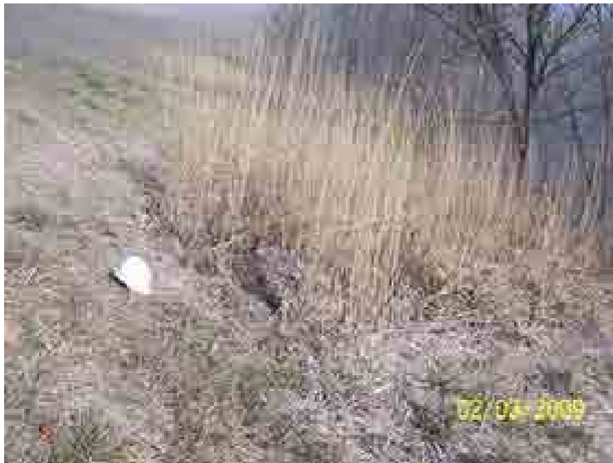
Drawing Mark GP-1-6 Seepage observed below the perimeter dike along the southeast side of the Gypsum Stack.
