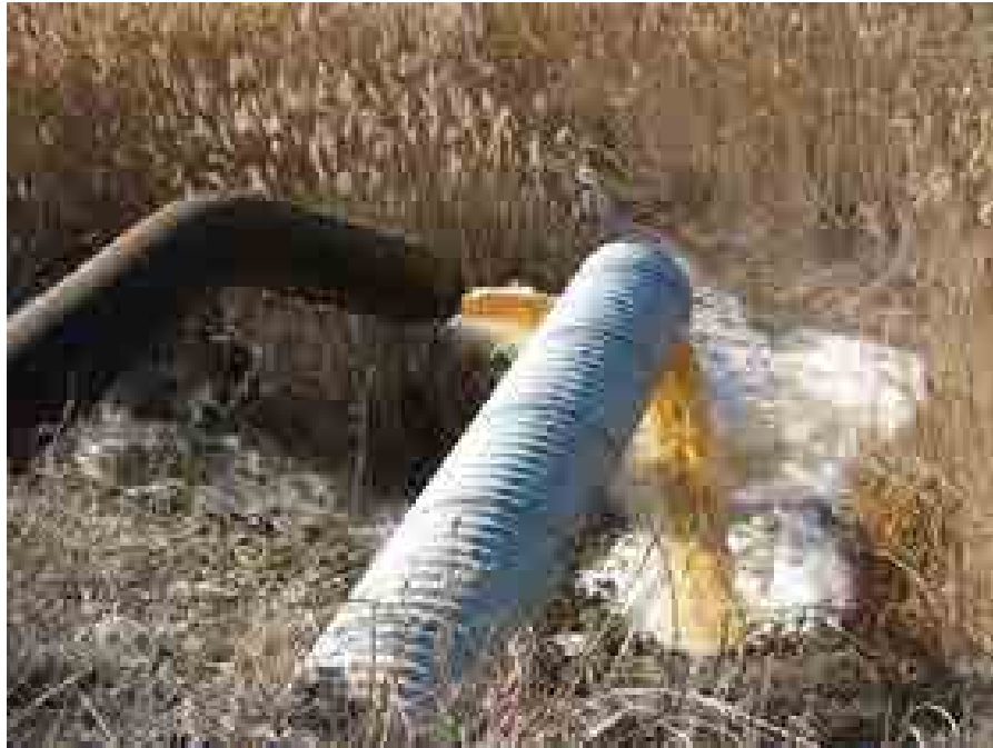
Drawing Mark GP-1-7 Discharge pipes and riprap channel along northwest corner of Gypsum Storage Area.
