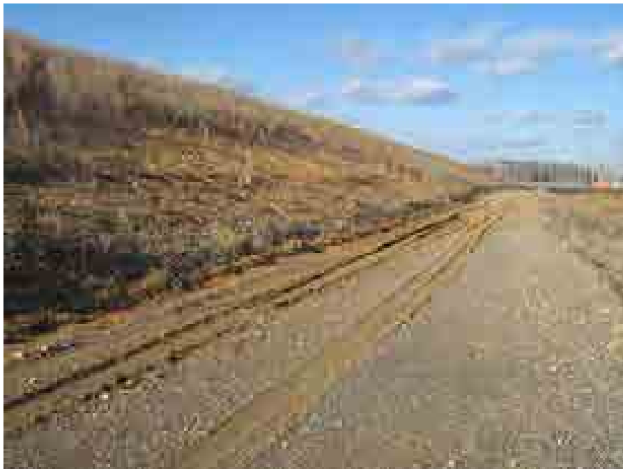
Drawing Mark DS-1-4 Exposed soil and erosion along southeast face of Dry Ash Stack.
