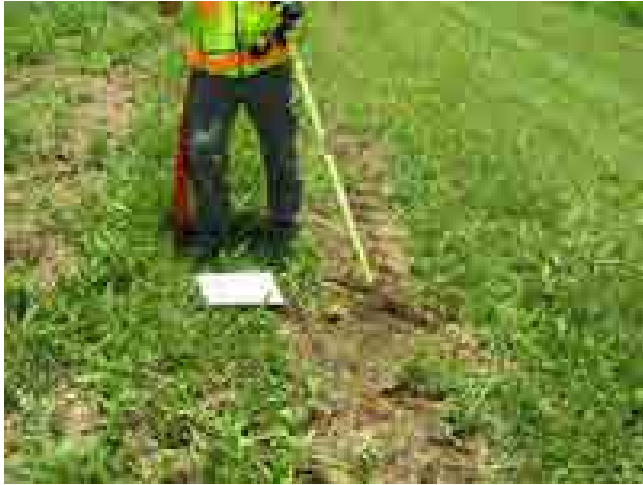
Photo 13 Rutting on exterior slope of the dike
