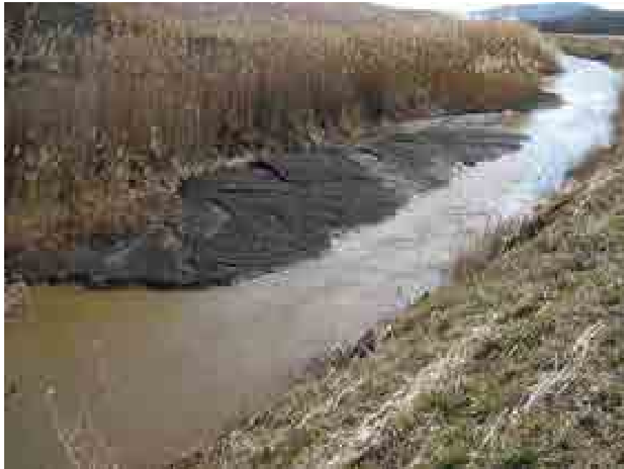
Drawing Mark DS-1-1 Eroded ash from the adjacent dry stack deposited within the west perimeter ditch.
