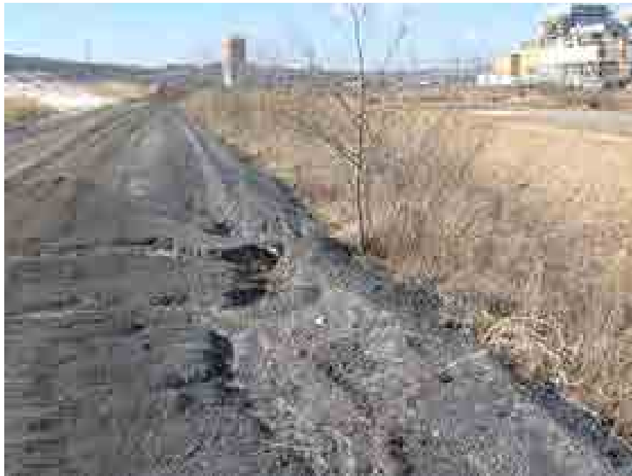
Drawing Mark GP-1-3 Trees and erosion along the perimeter ash dike at the northeast side of the Gypsum Storage Area.
