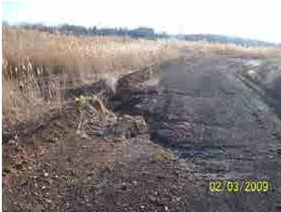
Drawing Mark DS-1-5 Erosion and rutting along access road at the base of the Dry Ash Stack.
