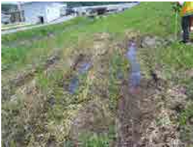
Photo 9 Ponding/Rutting below subdrain #21.
