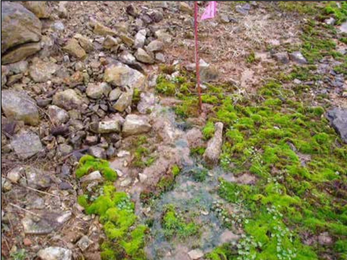
Figure 3. Example of Action Level 2 – Clear Flowing – Seepage Boil
