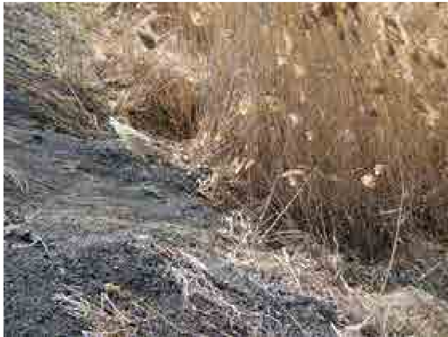
Drawing Mark GP-1-2 Small slope slough along ash divider dike outslope at NW side of the Gypsum Storage Area.
