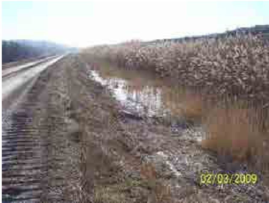
Drawing Mark GP-1-5 Heavy vegetation and sedimentation in perimeter drainage ditch along the southwest and southeast sides of the Gypsum Stack.
