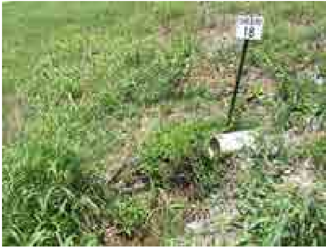
Photo 8 Erosion noted below subdrain 18.
