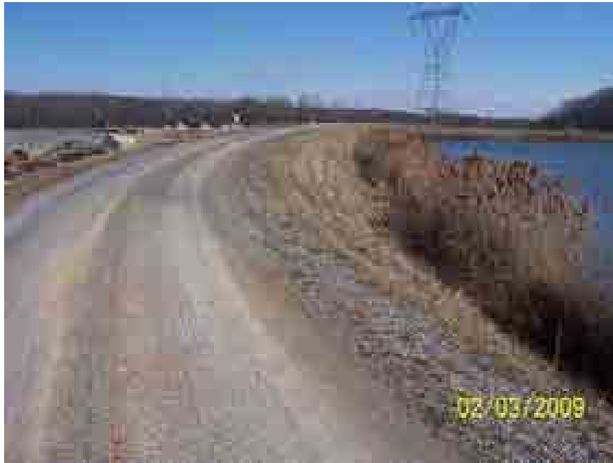
Drawing Mark AP-1-1 Crest and inside slopes of the perimeter dikes around the Ash Pond.
