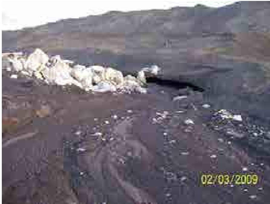
Drawing Mark DS-1-3 Erosion around existing rock check in north portion of Dry Ash Stack
