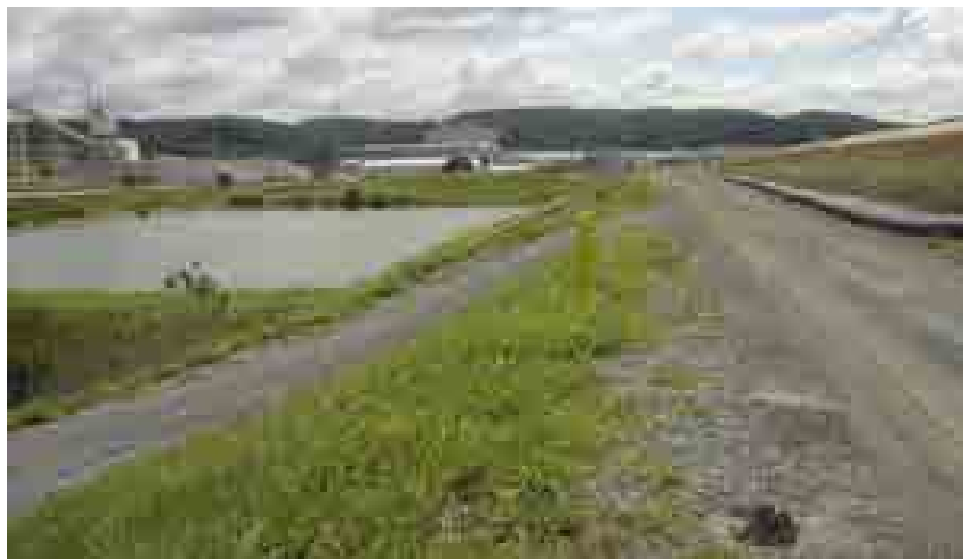
Figure 5.2.3-2 Photo showing outside slope, North Dike. Incised Bottom Ash Pond is on left side of the photo
