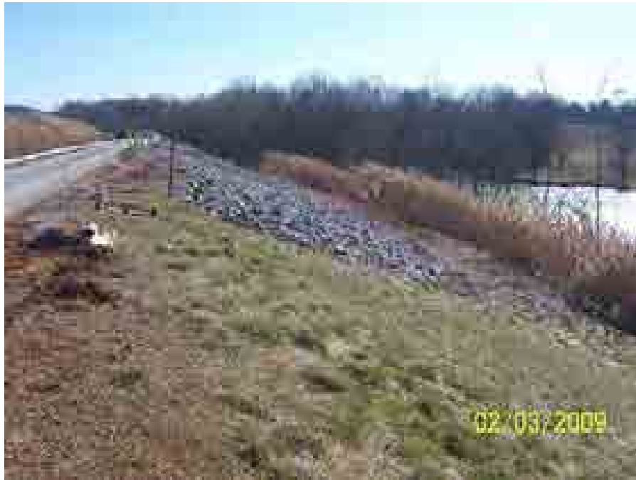
Drawing Mark GP-1-1 Riprap placed in area to temporarily repair slope slough along the perimeter dike at the NW corner of the Gypsum Stack.
