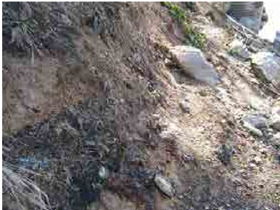
Drawing Mark DS-1-2 Seepage observed below the perimeter dike along the banks of Wells Creek.
