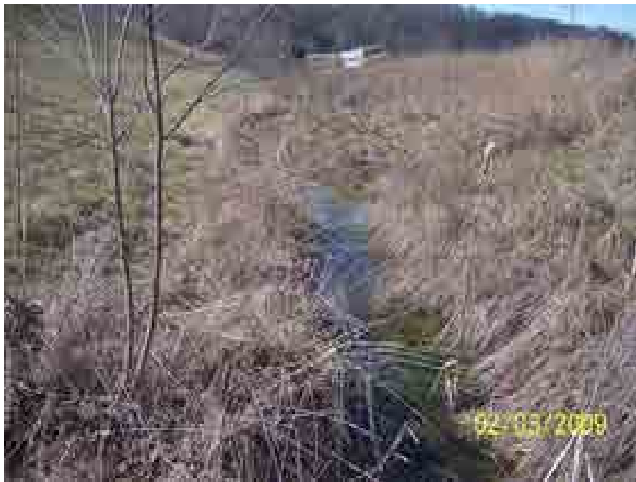
Drawing Mark AP-1-3 Standing water along toe of north perimeter Ash Pond dike.
