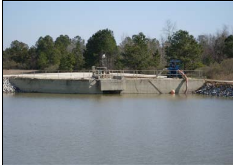
Photograph 5.17. View of discharge pump structure and auxiliary pump, looking northeast.
