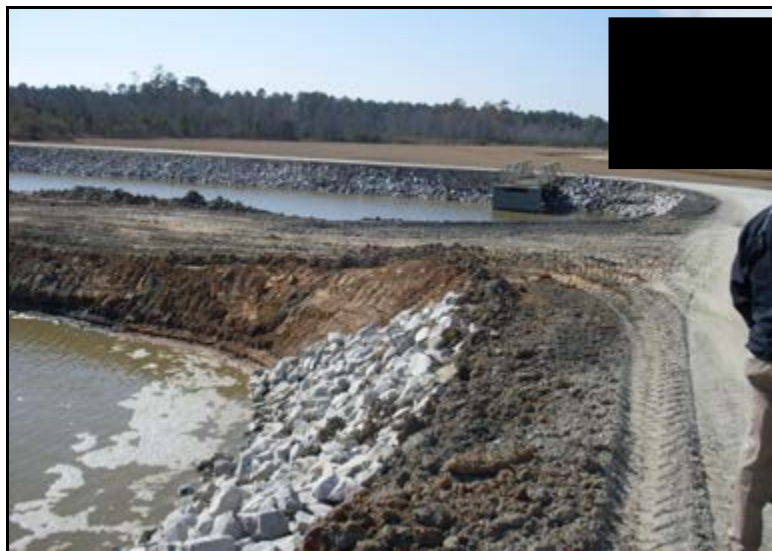
Photograph 5.9a. View of crest, inside slope, finger dike, and emergency overflow structure, northwest side looking southwest.
