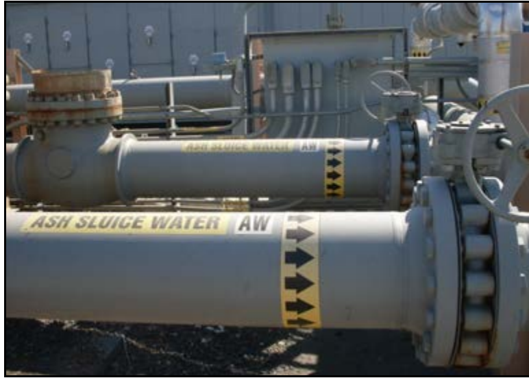
Photograph 5.13. Ash sluice lines to plant.
