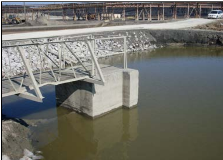
Photograph 5.15. Emergency overflow structure.
