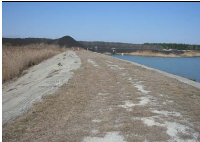
Photograph 5.2. View of crest and inside slope of Bottom Ash Pond 1 northeast dike, looking northwest.
