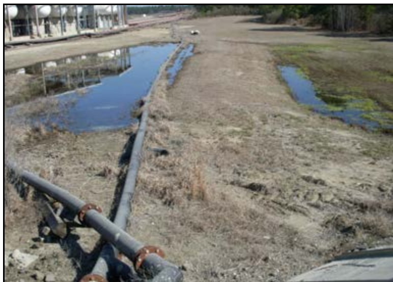
Photograph 5.18. View of pipes conveying water from Gypsum Pond to Bottom Ash Pond 2.
