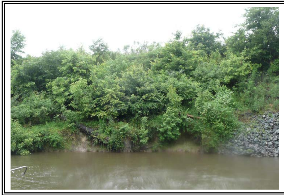
Erosion at the toe of the 1978 Ash Pond at discharge canal. Also note the fallen tree.
