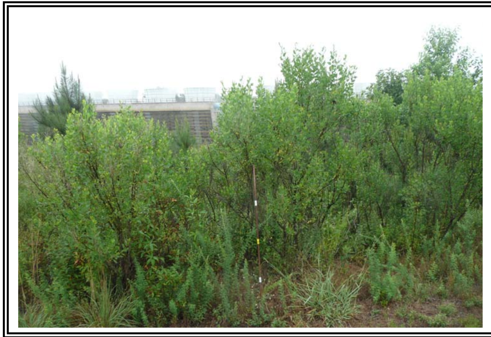
North end of 1978 Ash Pond Dike, downstream slope is covered with large brush.
