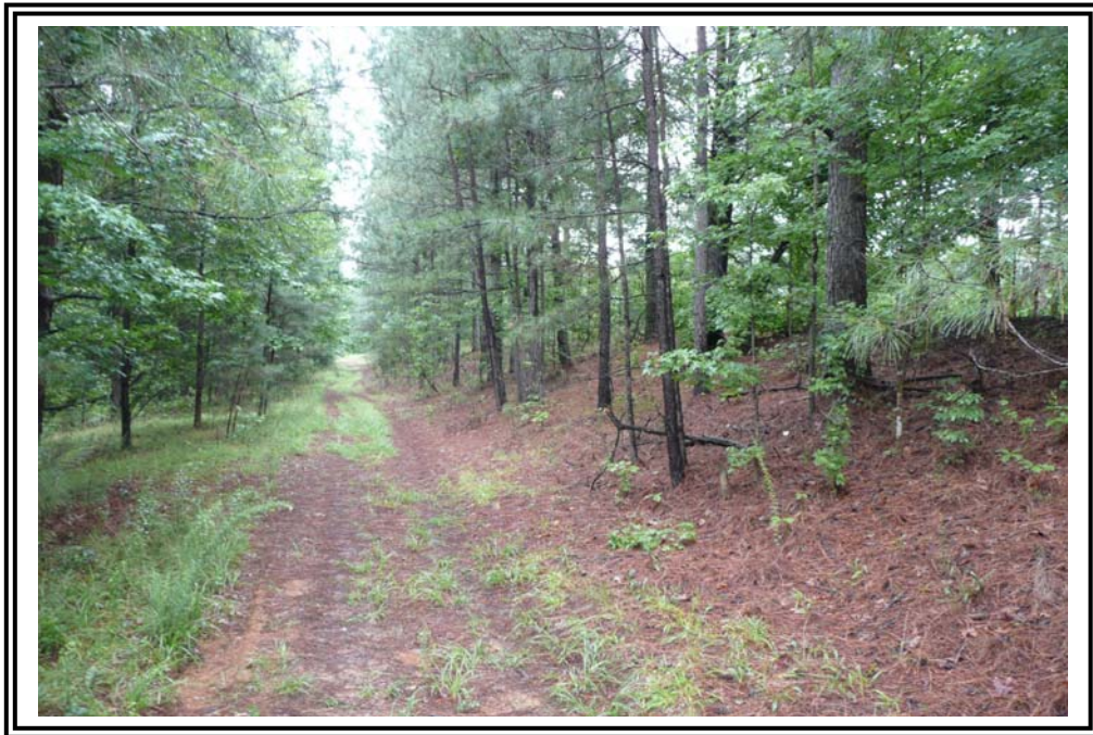
1970 Ash Pond east dike toe looking south. Note road runs along toe of dike in this area.
