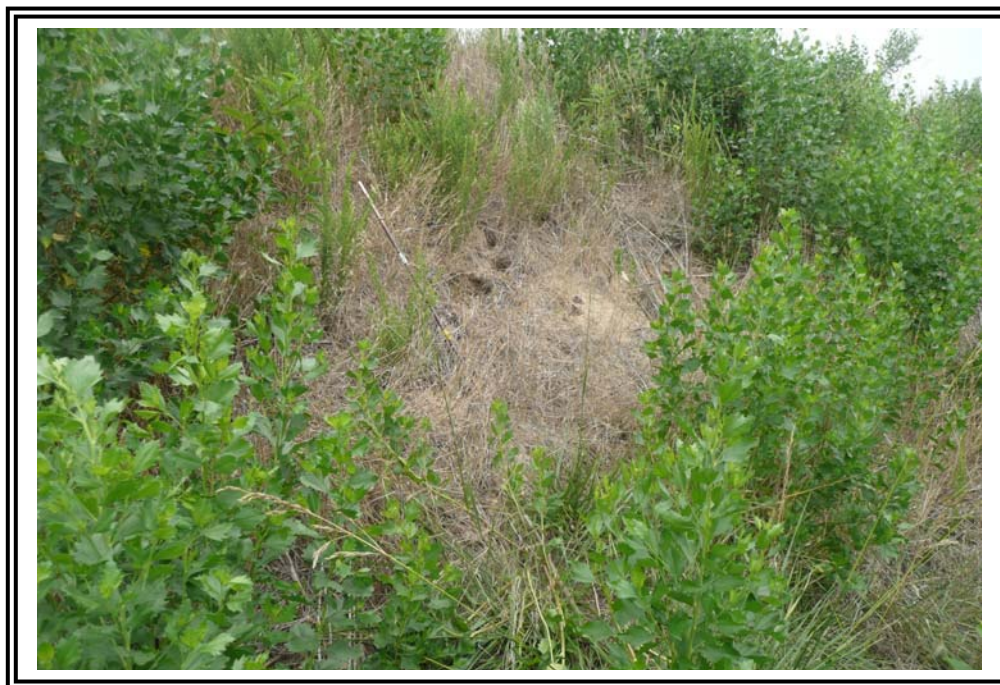
Scarp about 3 to 4 feet high near the top of the 1985 Ash Pond West Dike.
