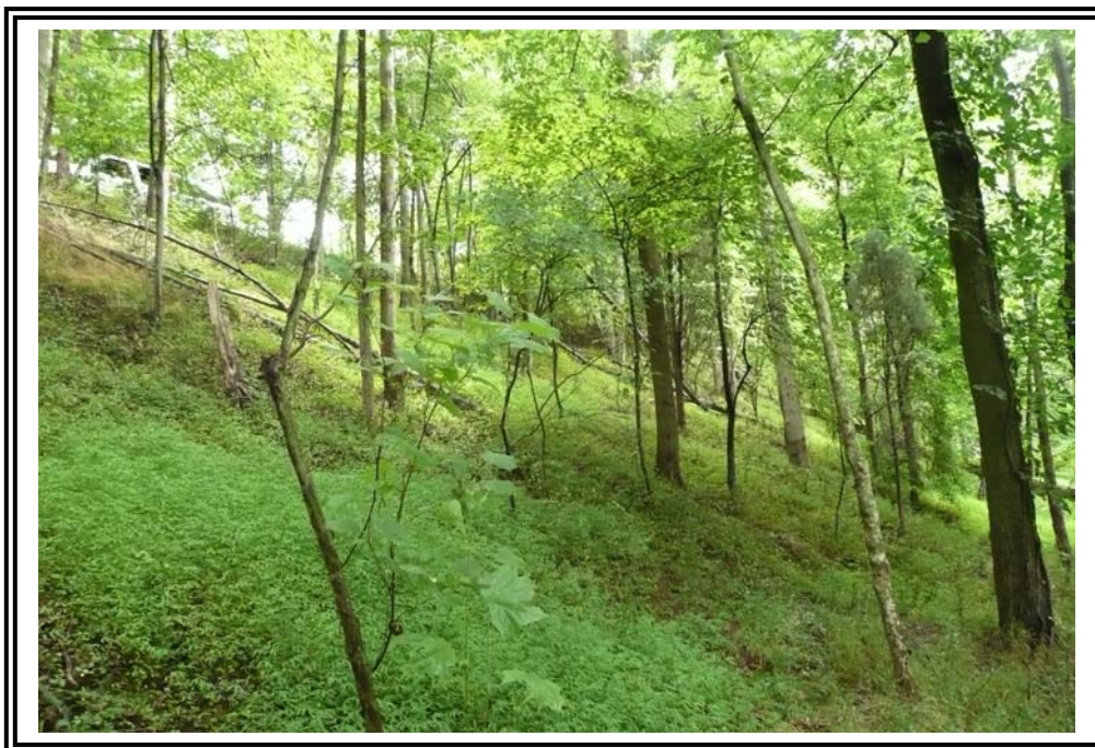
Downstream slope of 1963 Ash Pond west dike. Note suburban parked on crest for scale.
