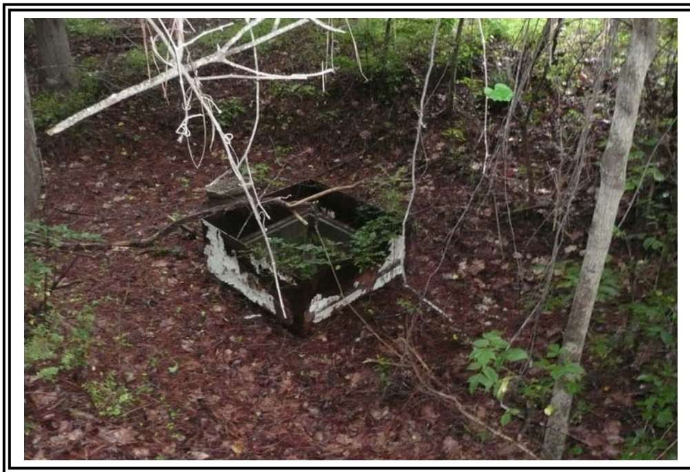
1970 Ash Pond outlet control structure. Note: water level in south end of pond was several feet lower than outlet during our visit.
