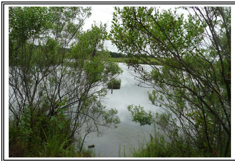
Outlet structure in 1978 Ash Pond.
