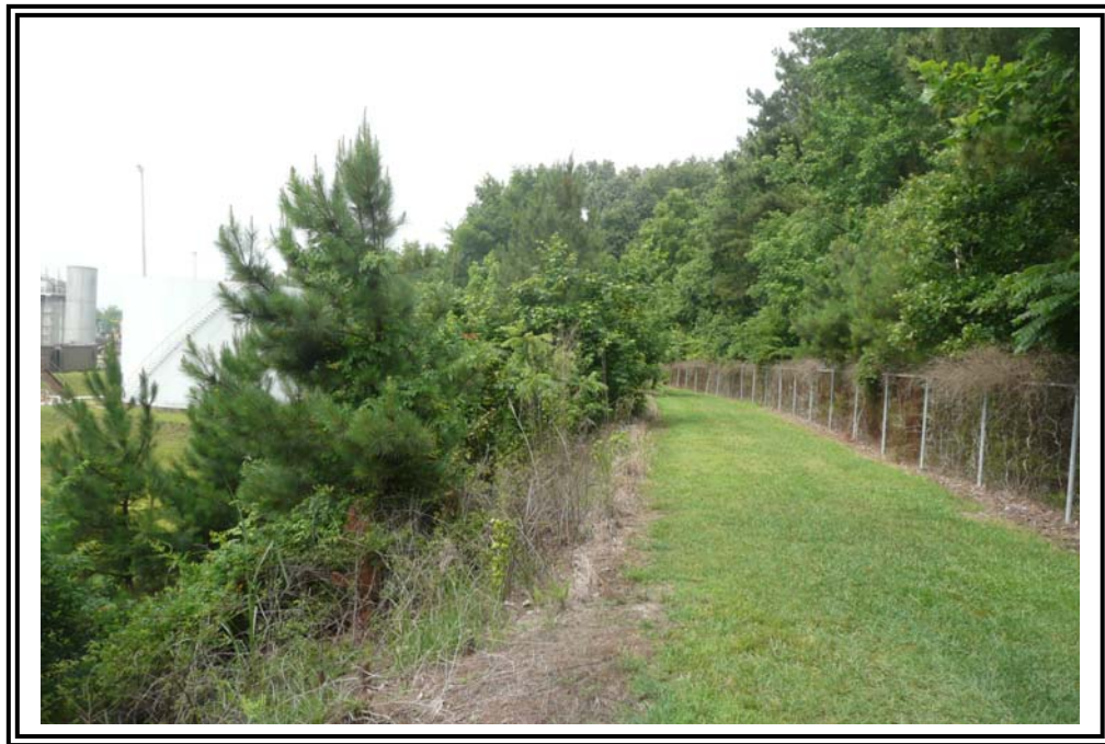
Flood control dike which contained the south side of the 1956 Ash Pond, looking southwest.
