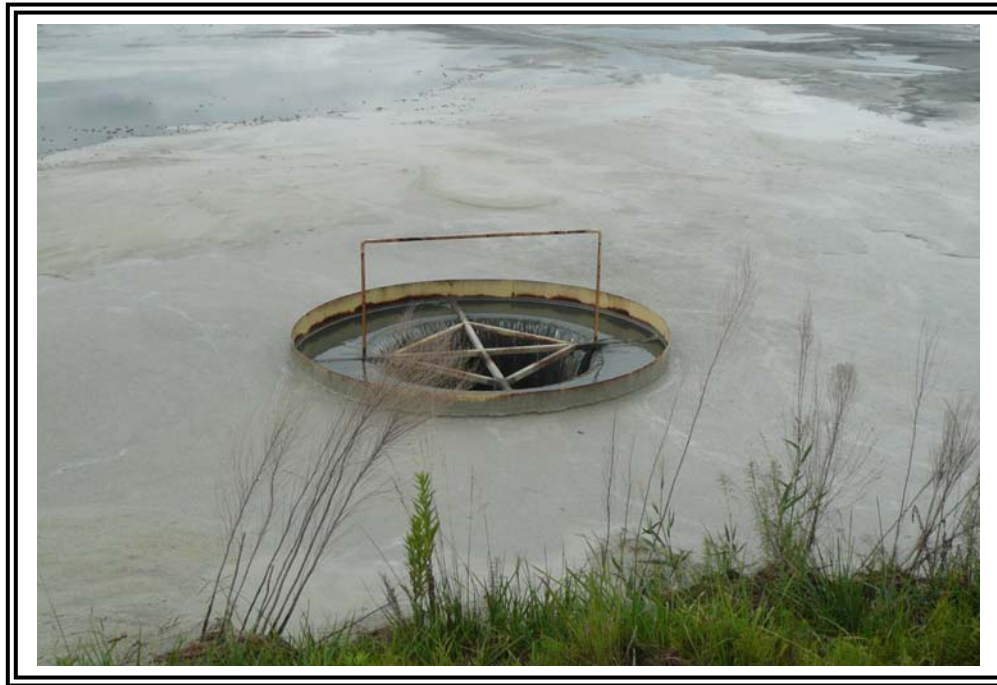
Close up of the outlet control structure in "Pond within a pond".
