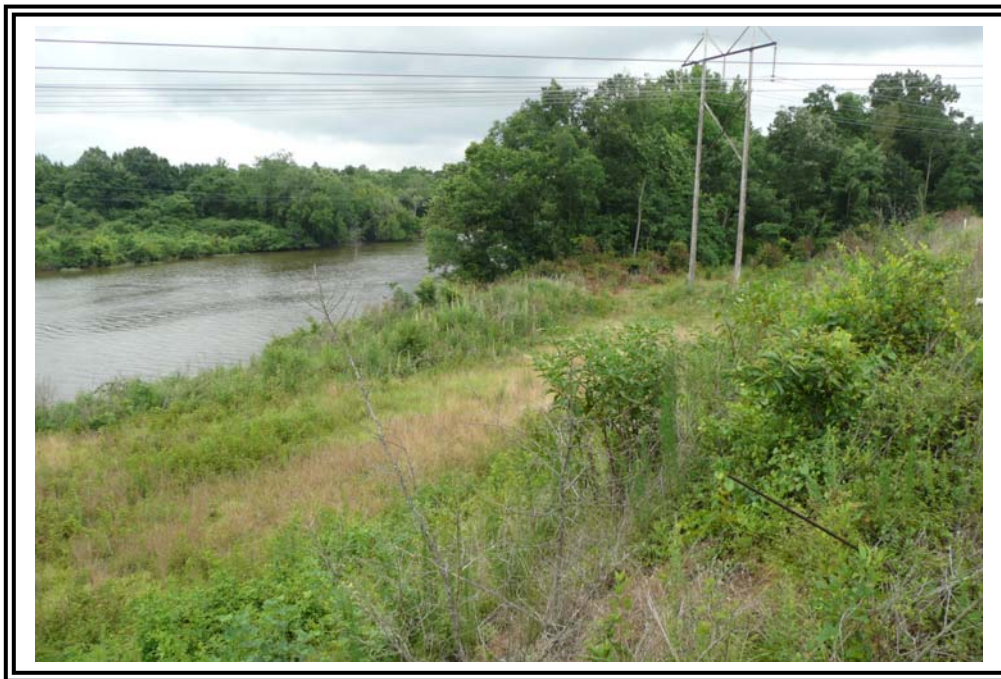
North end of 1963 Ash Pond west dike, looking northwest. Water is Cape Fear River.
