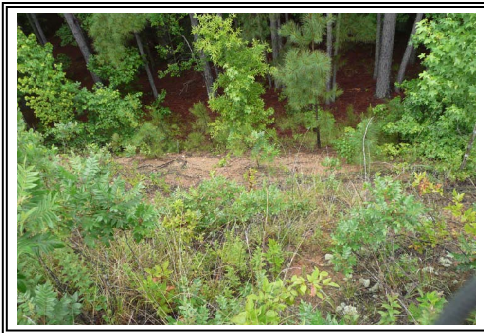
Downstream slope of the 1978 Ash Pond Dike. Note: Rows of trees are immediately beyond the toe.
