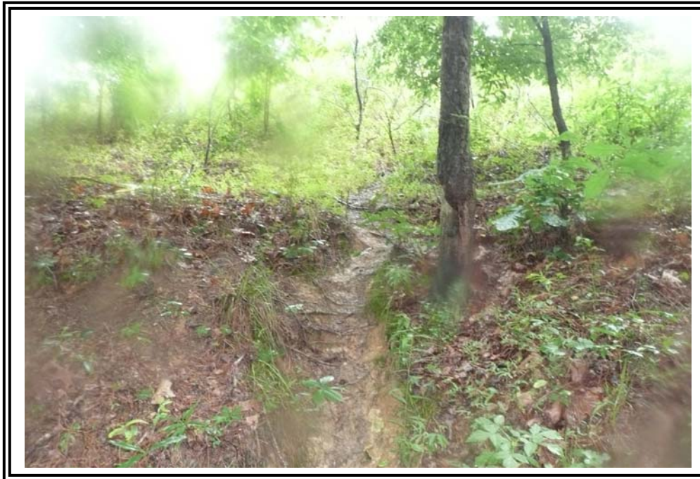
Animal slide (likely beaver or muskrat) on the downstream slope of the 1978 Ash Pond Dike.
