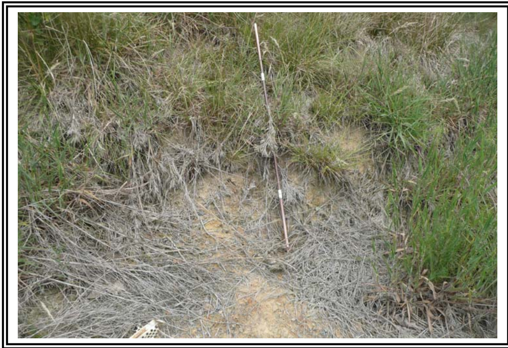
Erosion at the toe of the 1985 Ash Pond West Dike in an area of poor drainage.
