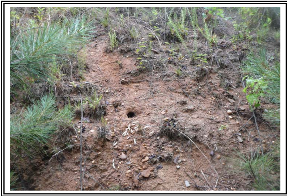
Evidence of animal burrow at the south end of the 1978 Ash Pond Dike.
