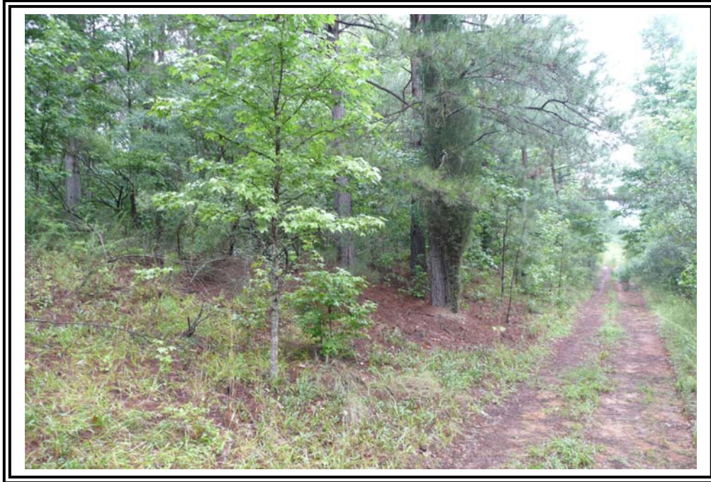
Toe of 1970 Ash Pond east dike, south end looking north. Road is at toe of dike.
