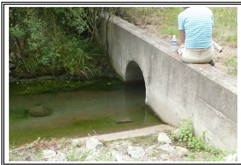
Culvert under the access road at the toe of the 1985 Ash Pond West Dike outlet channel.
