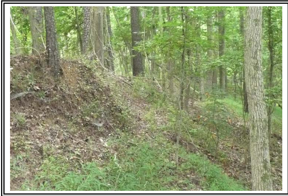
Typical of frequent areas of erosion on the downstream slopes of the 1956 Ash Pond Dikes.
