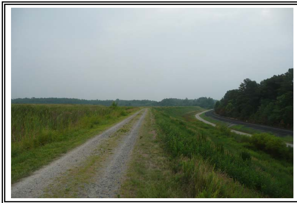
West Dike crest of the 1985 Ash Pond, looking southeast. Note: "Pond within a pond" to the upstream side of the crest. Ash in 1985 Ash Pond approximately at the crest of the dike.
