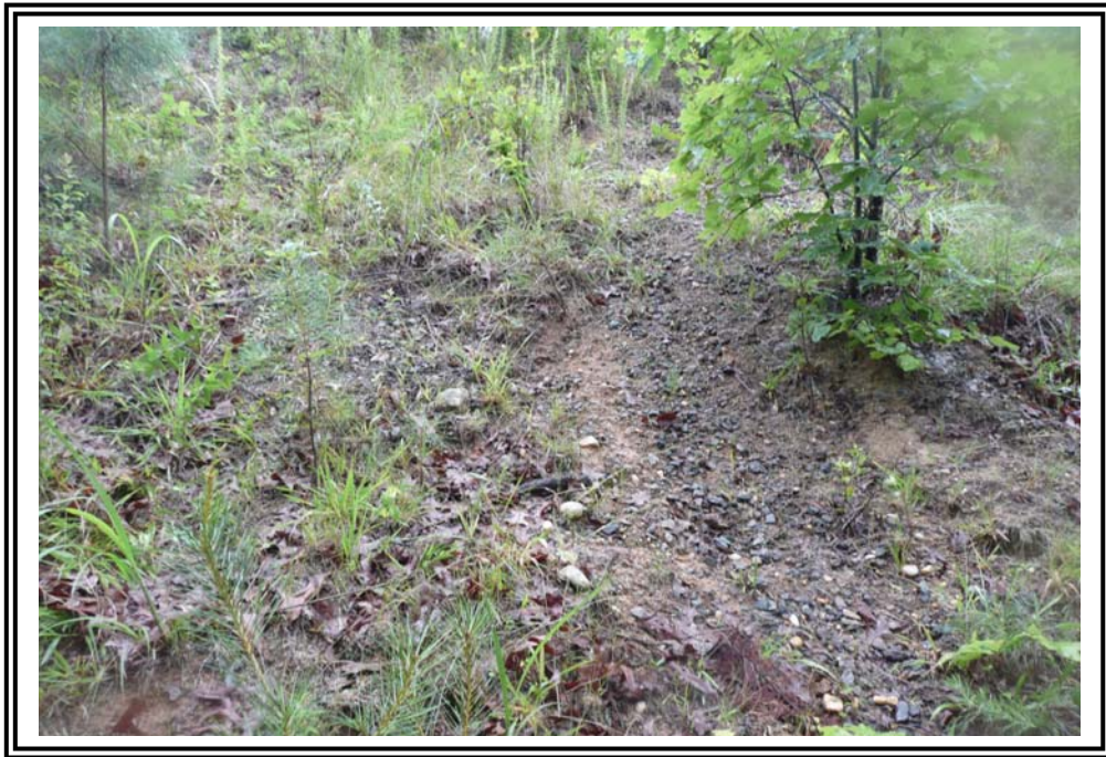
Surface erosion southeast of the downstream slope of the 1978 Ash Pond Dike.
