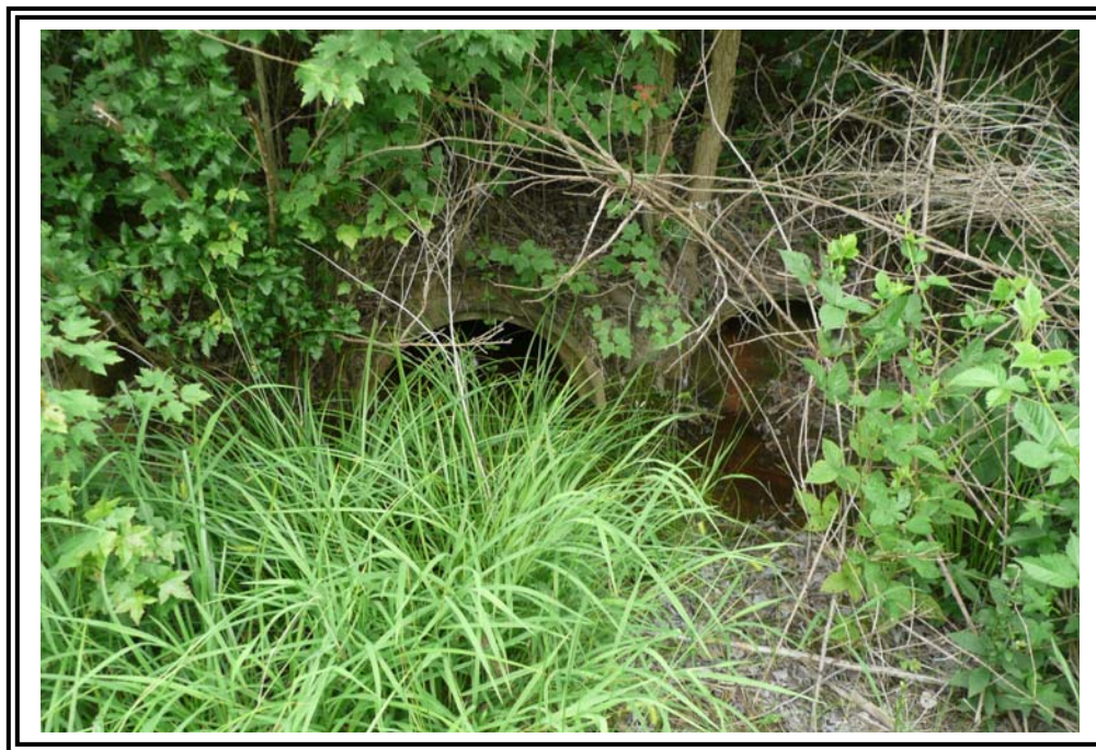
Double culvert under railroad spur for ditch line along West Dike of 1985 Ash Pond.
