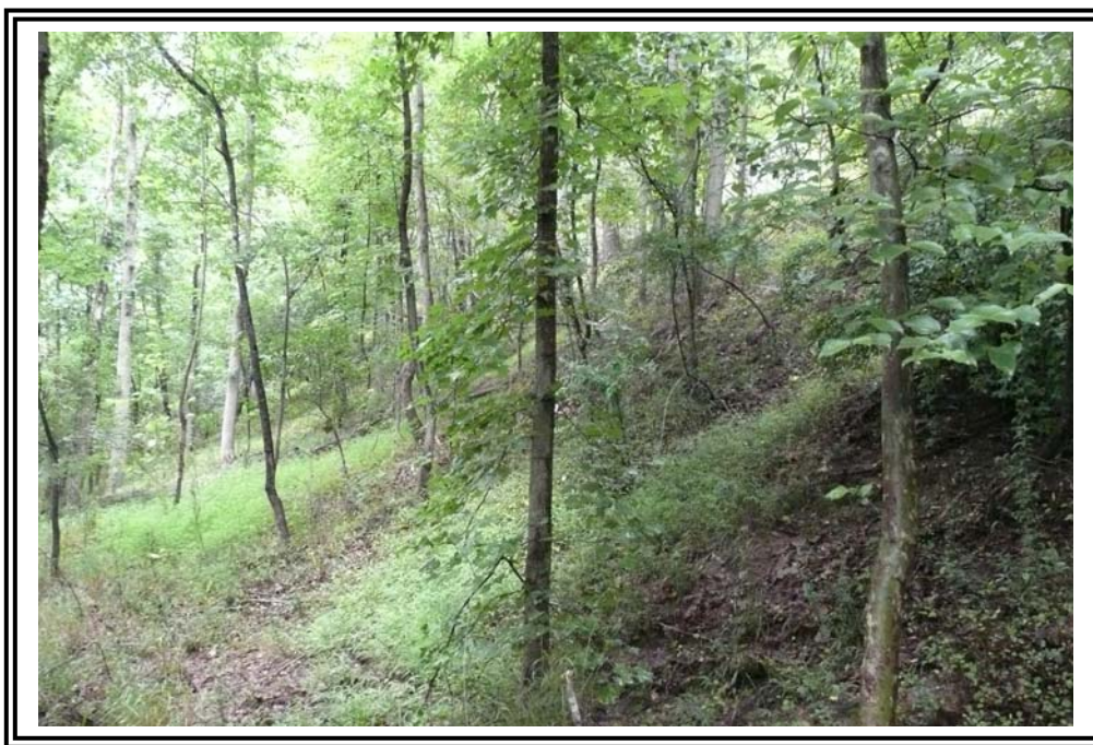
Steepened conditions on 1963 Ash Pond west dike from surface erosion and sloughing.
