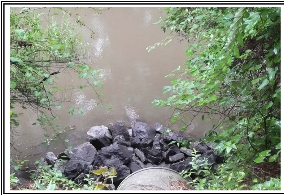
Discharge end of the outlet pipe in the 1978 Ash Pond.
