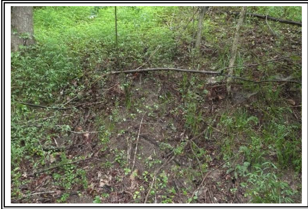
Surface erosion on 1970 Ash Pond west dike downstream slope.
