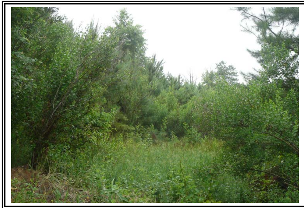
General vegetation conditions on the north end of the 1978 Ash Pond Dike downstream slope.
