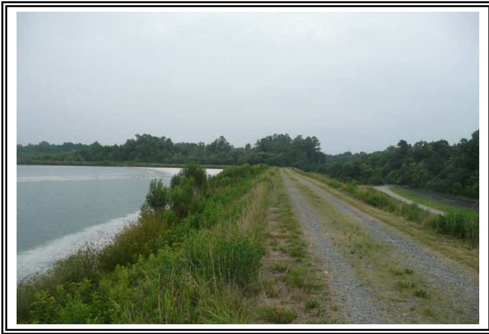
South end of west Dike crest at the 1985 Ash Pond, looking southeast.
