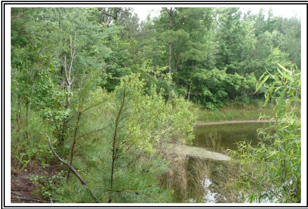
Upstream slope of south dike at 1970 Ash Pond looking southwest from east dike.
