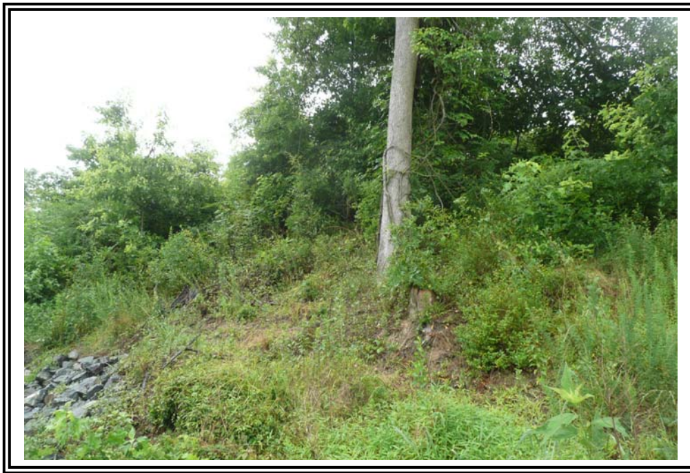
Erosion/surface sloughing around the tree stump on the 1978 Ash Pond Dike.
