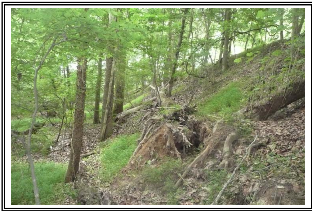
Uprooted tree on the 1956 Ash Pond Dike.
