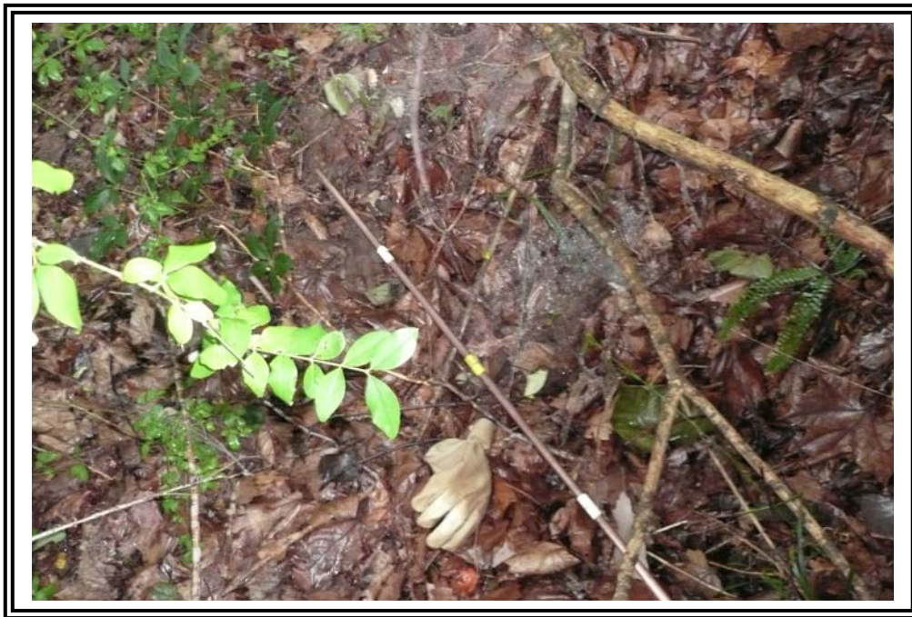
Erosion feature along 1970 Ash Pond west dike toe. Work glove placed below 4' probing rod supported at edge of feature for scale purposes.
