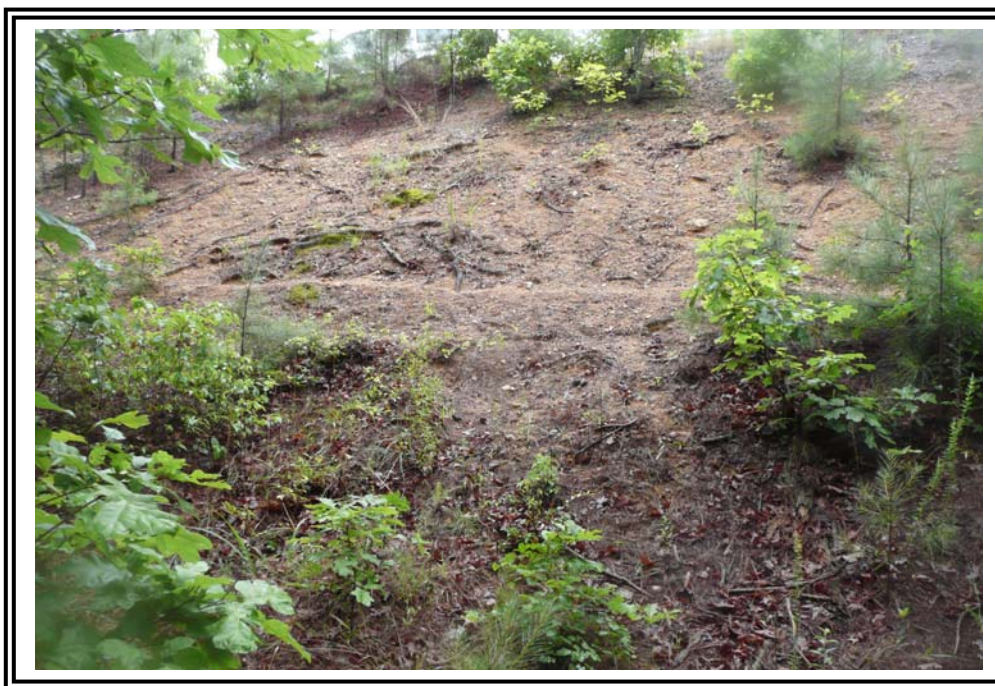
Downstream slope at the south end of the 1978 Ash Pond Dike is devoid of vegetation.
