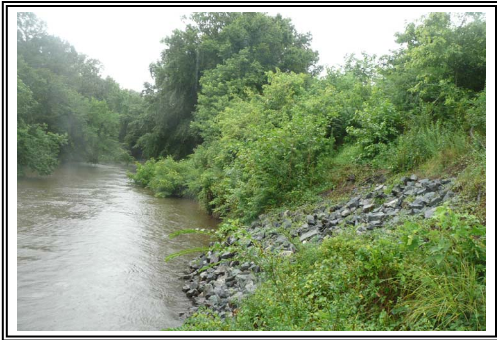
Rip rap fill at the toe of the 1978 Ash Pond Dike along the discharge canal.
