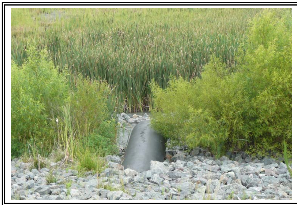
Close up of "Pond within a Pond" outlet.
