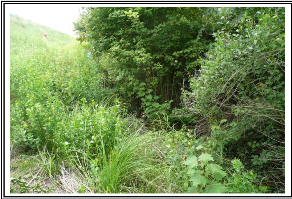
Tree growth at the toe of the 1985 Ash Pond West Dike.
