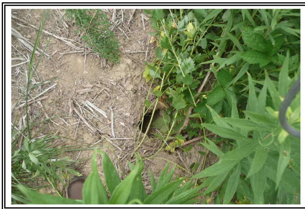
Rodent hole on the 1985 Ash Pond West Dike.
