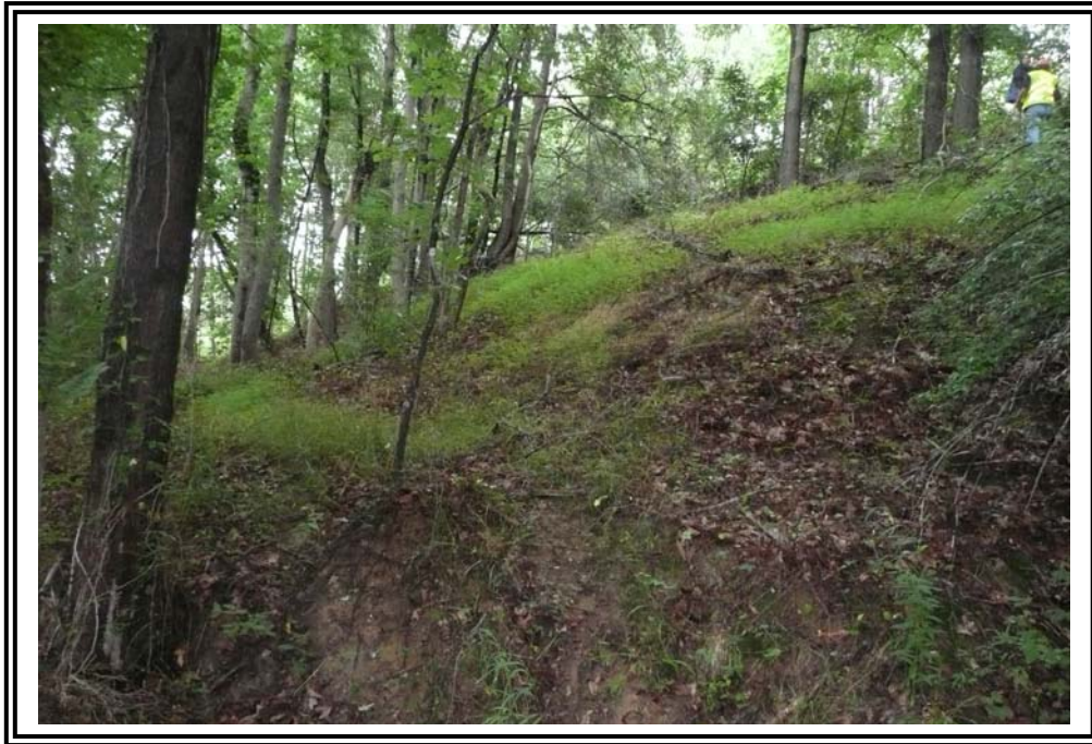
Steepened conditions on 1963 Ash Pond west dike from surface erosion and sloughing.
