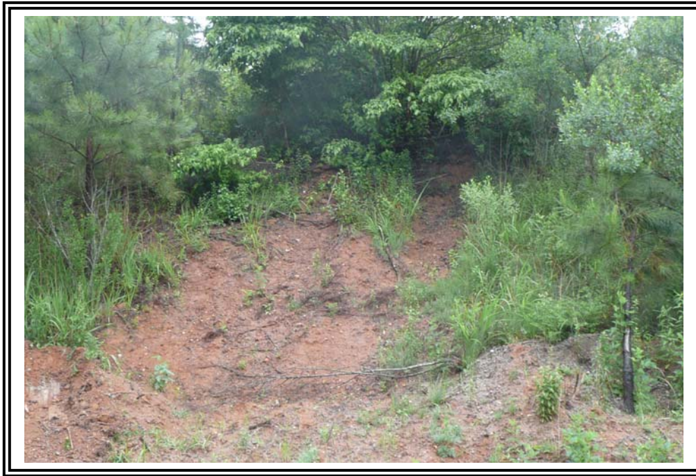
Example of poor vegetative cover, erosion, and probable human activity on the downstream slope of the 1978 Ash Pond Dike.
