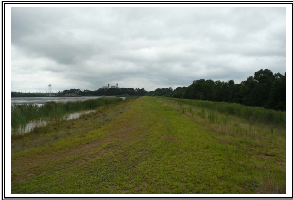
East Dike of "Pond within a Pond" crest. Notice ash stockpiles within the pond.
