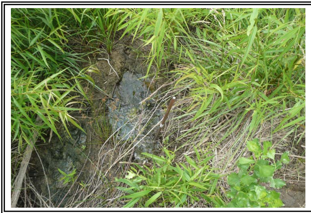
Possible seepage at the toe of the 1985 Ash Pond West Dike.
