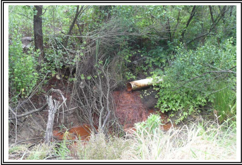
Apparent trench/field drain outlet at north dike toe on 1978 pond adjacent to cooling towers.
