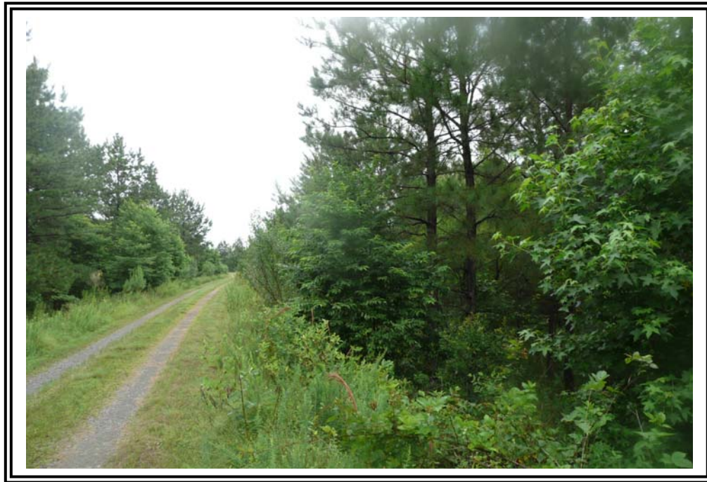
West Dike of 1978 Ash Pond shared with 1963/1970 Ash Ponds. Looking north, trees on either side are growing in deposited ash within the 1970 (left) and 1978 (right) ponds.
