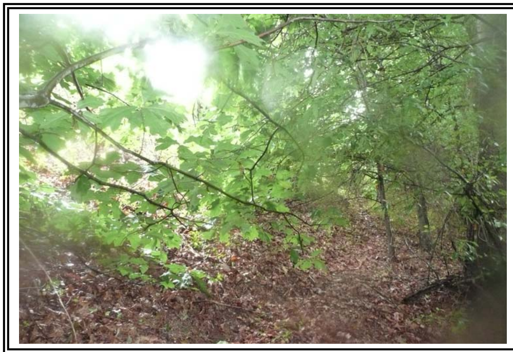
Slough on the downstream slope, east side of the 1978 Ash Pond Dike.
