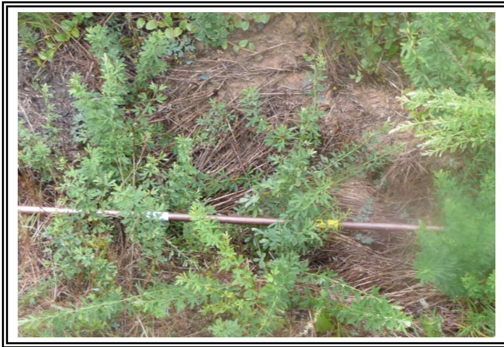
Irregular ground surface on the downstream slope at the east side of the 1978 Ash Pond Dike.
