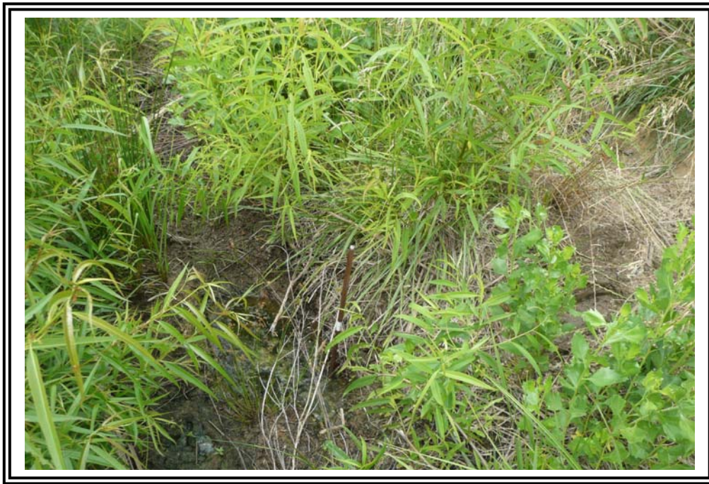
Soft soil at the toe of the 1985 Ash Pond West Dike. Probe pushed into the ground about 2 feet.
