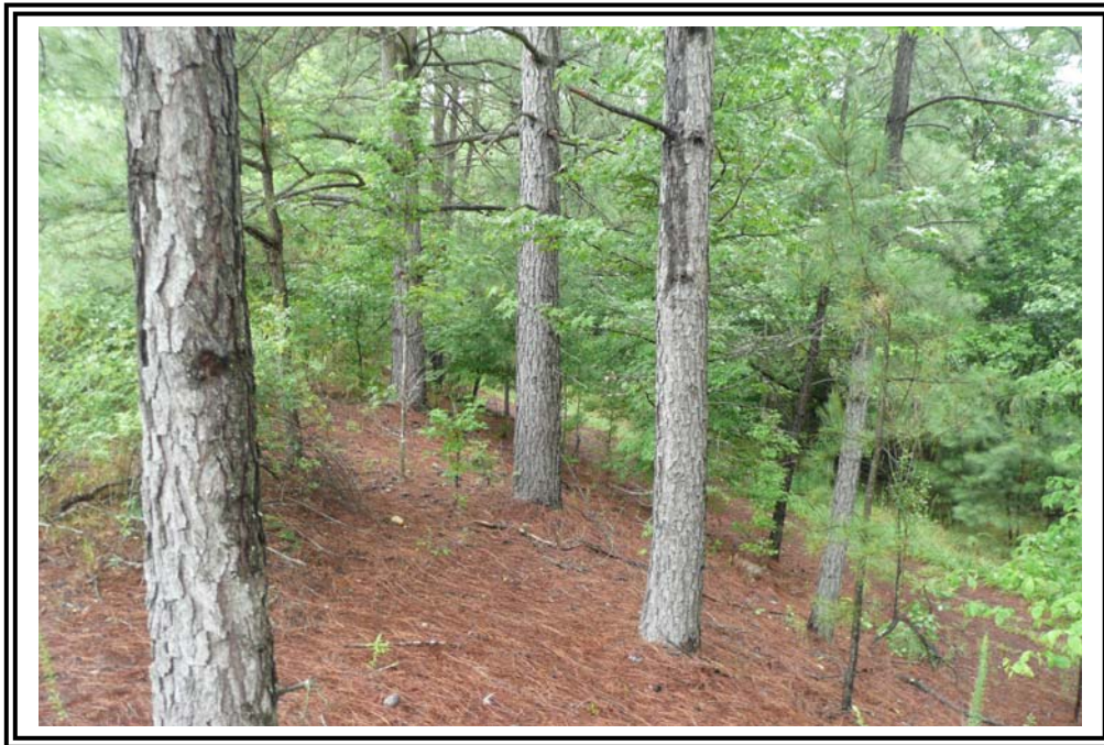
Example of tree coverage on 1978 pond east dike.
