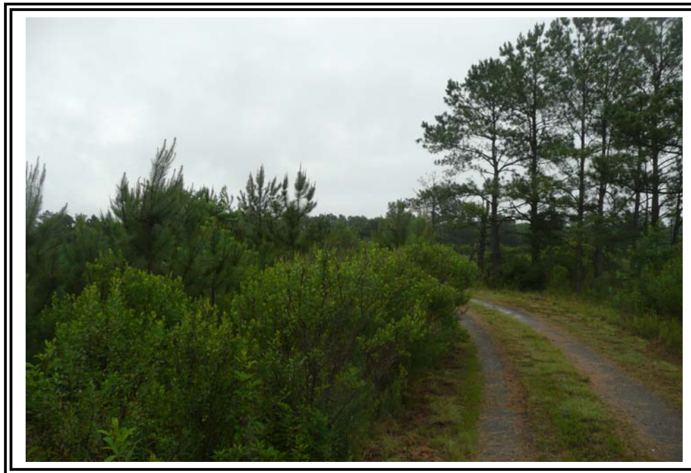
North end of 1978 Ash Pond Dike crest. Brush and small Pine trees are in the left of the photo and are on the downstream slope. Tall Pine trees on the right of the photo are in deposited ash within the pond.
