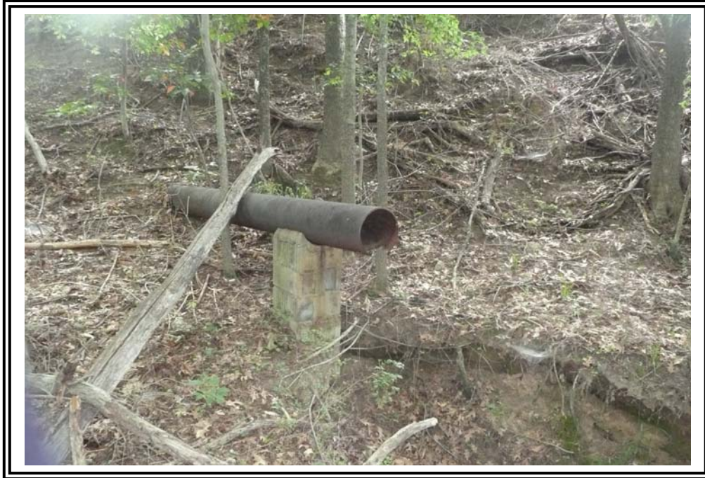
Former outlet pipe from 1956 Ash Pond. Pond no longer contains free water.
