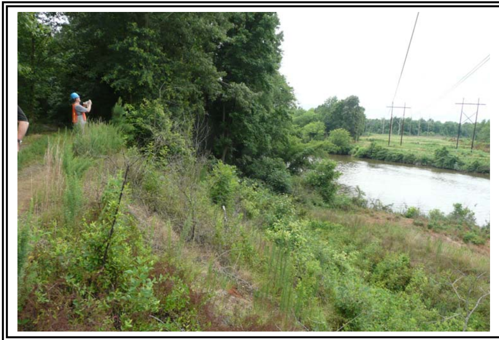
North end of 1963 Ash Pond west dike looking south. This is adjacent to the 1982 slide area. Water in background is the Cape Fear River.
