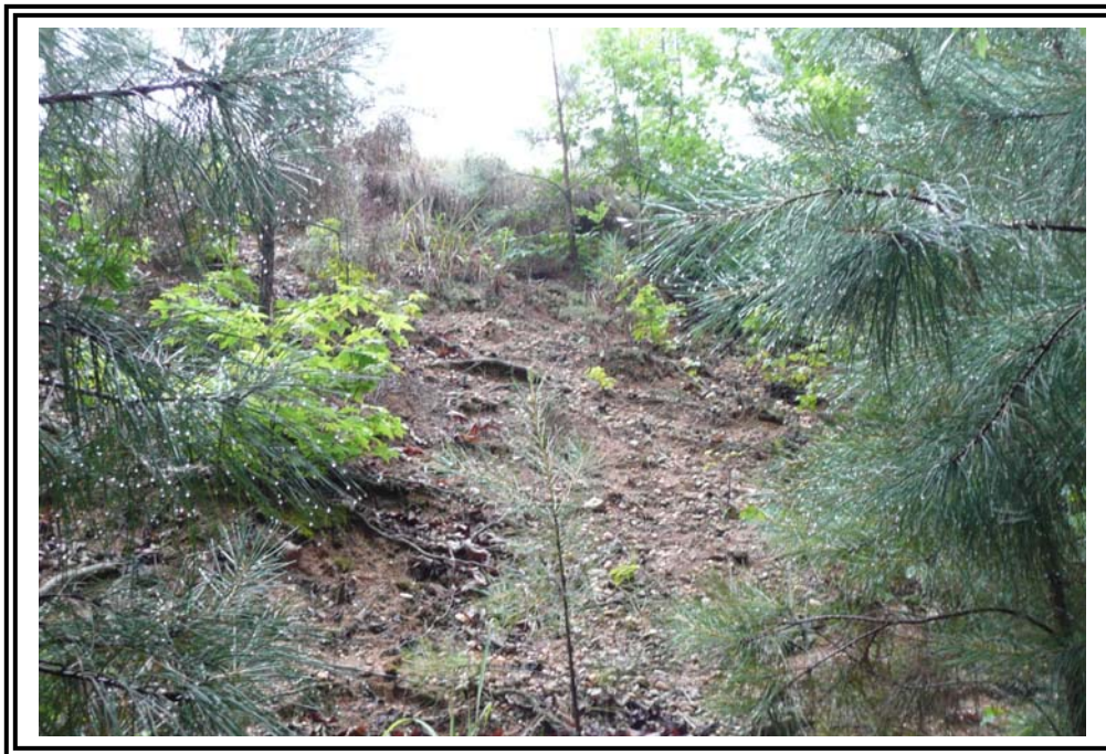
Surface erosion southeast of the downstream slope of the 1978 Ash Pond Dike.
