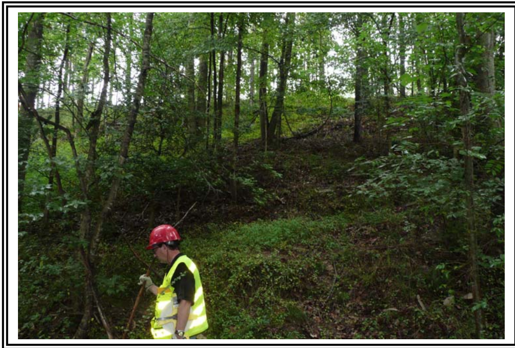
Surface erosion and sloughing on 1970 Ash Pond west dike downstream slope.
