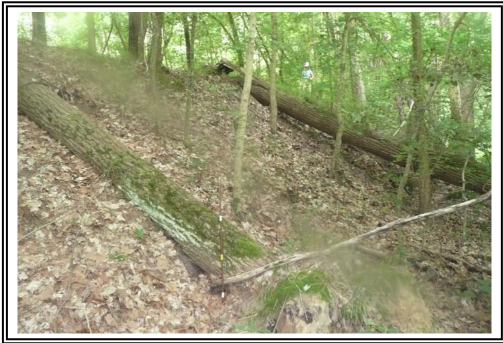
Typical size of fallen trees on the 1956 Ash Pond Dike slopes.
