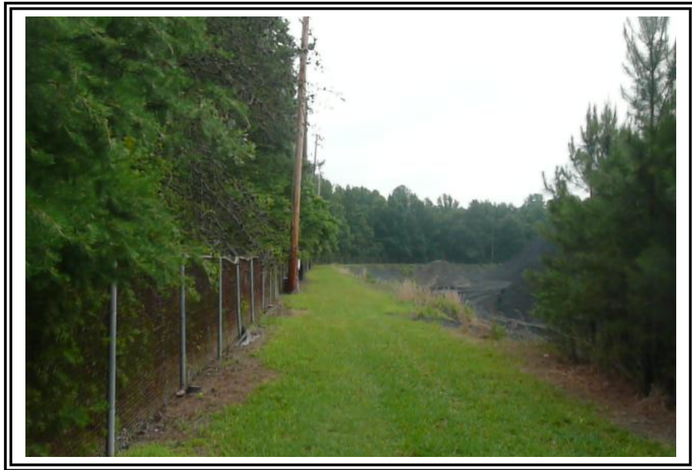
Flood control dike which contained the south side of the 1956 Ash Pond, looking northeast.
