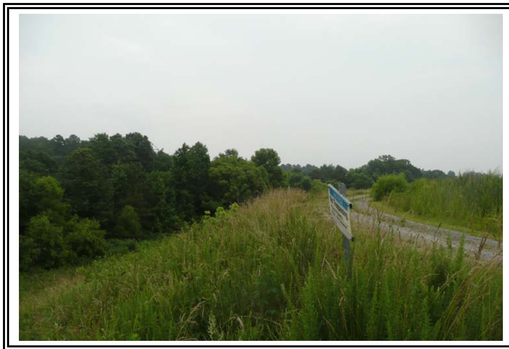
Dike crest at the north corner of the 1985 Ash Pond, near the ash line crossing.
