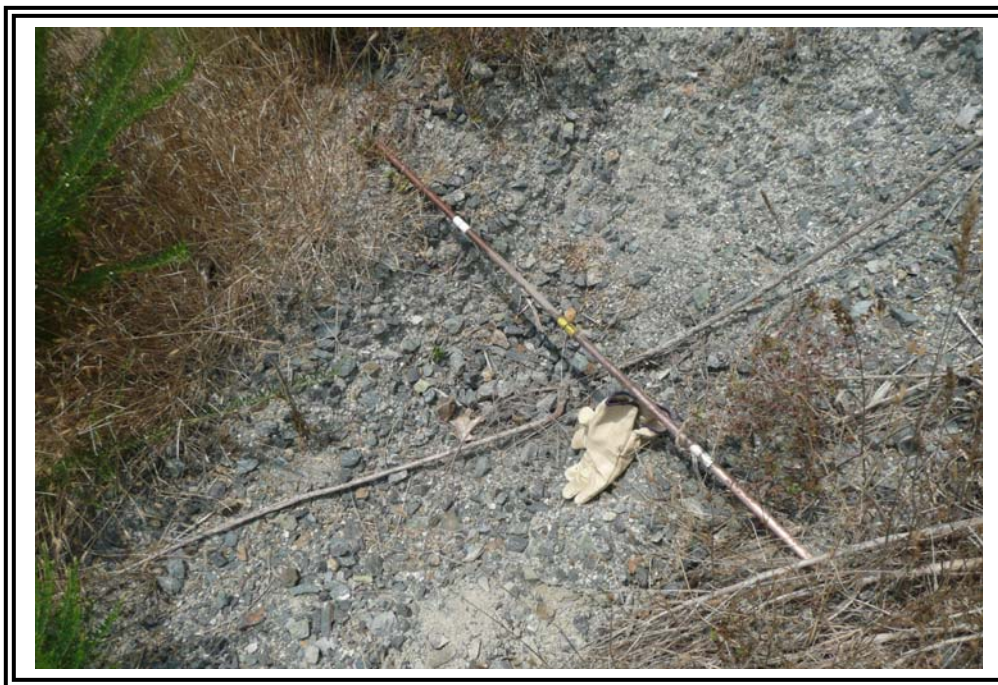
Stone filled erosion and /or abandoned rodent hole on the 1985 Ash Pond West Dike. Progress Energy reports filling rodent holes and erosion features with gravel.
