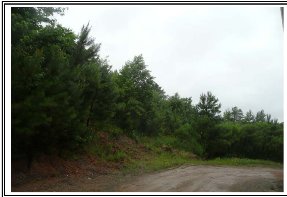
Toe of the 1978 Ash Pond Dike at the north corner, looking west.
