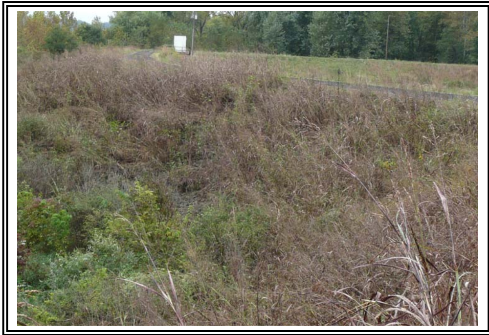
East dike exterior slope, looking south. Note rock slope protection/drain in this area is generally obscured by vegetation.
