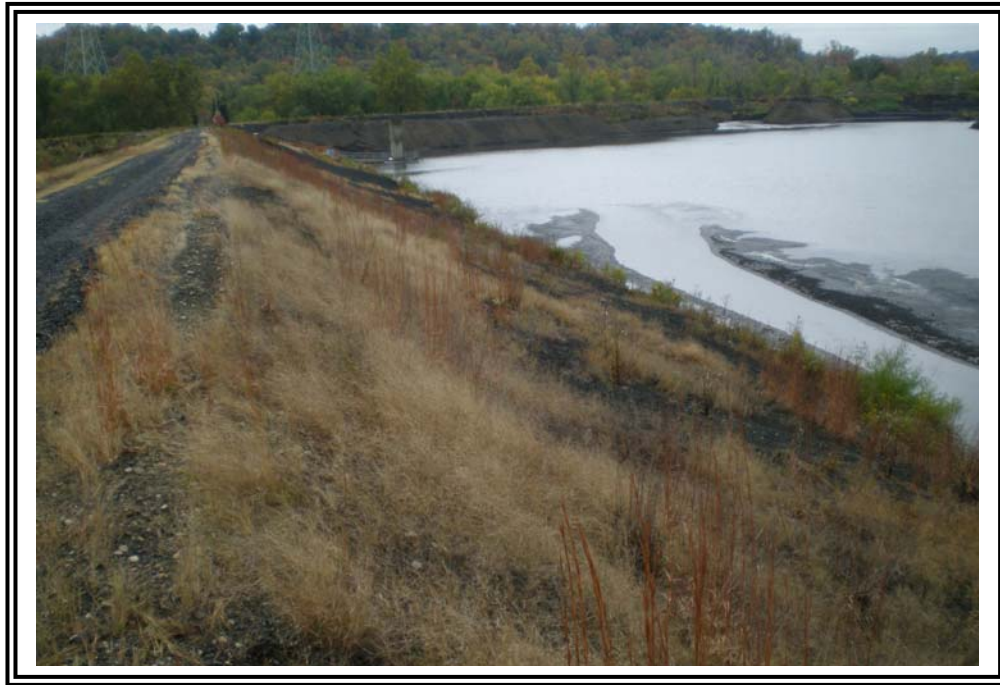
Crest of splitter dike and interior slope of Bottom Ash Pond, looking north.
