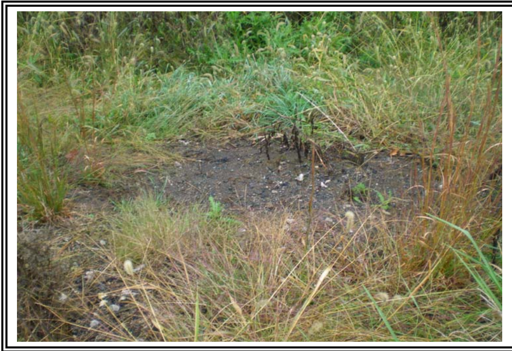
Loss of ground cover and some erosion of exterior slope of south dike.
