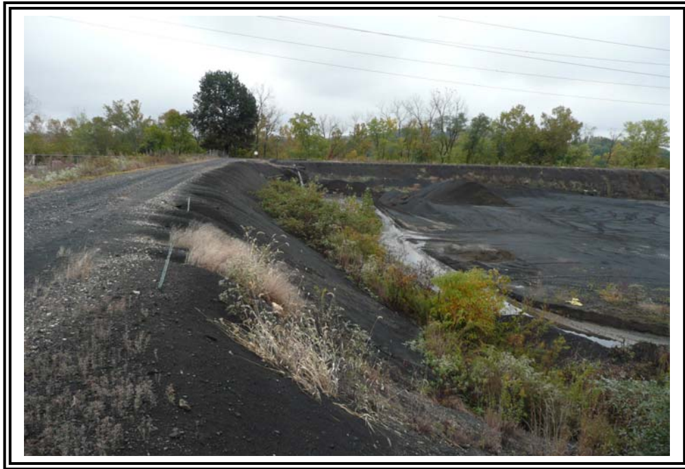
Interior slope and crest of north dike at northeast corner of pond, looking east. This area does not actively impound water.
