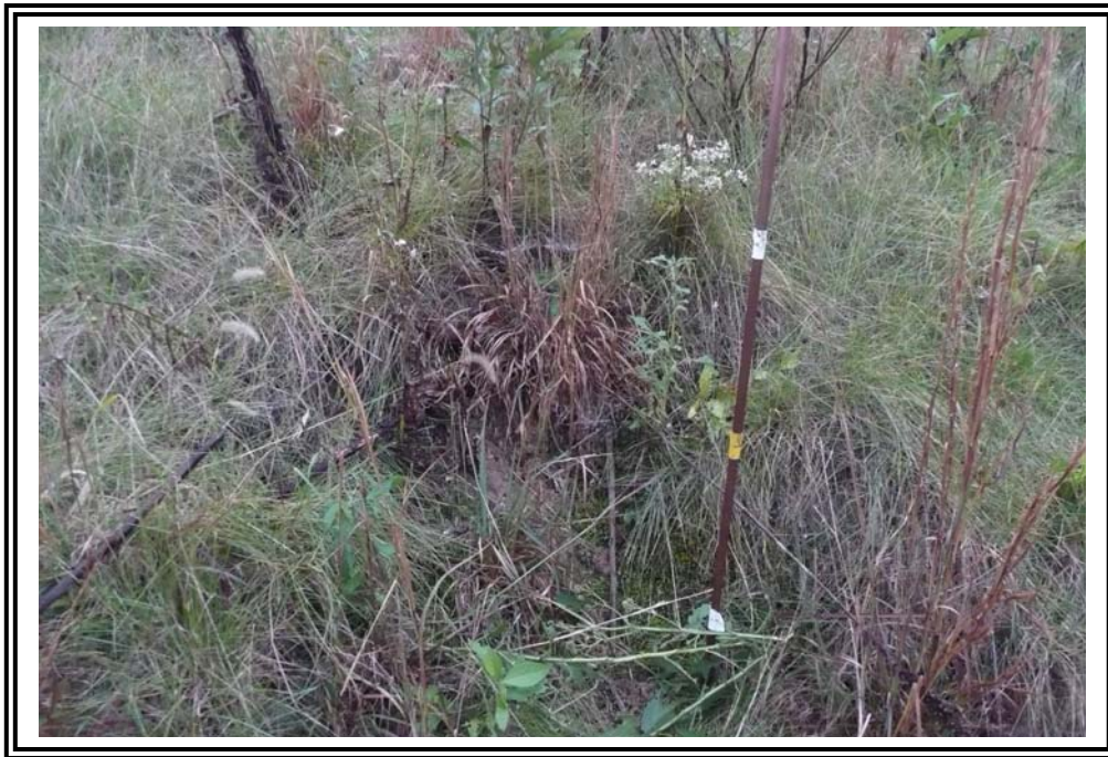
Small scarp/slough in west dike exterior slope.
