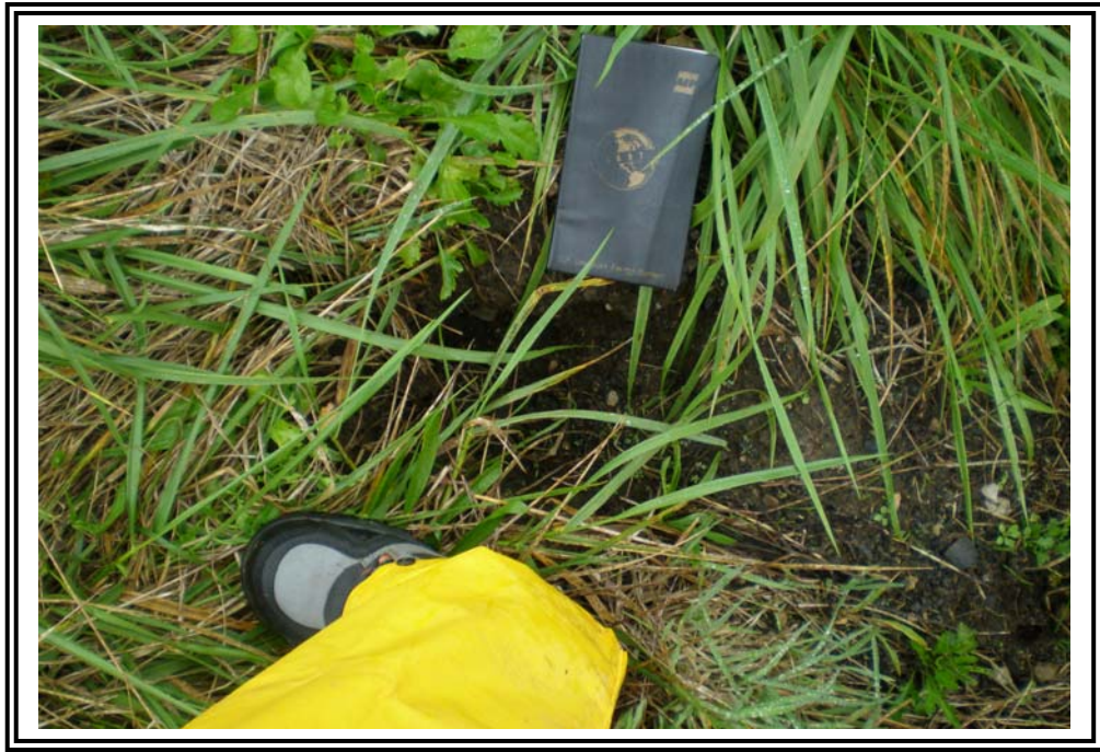
Animal burrow on the exterior slope of the south dike.
