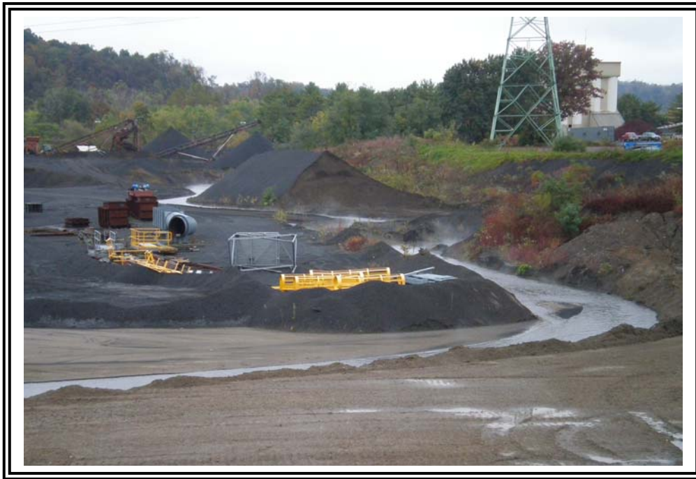
Looking across the northern end of the Bottom Ash Pond at the north dike.
