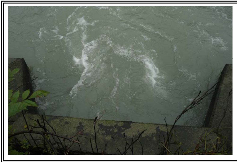
South Fly Ash Pond outlet headwall. Outlet partially submerged during site visit.
