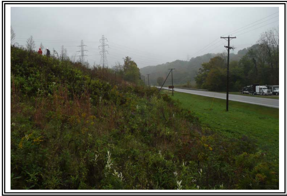
Exterior slope of west dike, looking south. Note moderate to heavy vegetation.
