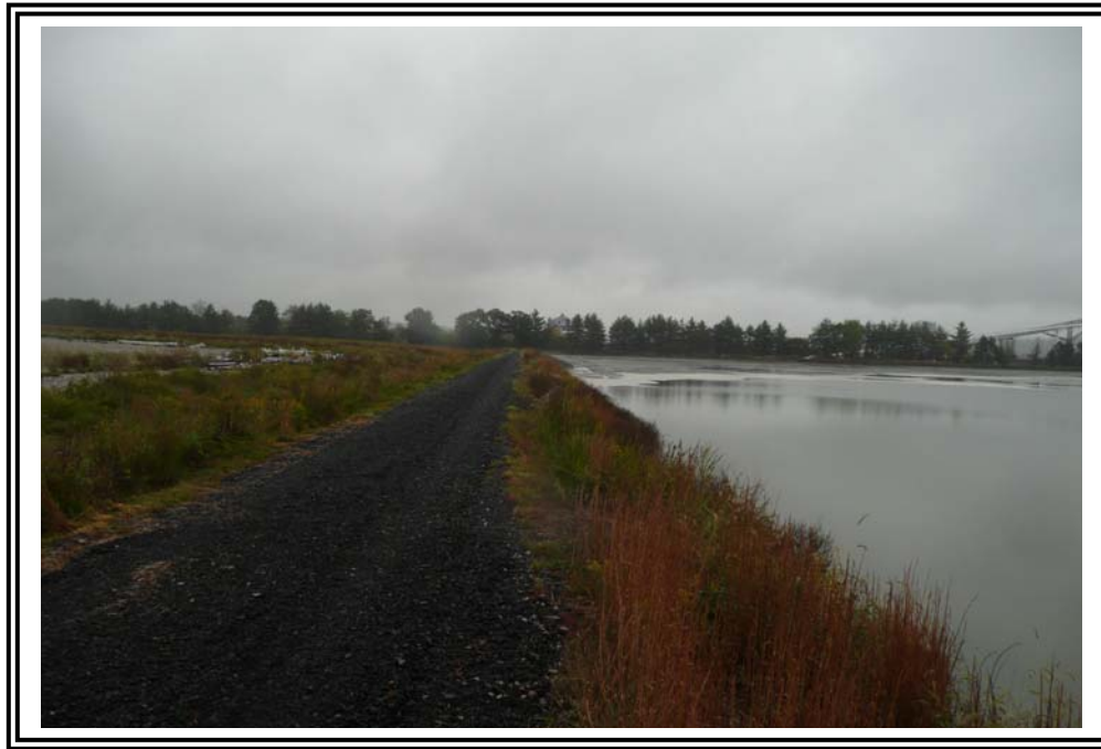
Crest and interior slope of north dike, looking east. Slope is covered with bottom ash and vegetation.
