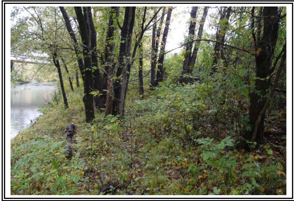
Toe of the exterior slope of south dike, looking west. Note trees and heavy vegetation and Kyger Creek adjacent to the slope toe. There is approximately 12 feet to the creek from the toe.
