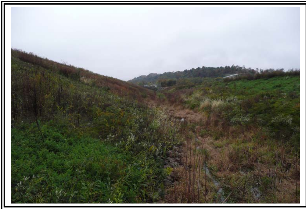
West dike exterior slope, looking south. Standing water observed in rock lined ditch at toe.
