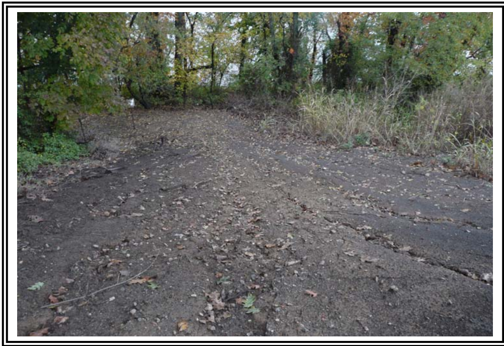
Loss of vegetation cover and erosion rills on exterior slope of the east dike.
