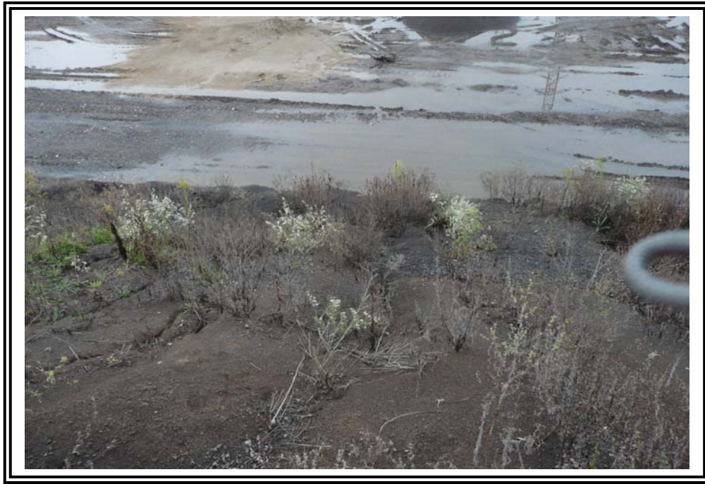
Erosion rills and isolated vegetation cover on interior slope of east dike.
