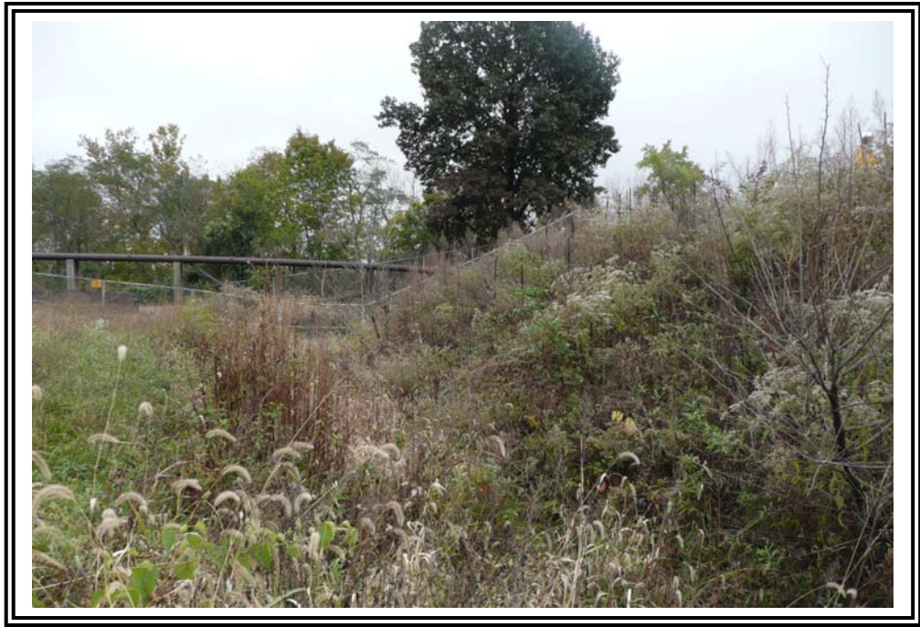
Exterior slope of north dike where sluice pipes enter the pond, looking east. Moderate to heavy woody vegetation was observed.
