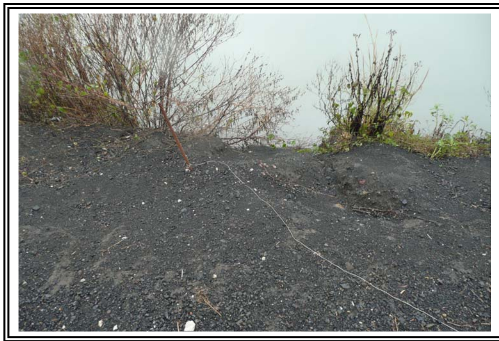
Bottom ash and erosion rills observed in the ash covering the interior slope of the north dike.
