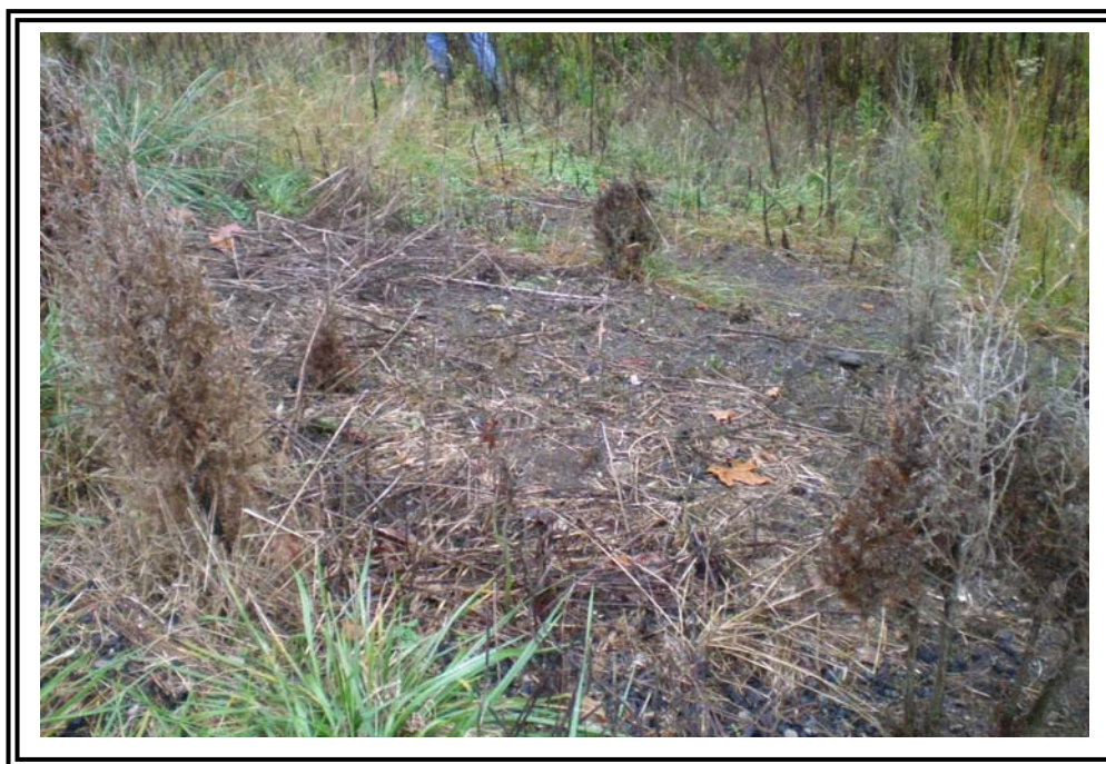
Loss of ground cover and some erosion of exterior slope of south dike.
