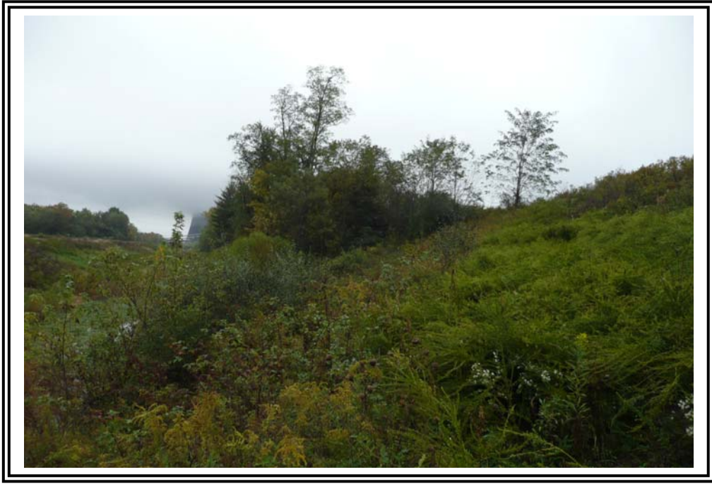
West dike exterior slope, looking north. Note moderate to heavy vegetation.
