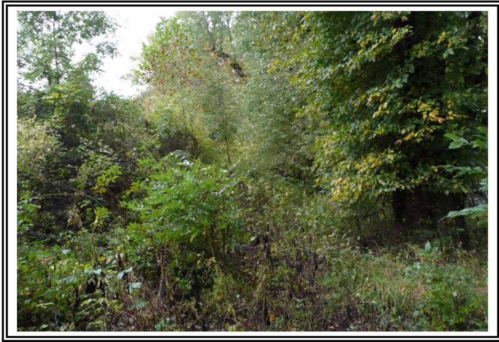
Exterior slope of south dike, looking east. Note heavy brush and vegetation.
