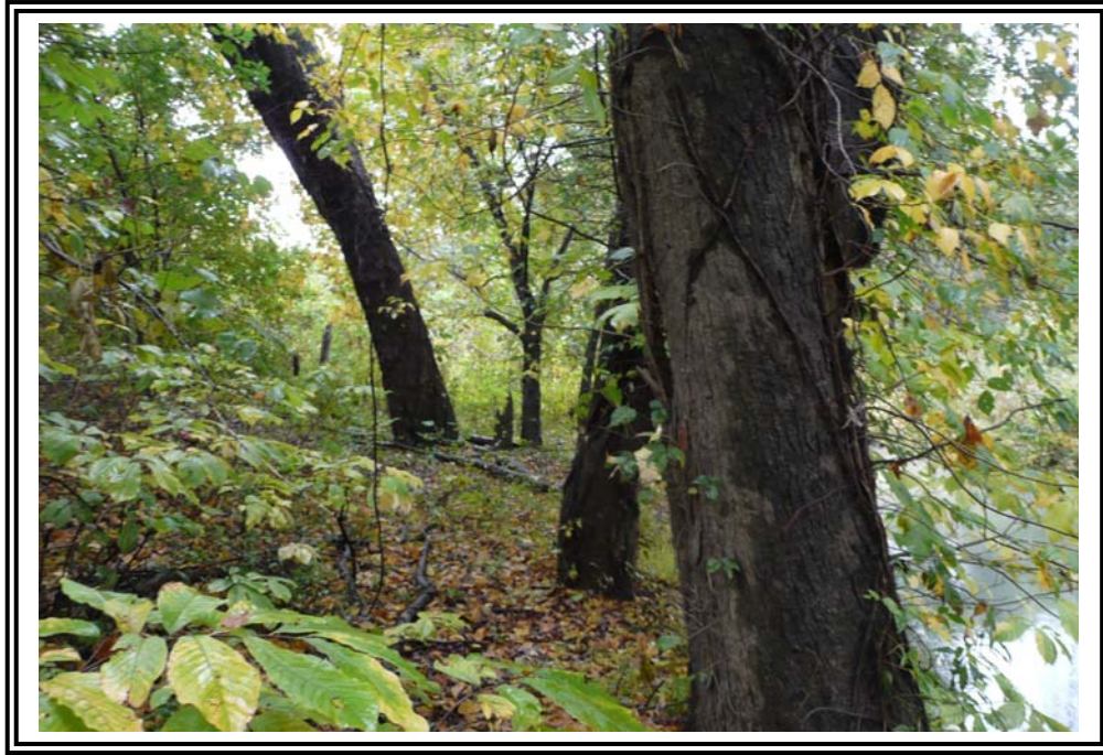
Toe of exterior slope of south dike, facing east. Note curvature of trees towards the dike.
