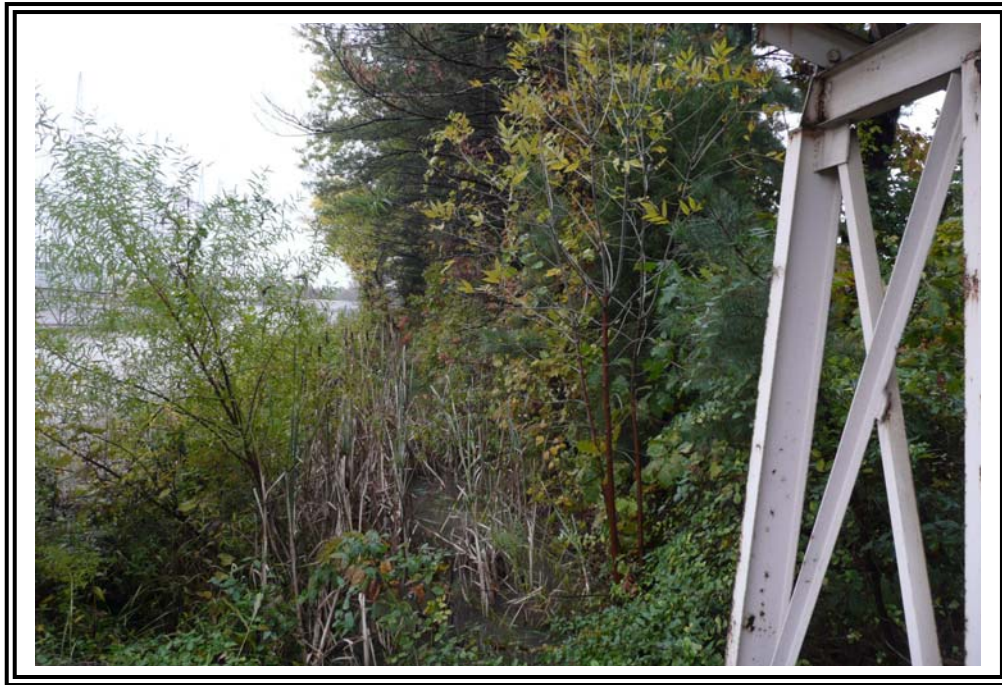
Exterior slope of north dike, looking east. Trees and heavy vegetation was observed.
