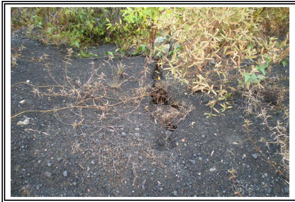
Crest of splitter dike and interior slope of Bottom Ash Pond, looking north.
