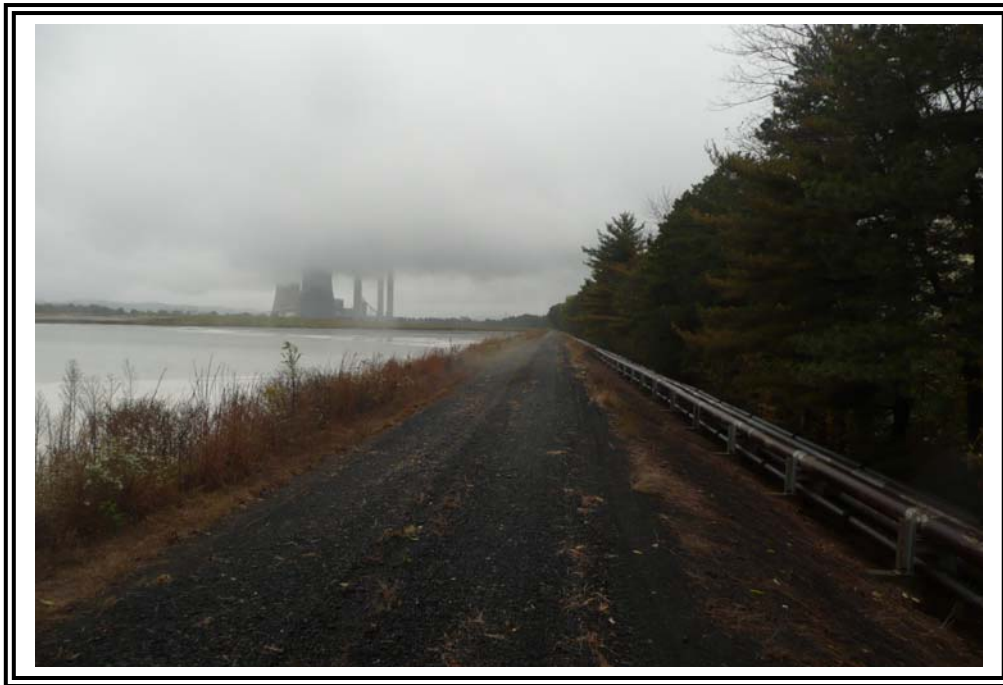
Crest of east dike, facing north. Note pipeline trace and trees on lower portion of the slope.
