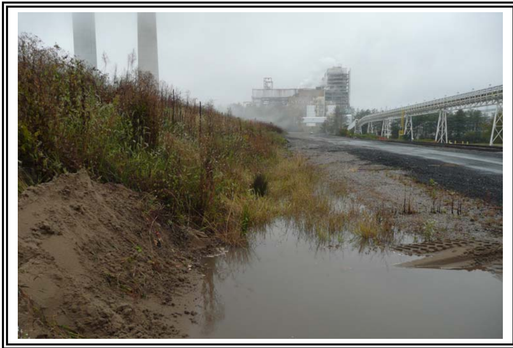
Water pooling in ditch line at toe of south dike. Water is due to recent heavy rainfall and poor drainage.
