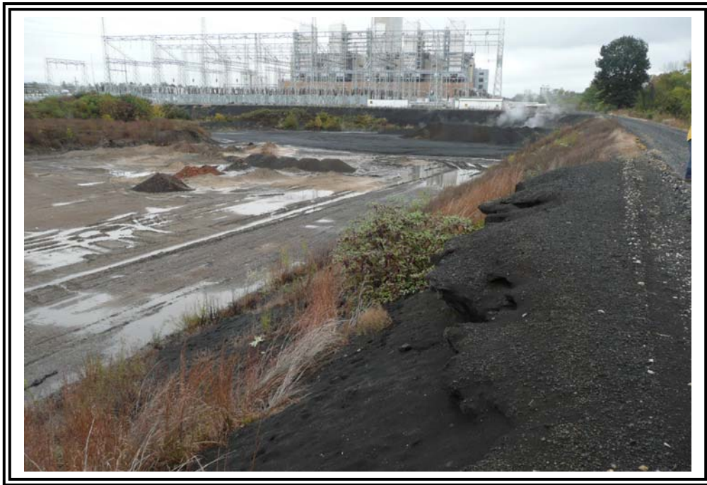
East dike and interior slope, looking north. Note erosion and undercutting of bottom ash material at the crest. Brush vegetation was also evident.
