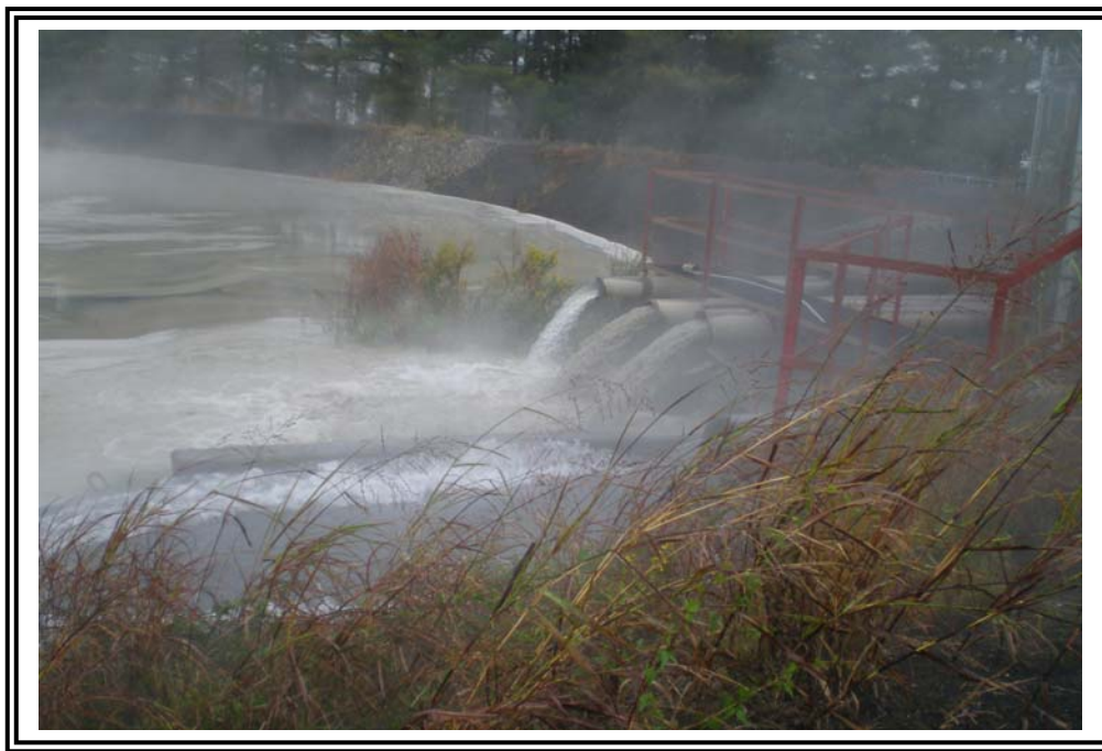
Sluice lines entering the South Fly Ash Pond at the southeast corner of the pond, facing east.
