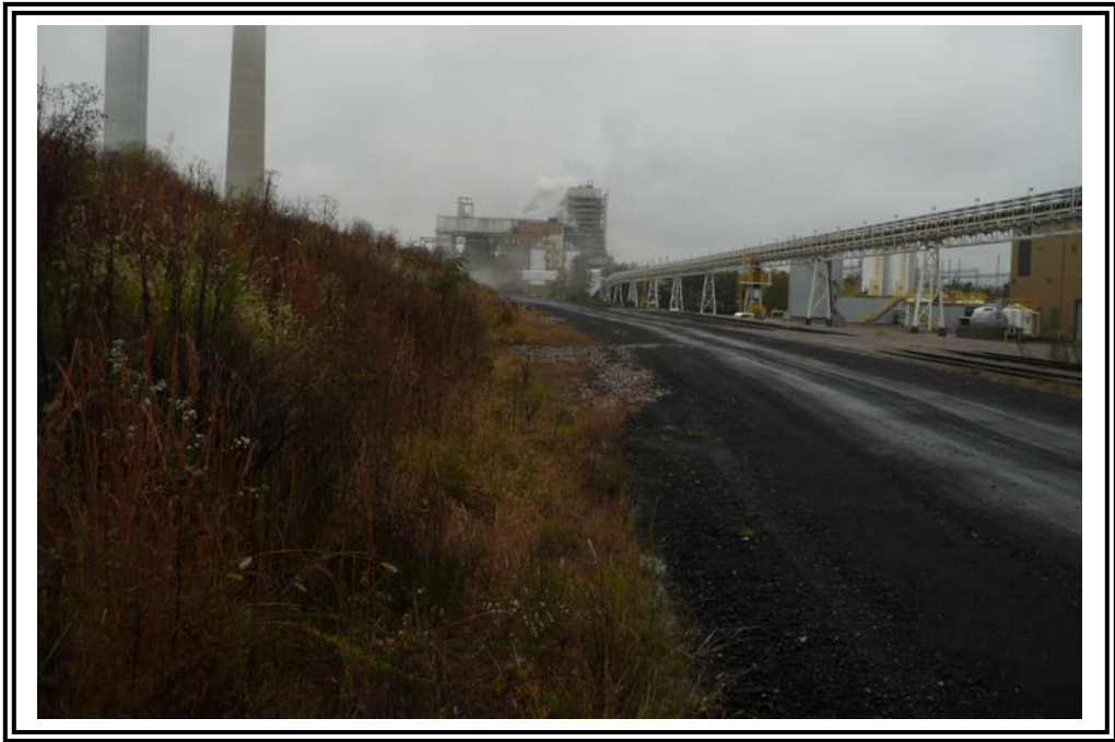
Exterior slope of south dike. Note vegetation on slope and ditch line between the slope toe and access drive.
