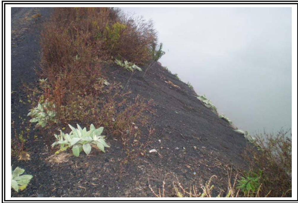
Loss of ground cover and erosion observed on interior slope of west dike.
