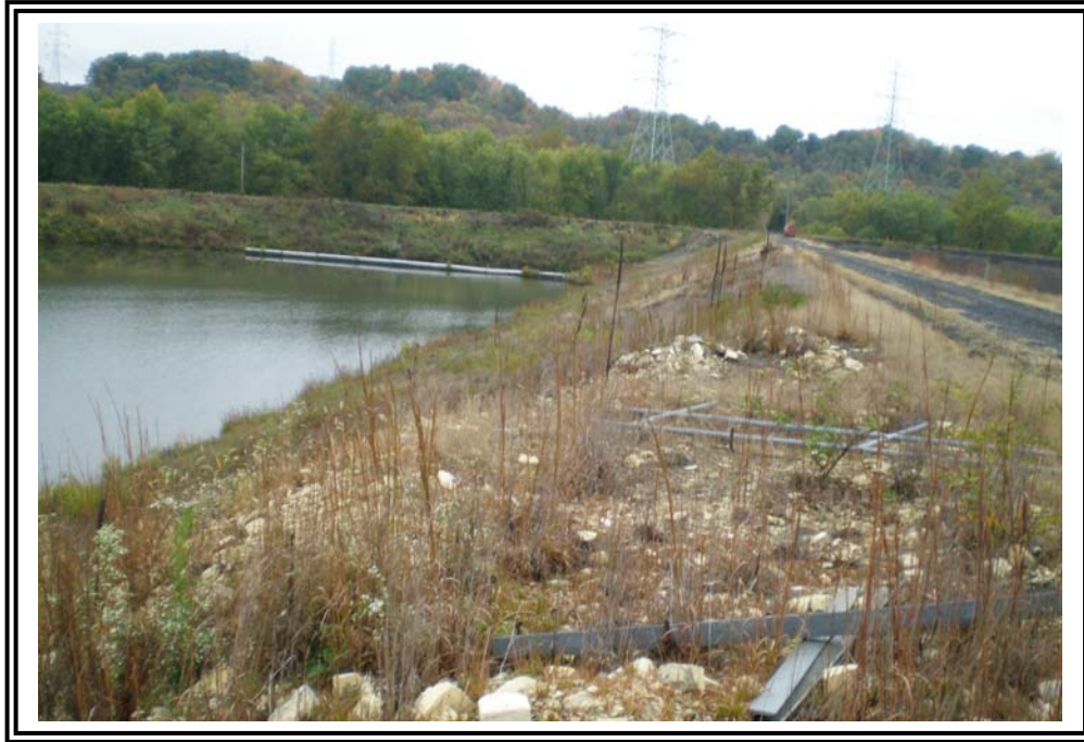
Crest of splitter dike and interior slope of Clearwater Pond, looking north.
