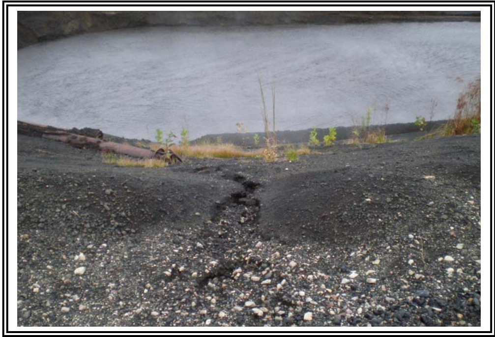
Erosion rills on interior slope of north dike.
