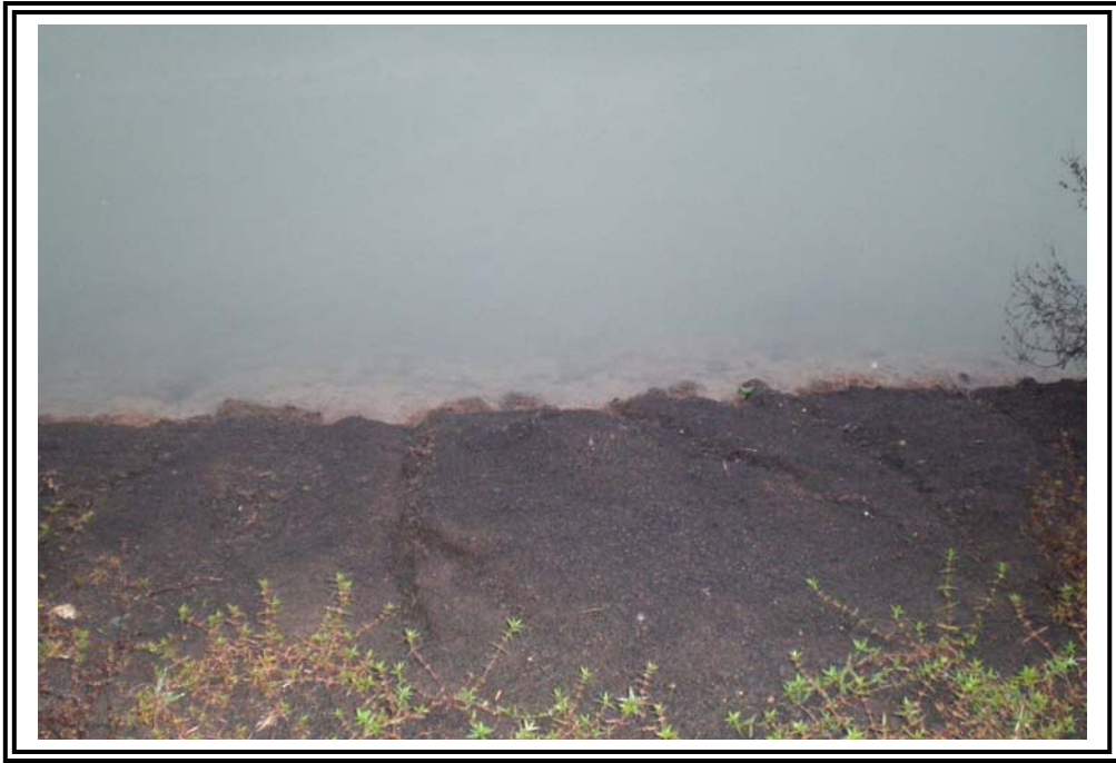
Erosion rills and loss of ground cover on interior slope of west dike.
