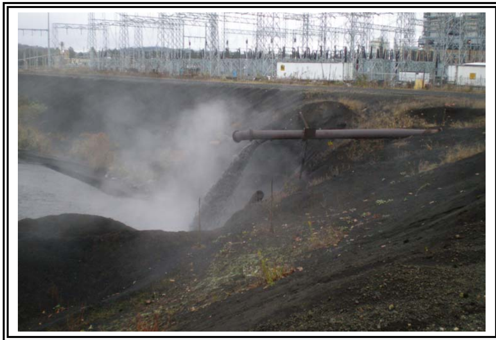
Sluice lines entering the Bottom Ash Pond in the northeast corner of the pond, facing northwest.
