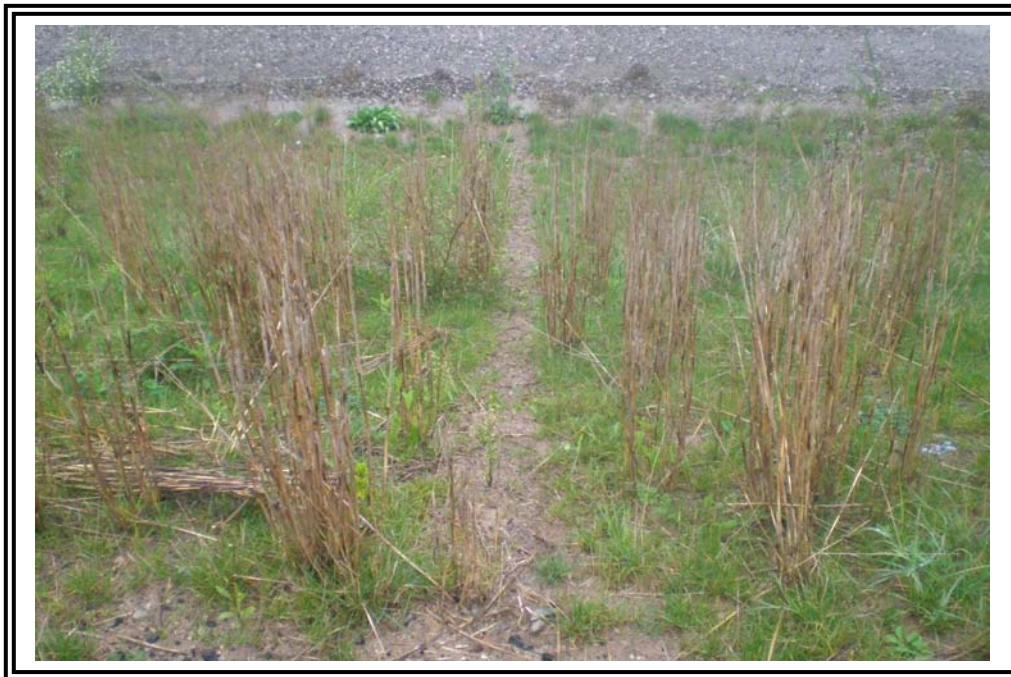
Rill in exterior slope of south dike created by concentrated run-off from the maintenance road along the crest of dike.
