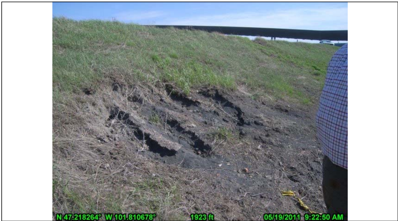
39-Ash Pond Northwest Waterside Embankment Scarping (looking NE)
