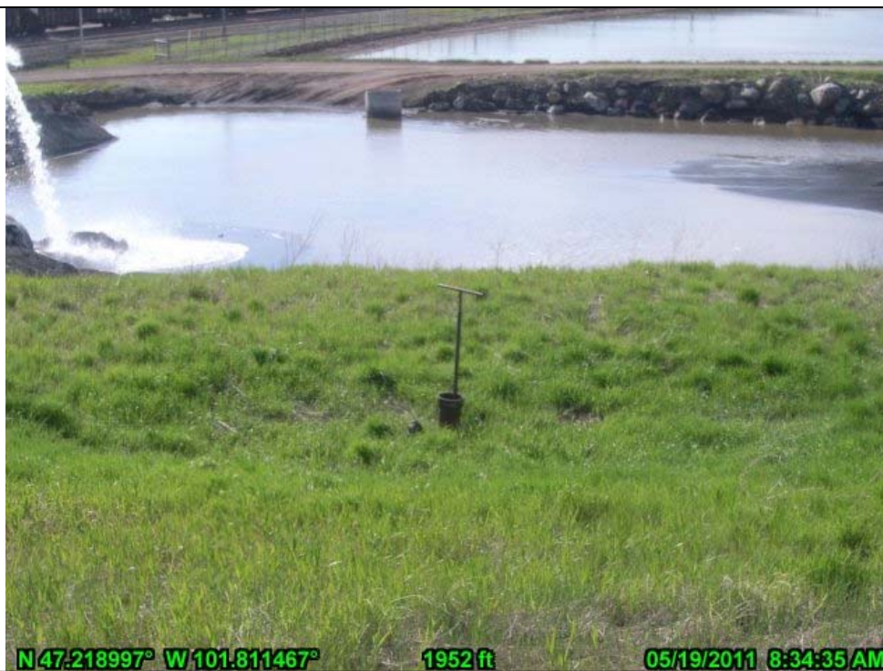
18-Valve Operator between Nelson and Sluice Pond (looking SE)
