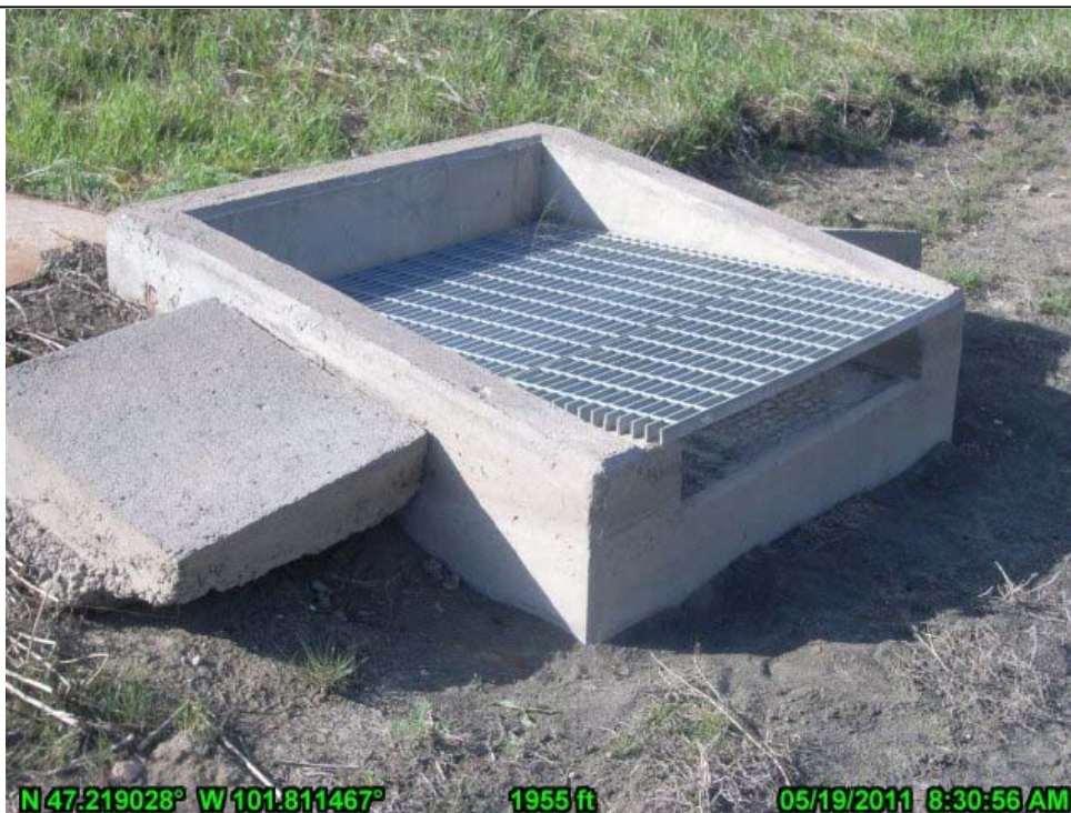
17-Nelson Pond Overflow Inlet Structure
