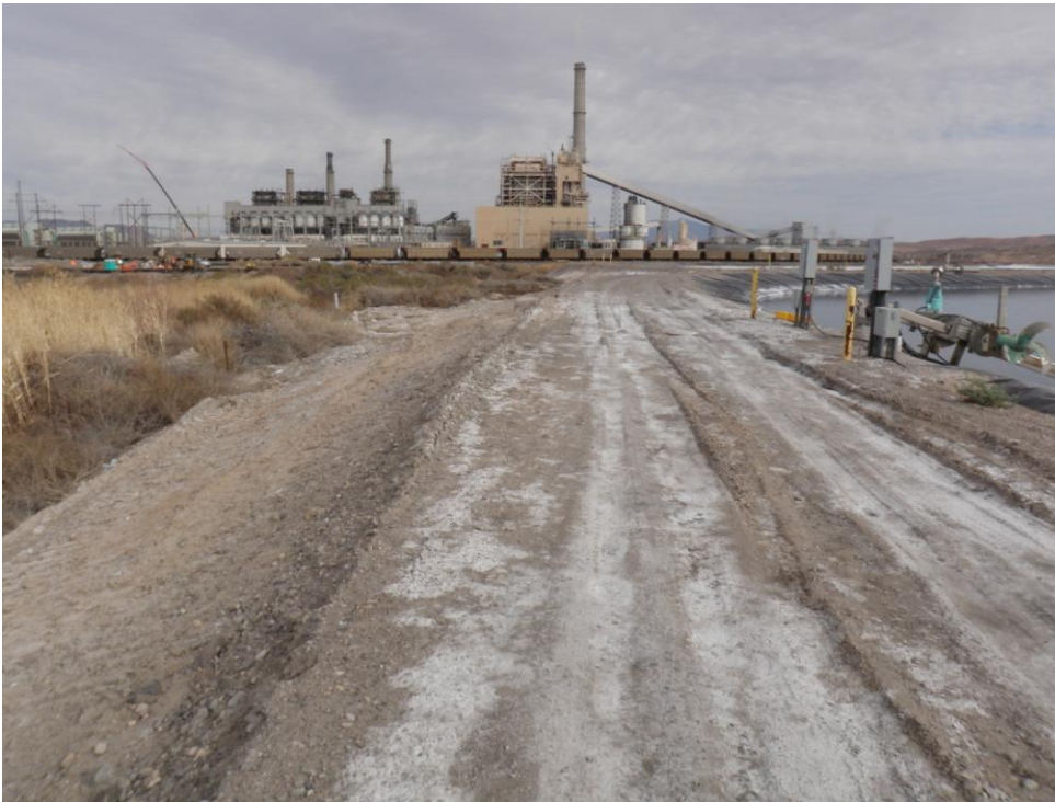
Photo 25: Looking east. Pond E2 north dike near northeast corner. Muddy River on right.
