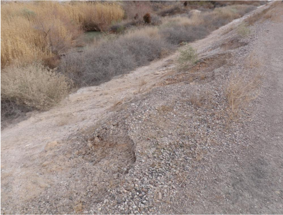
Photo 15: Pond F. Typical erosion of aggregate road base overbuild on top of soil cement slope protection.
