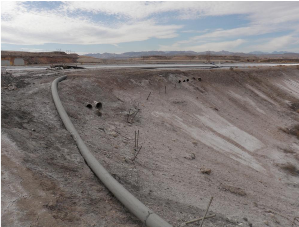
Photo 17: Looking southwest. Abandoned pipe penetrations through north dike of Pond F, near the northeast corner of the Pond.
