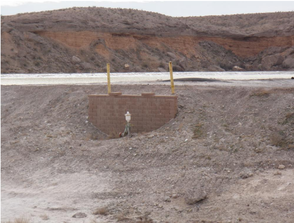
Photo 19: Typical retaining wall to protect air release valve. Looking west at east dike of Pond E2.
