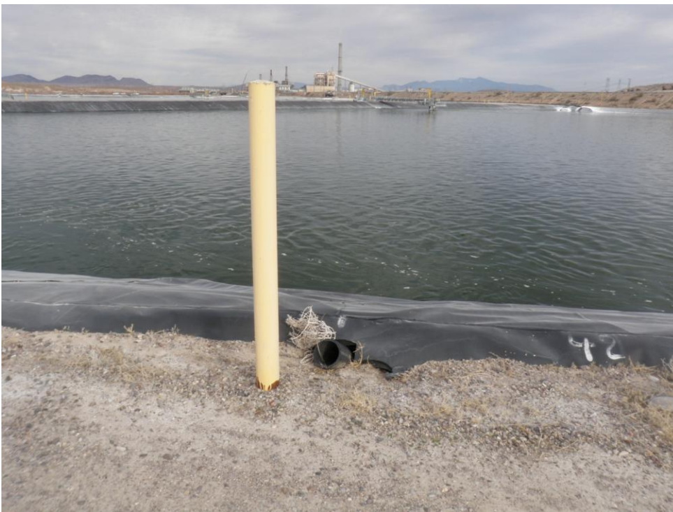
Photo 34: Looking east. Pond B3 west dike. Interstitial drain with HDPE liner in need of repair.
