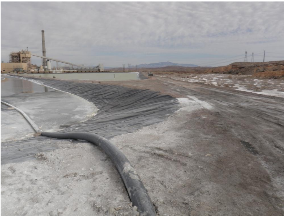
Photo 20: Looking east. Pond E1 in background. Pond E2 with outlet pipe in foreground.
