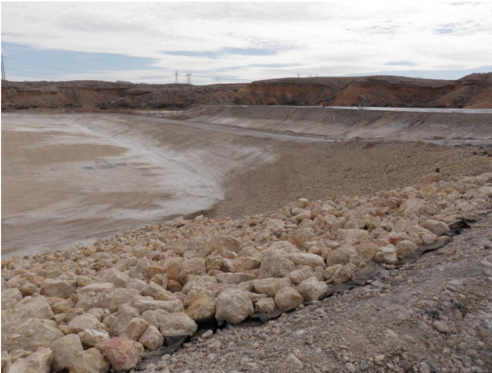
Photo 10: Looking south. Former Pond G. Riprap slope protection and partially removed dike. North dike of Pond E1 at right.
