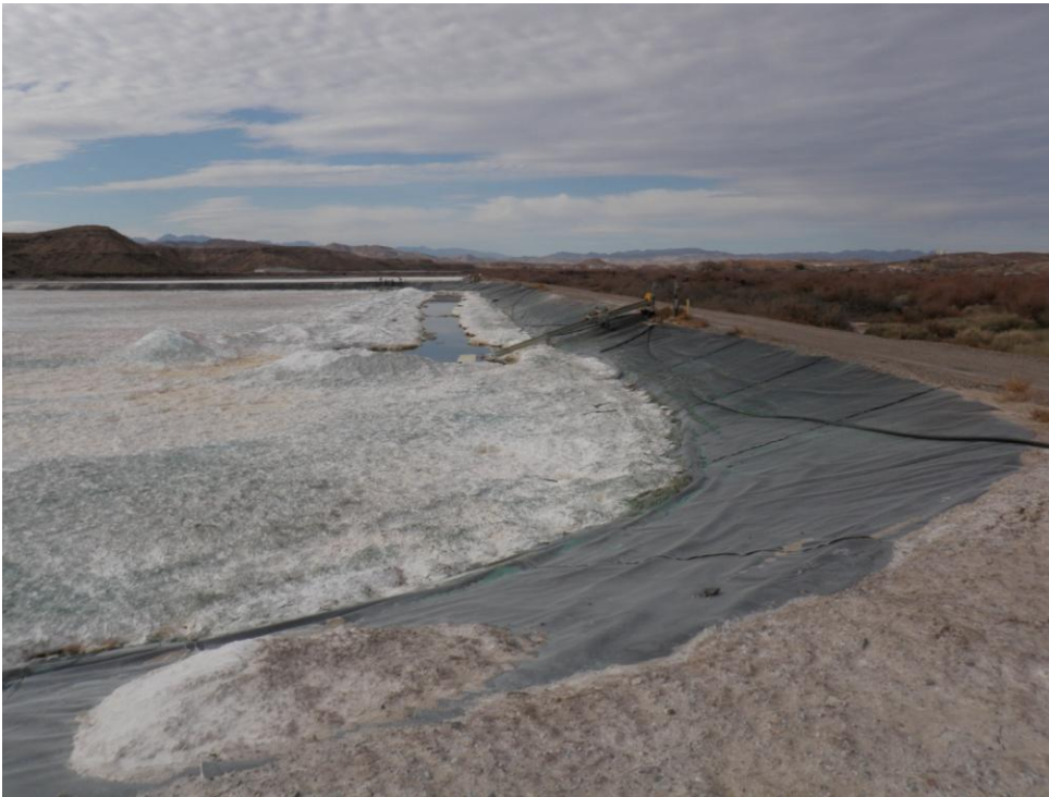
Photo 35: Looking northwest. Pond C1 HDPE liner north dike. Pond C2 in background. Muddy River at right.
