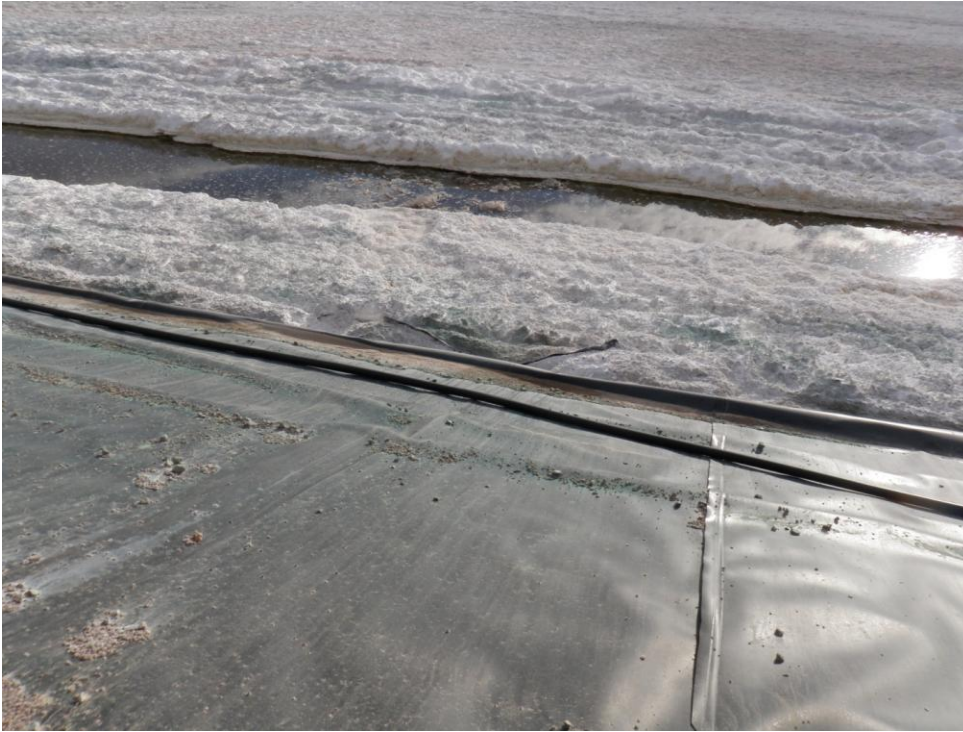
Photo 41: Bulge in HDPE liner on Pond C1 north dike.
