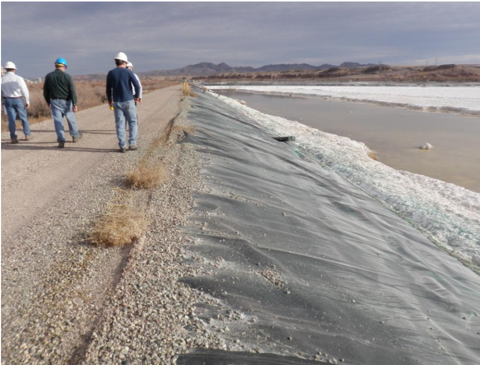
Photo 39: Looking southeast. Pond C2 north dike. HDPE with abandoned penetration.
