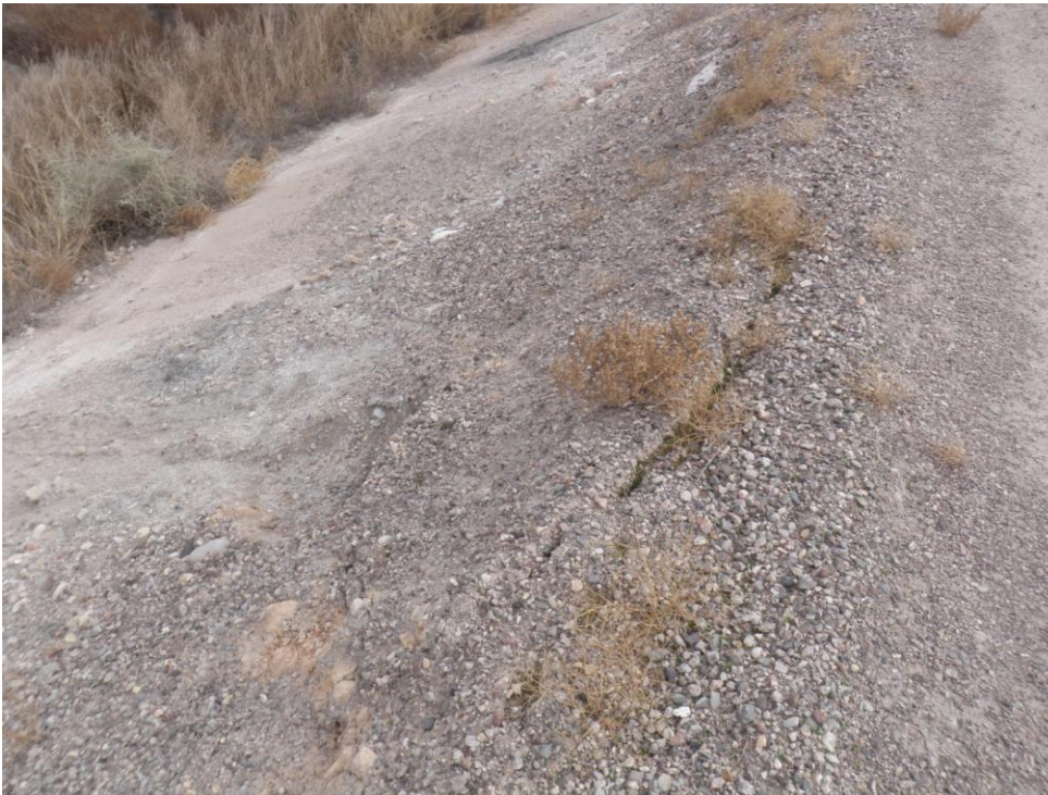
Photo 14: Pond F. Typical cracking and vegetation located along edge of crest and slope.
