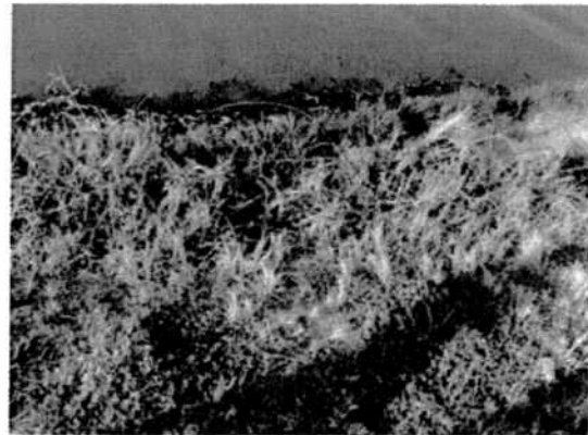
Figure 7: South Pond Upstream Embankment (Note geotextile well placed and functioning as intended)
