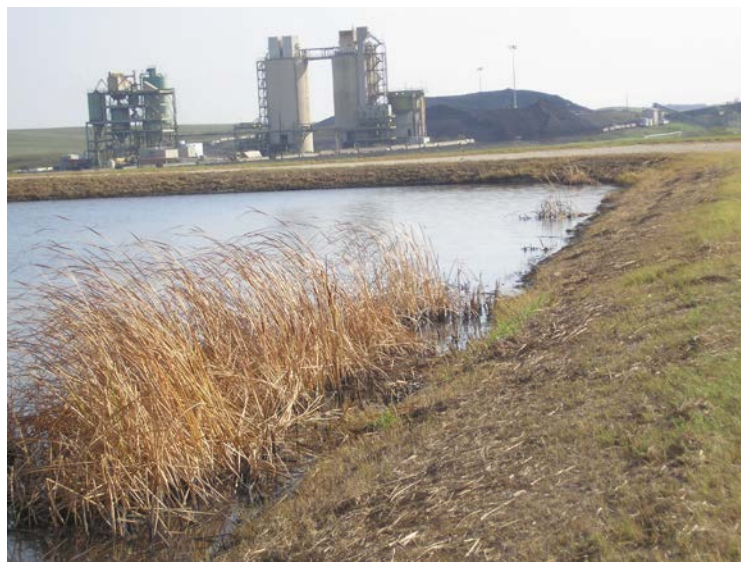
Figure 5.2.2-2 Area of Interior Slope Erosion – West Embankment
