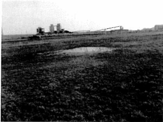
Figure 16: North Pond Standing Water at Toe
