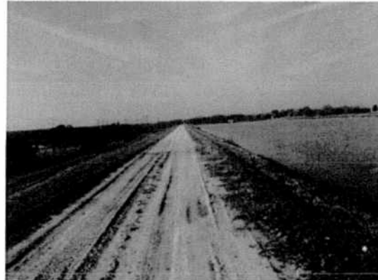
Figure 5: Crest Rutting South Pond
