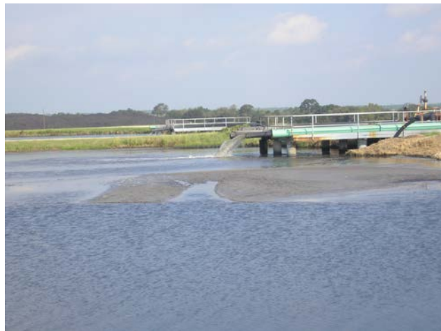
Photograph 2.2.2-1: Ash sluice water return pipes from dewatering bins to Bottom Ash Pond
