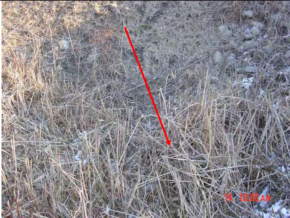
Photo #13: Culvert inlet clogged with vegetation, west side of south embankment, looking NE
