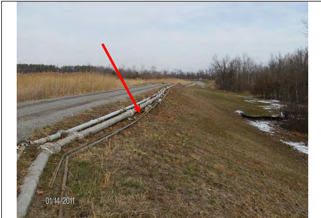
Photo #4: South embankment, exterior slope, looking east Note: Low spot in crest
