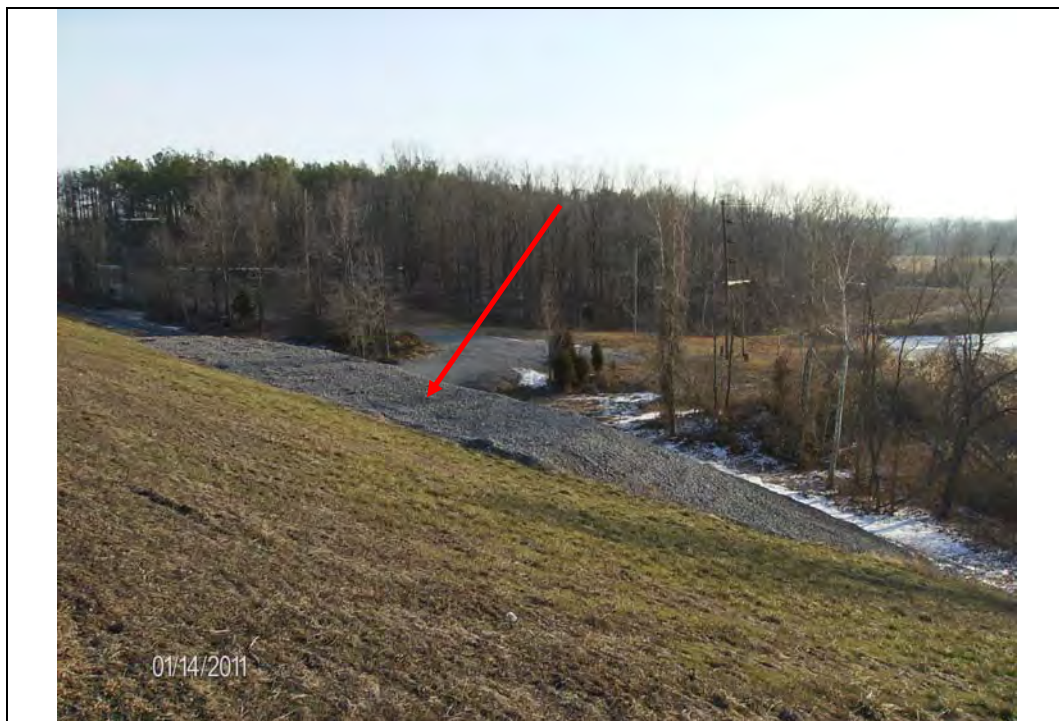
Photo #8: East end of south embankment, exterior slope, looking east Note: Rock toe berm
