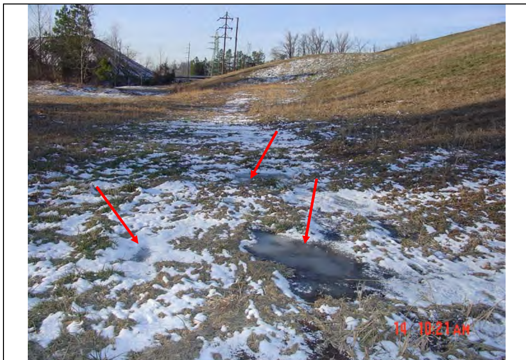
Photo #4: South embankment toe, looking SW Note: Ponded water along exterior slope toe
