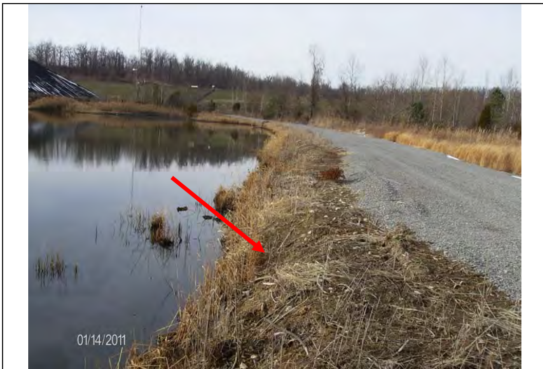
Photo #6: East embankment, interior slope, looking north Note: Animal burrows
