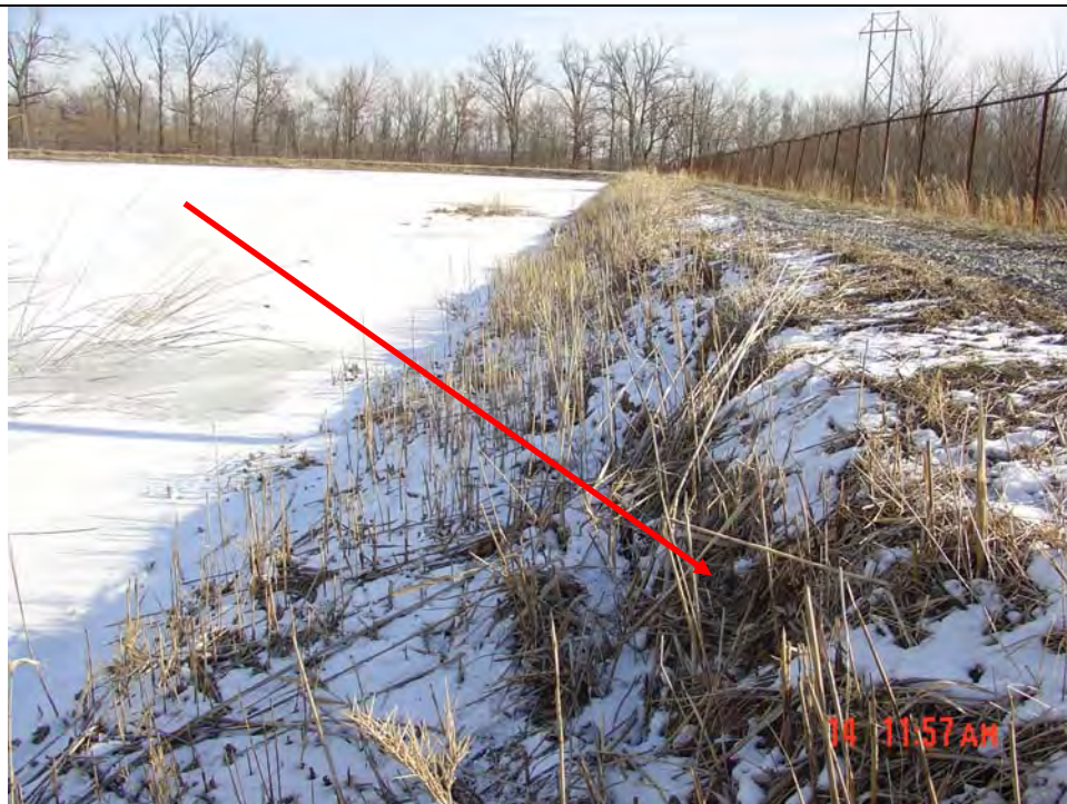
Photo #2: Interior slope of south embankment, looking east Note: Note wave erosion encroaching on edge of dam crest
