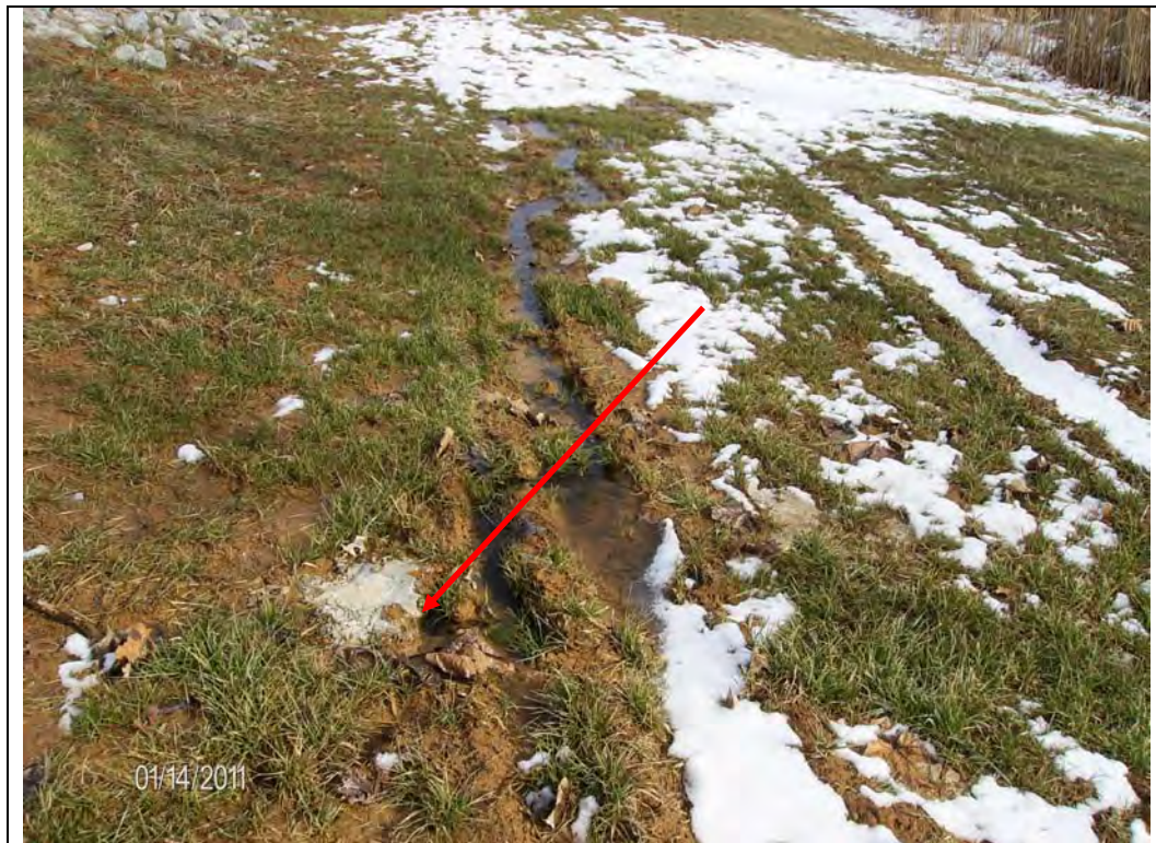
Photo #2: Seep at toe of south embankment, looking east Note: Source of flow adjacent to grouted hole
