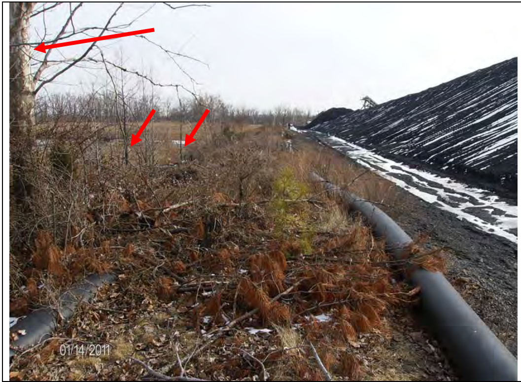
Photo #1: West embankment at NW corner, looking south Note: Sparse vegetation and trees along interior of embankment
