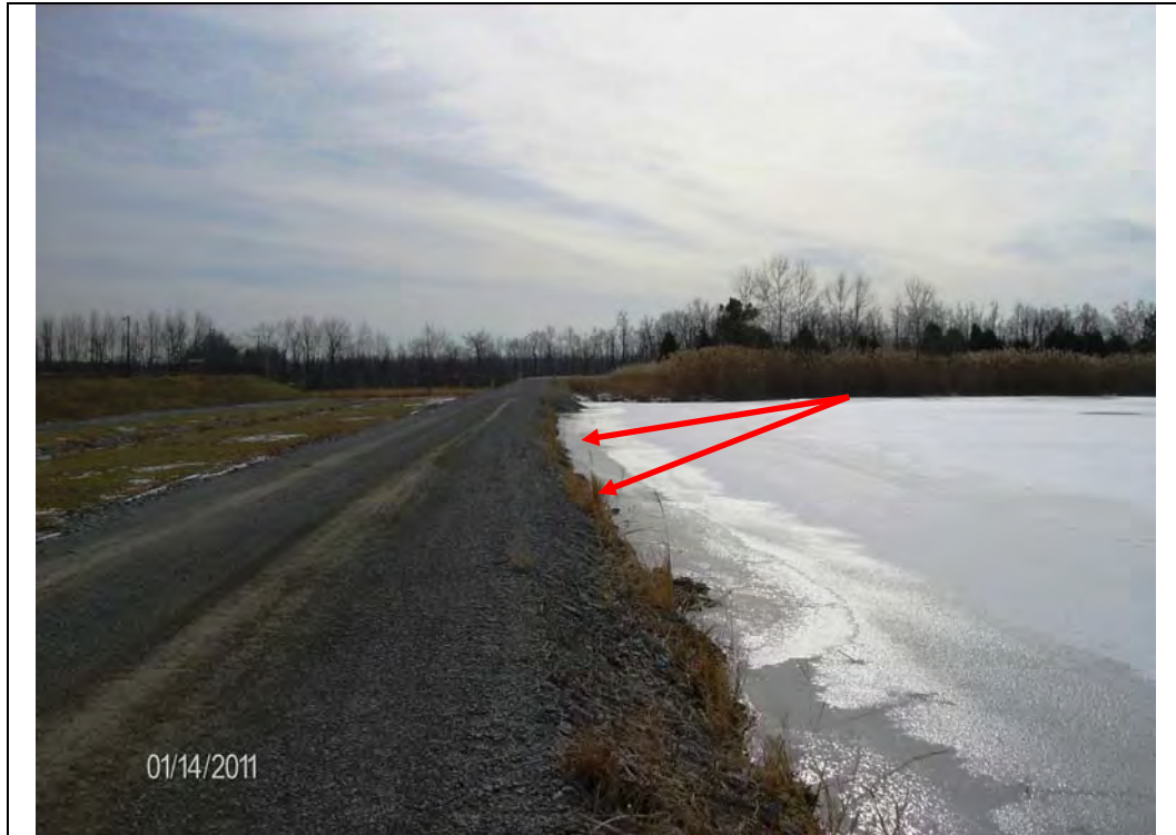
Photo #1: East embankment crest and upstream slope, looking south Note: steep slopes with sparse rip rap erosion protection.
