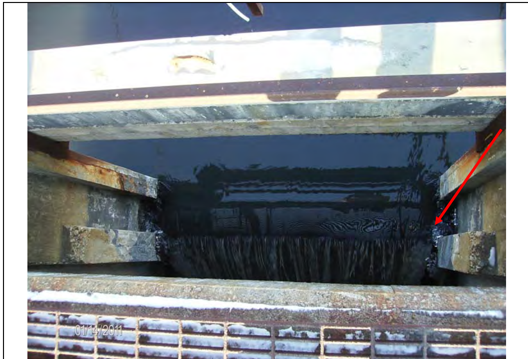
Photo #7: Principal Spillway inlet Note: Top of stop logs just below water surface
