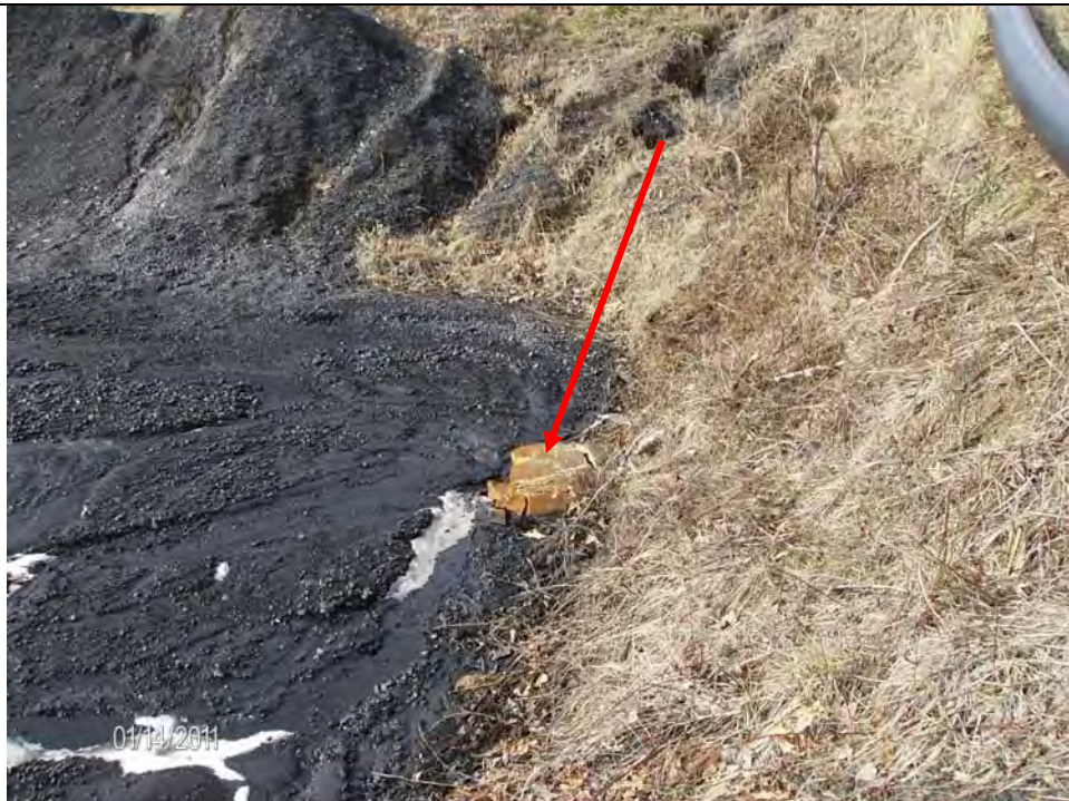
Photo #14: Repair concrete culvert inlet at toe near west end of south embankment, looking NW
