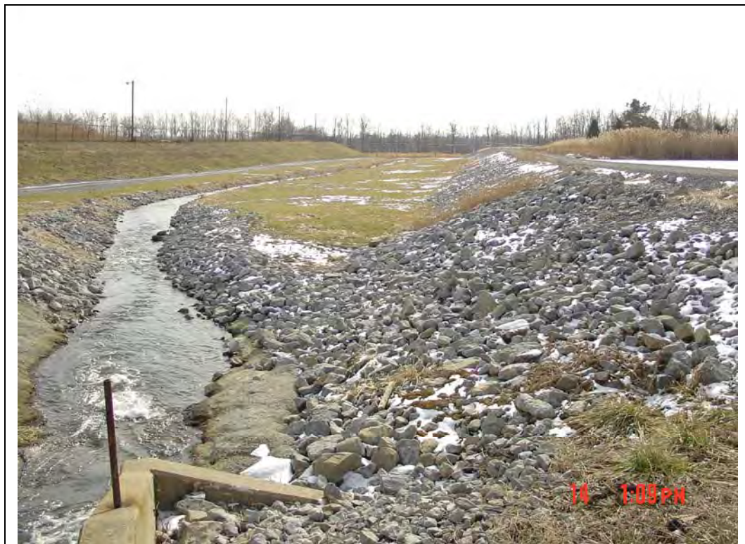
Photo #4: East embankment, downstream slope, toe, and principal spillway outlet, looking south
