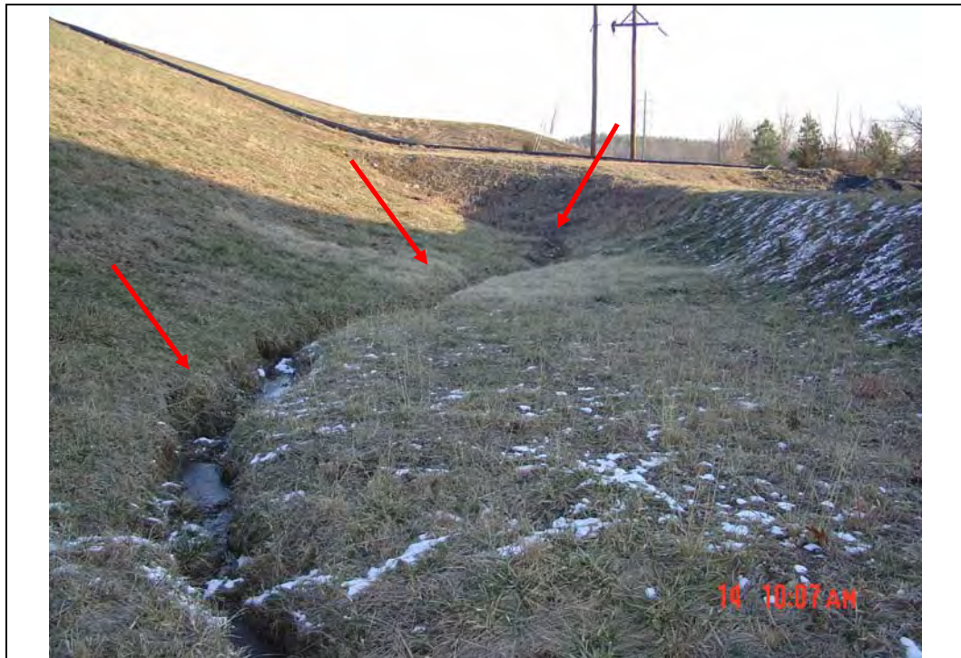
Photo #3: South embankment toe, exterior slope, looking NE Note: Groin ditch along toe, clogged culvert
