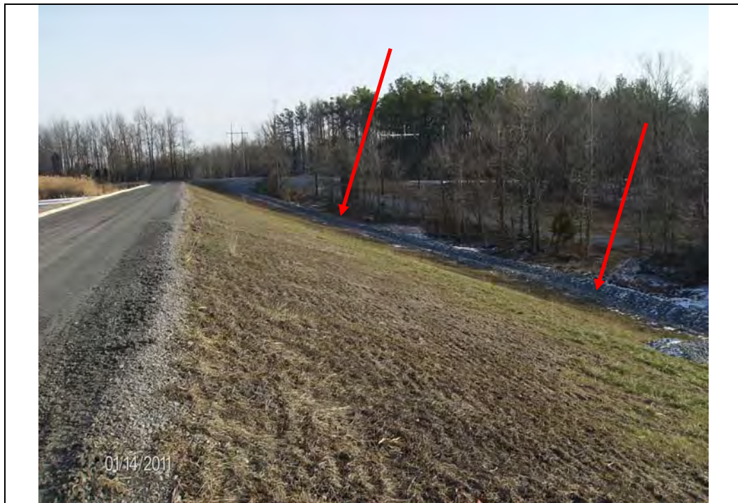
Photo #9: East end of south embankment, exterior slope, looking NE Note: Rock groin ditch recently installed along toe
