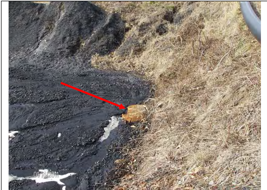
Photo #3: Inlet pipe from coal storage yard to coal runoff pond crushed, partially filled with coal, looking north
